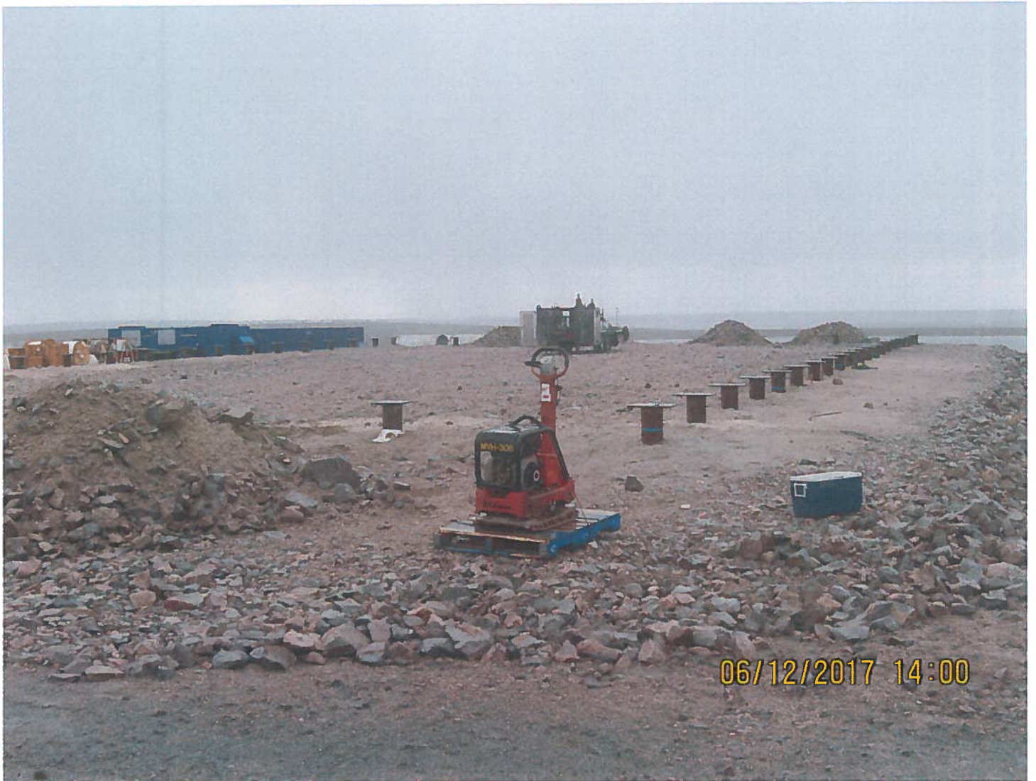
Photo 1: Sable Office Complex - Pilings have been installed for the new Chamco Building that will be installed this summer. The building will be used as a Maintenance building for equipment.
