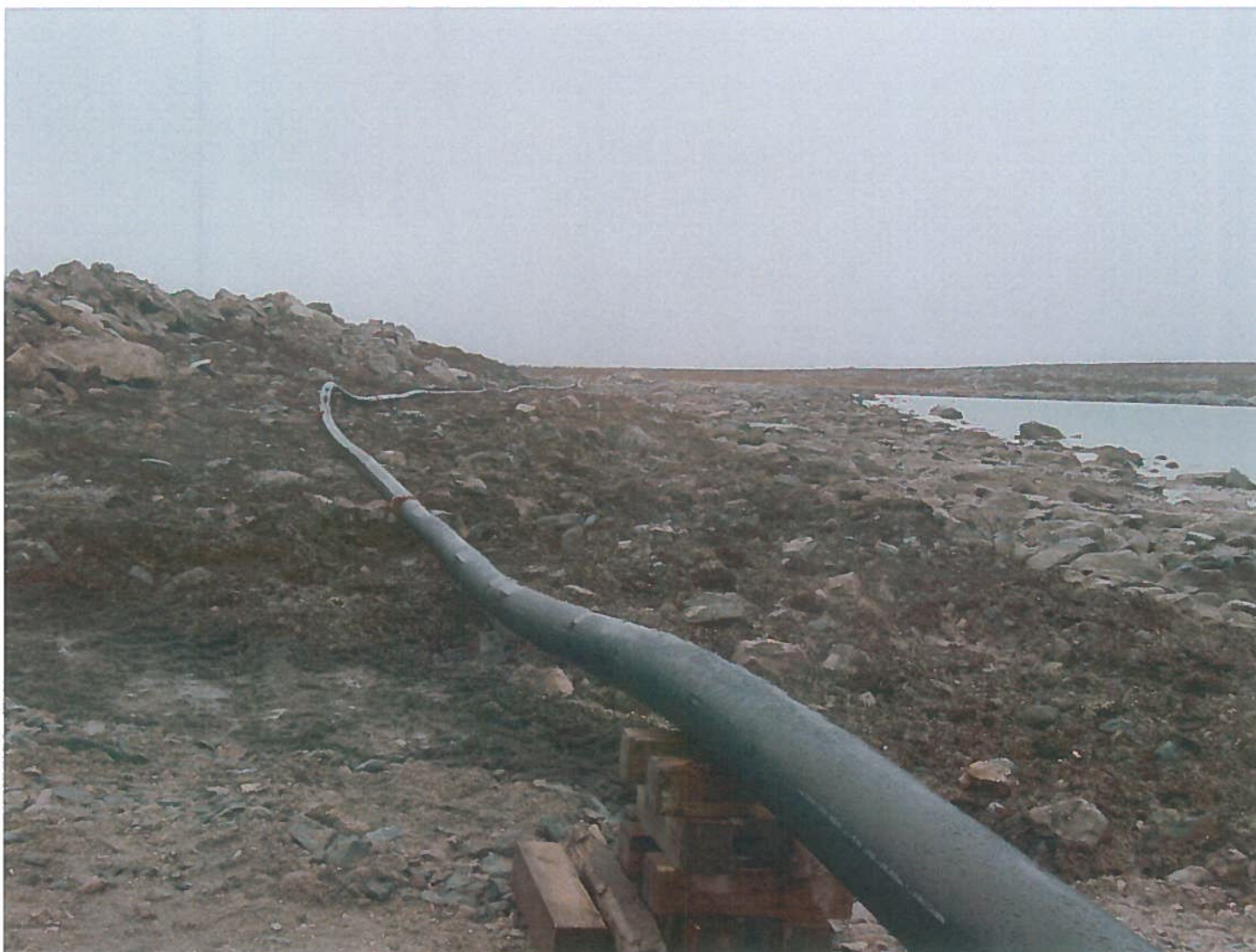
Photo 4: Sable Lake Dewatering Line- A 10" HDPE line was joined together in sections from Sable to Ulu Lake. The dewatering line is inspected daily for leaks by DDEC environment staff.
