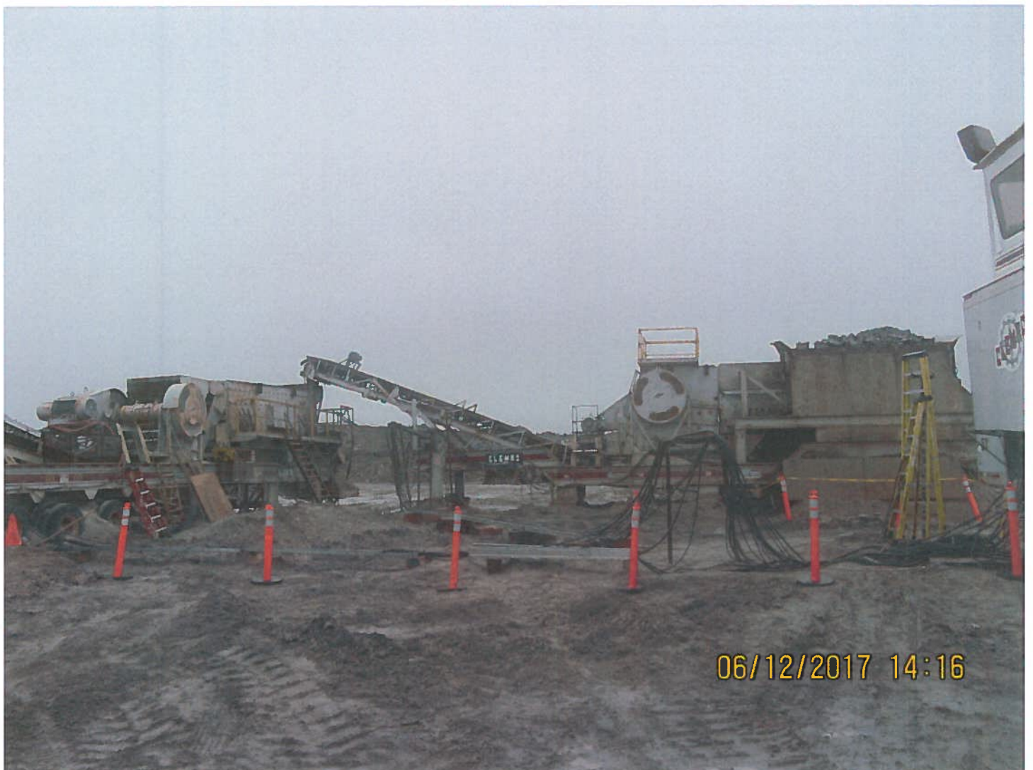
Photo 2: Sable Development - The Crusher at Sable started in the first week of June. Crushed rock of various sizes will be used for several projects at the Sable Development.
