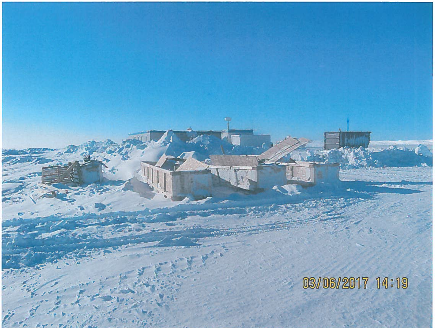
Photo 1: Sable Office Complex - Several crates and pallets were noted at the parking facility. The crates/pallets/scrap steel and wood debris will need to be disposed of to an approved facility
