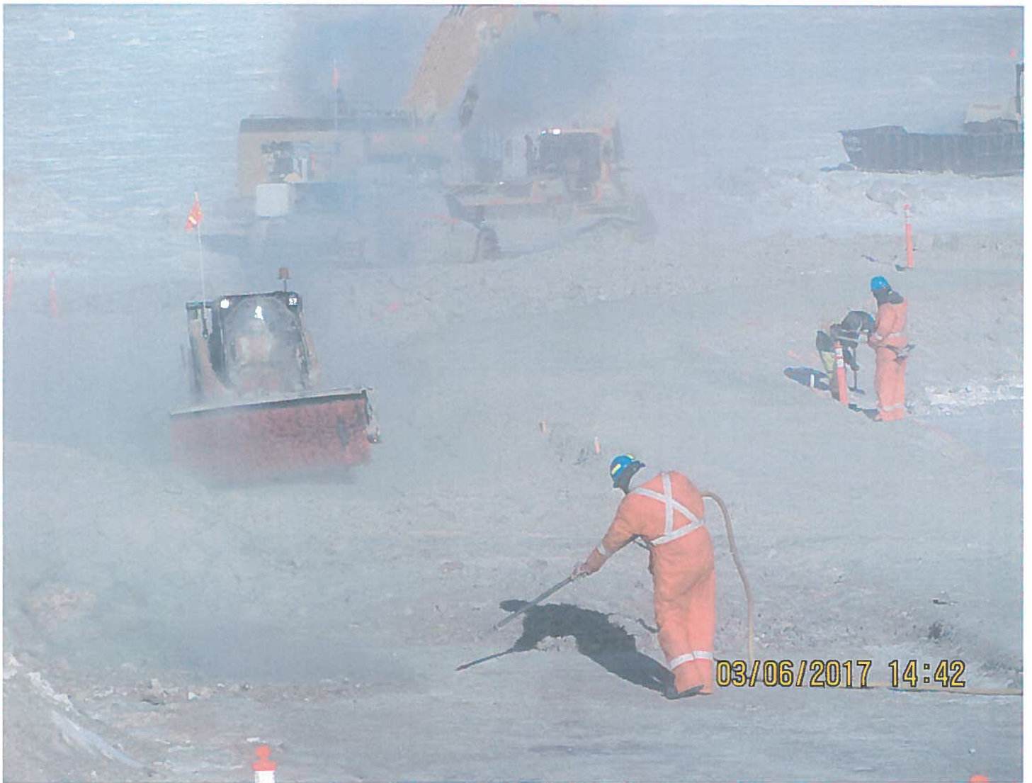
Photo 3: Two Rock Frozen Core Dam - Nuna staff are preparing the surface of the frozen core dam. The surface is being cleaned by a bobcat with a brush attachment and by compressed air. A clean surface is required to ensure the layers of slurry bond together.
