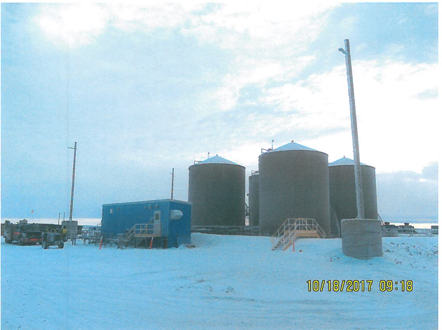
Photo 2: Sable Office Complex - Work with fuel piping and electrical continues within the 4 - 500,000 Litre fuel tank berm. The refuelling facility will be functional in the near future.
