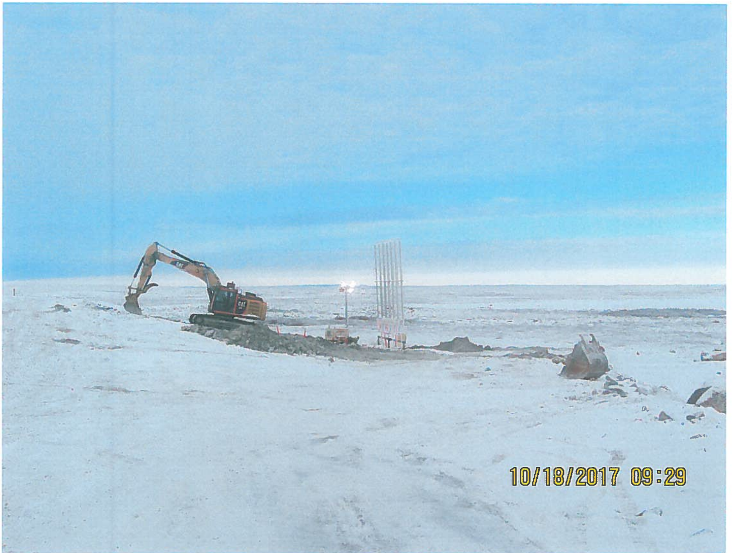
Photo 5: Frozen Core Dam - An excavator was observed working on the downstream side of the frozen core dam. Repair work was being conducted on a small section of the dam.
