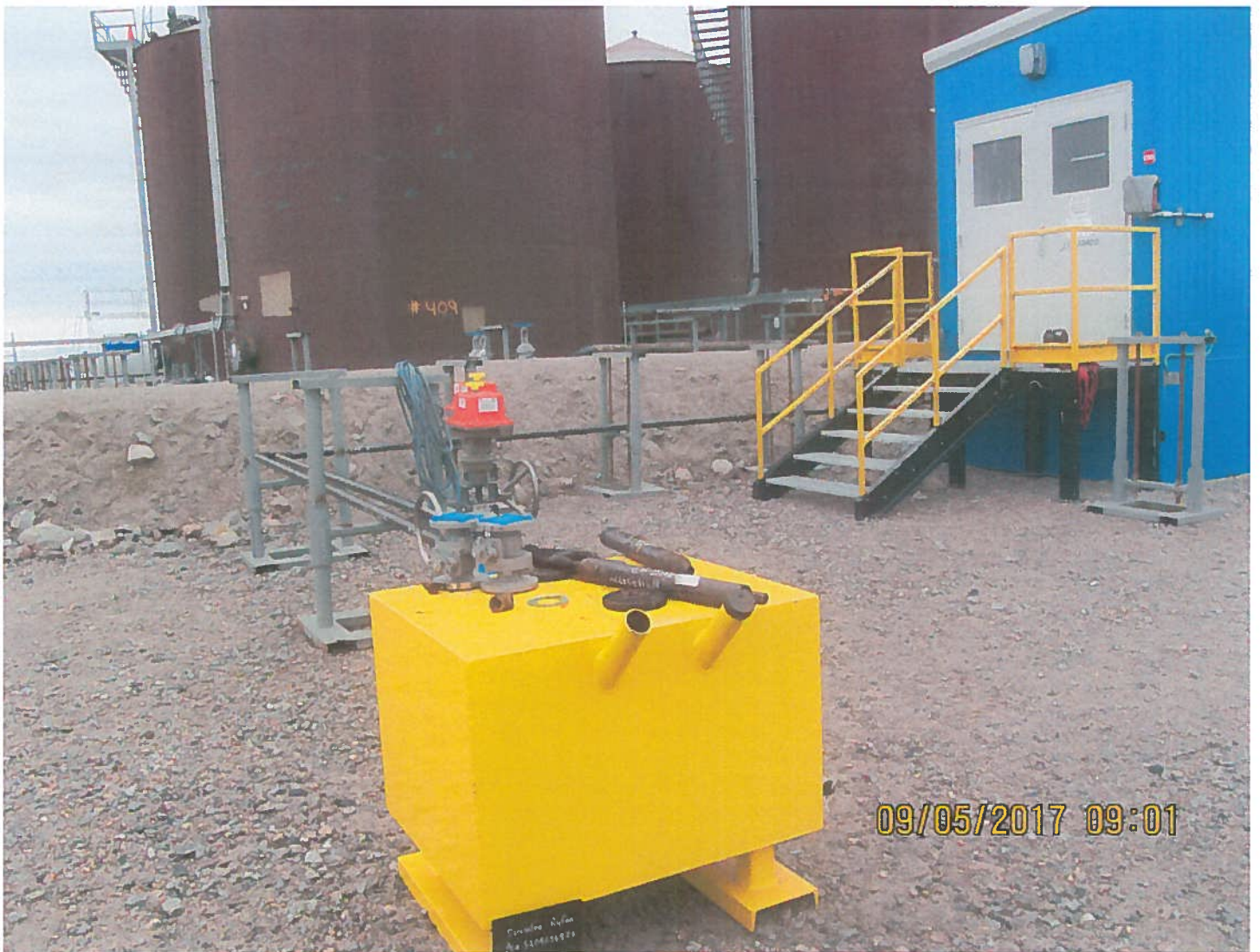
Photo 3: Sable Office Complex - A refueling nozzle cradle will be installed as part of the refuelling stations in the near future. The Inspector noted piping and fittings were in position for this unit.
