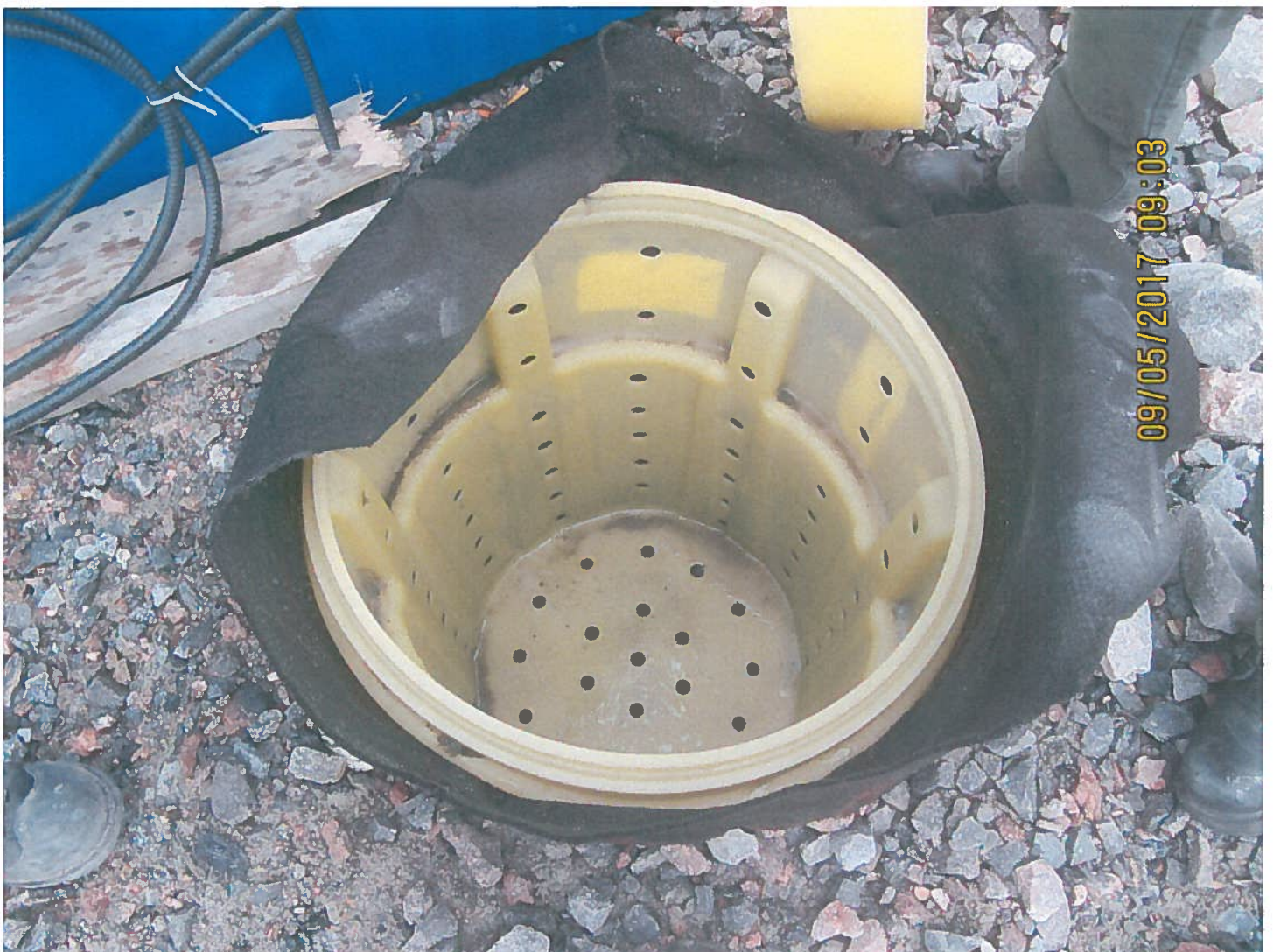
Photo 4: Sable Office Complex - A Berm pump out sump was installed to assist in the removal water from this facility.
