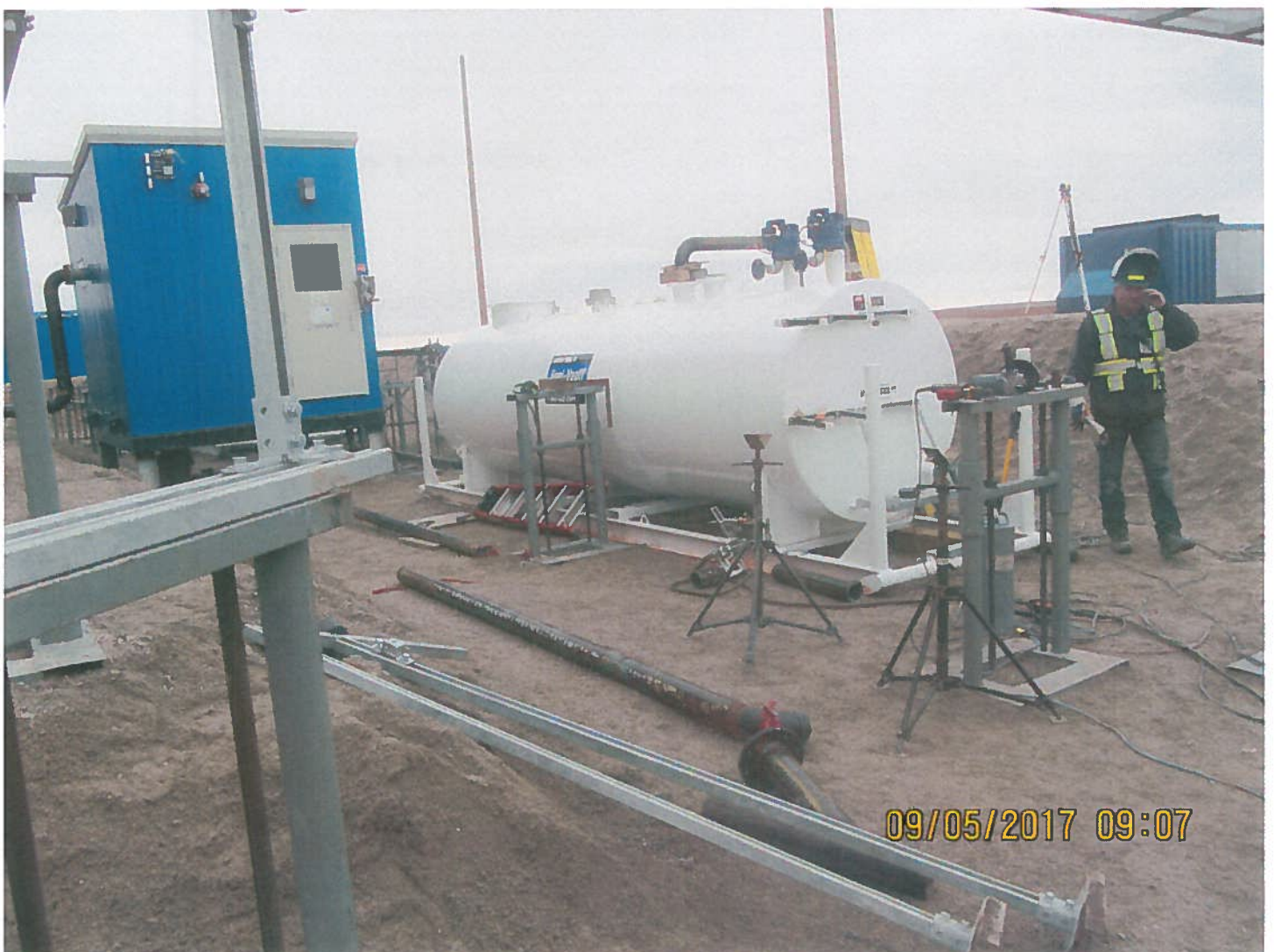
Photo 2: Sable Office Complex - Work with fuel piping and electrical continues within the 4 - 500,000 Litre fuel tank berm
