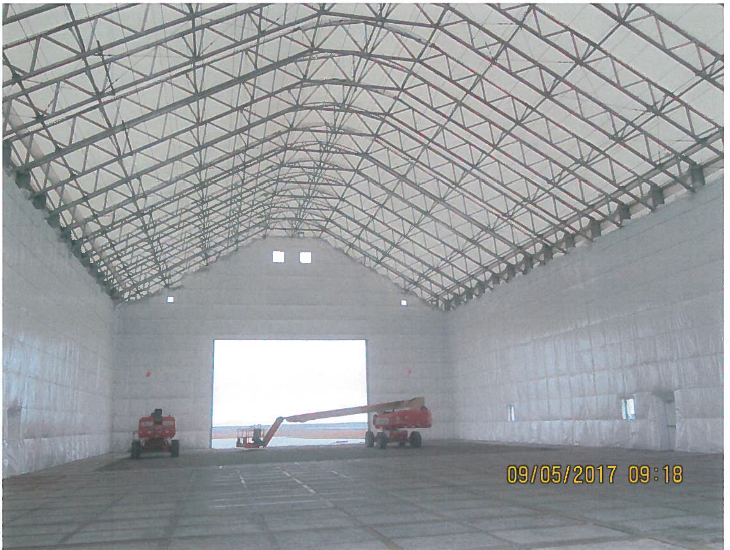
Photo 1: Sable Office Complex - The Frame of the maintenance shelter has now been completed. All 4 walls and the roof of this building have now been covered
