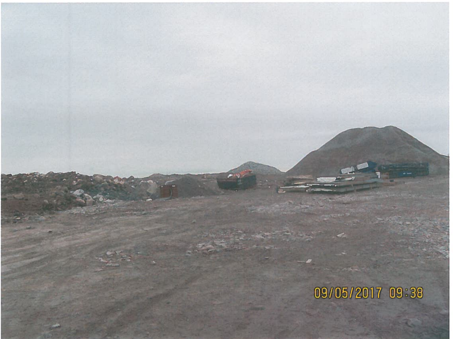
Photo 8: Sable Frozen Core Building Laydown Area - The Laydown for this facility was cleaned up shortly after this inspection.
