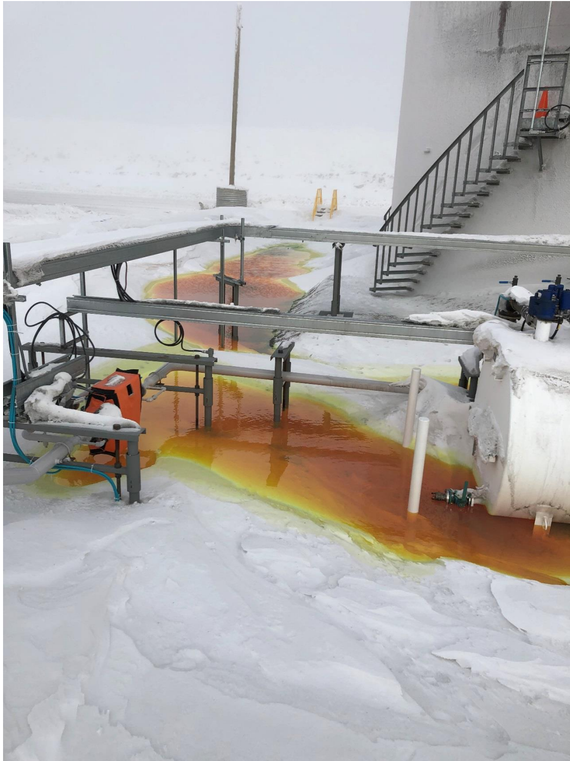
Figure 3. Pooled Diesel within Sable Fuel Tank Farm Containment Berm (March 21, 2019)
