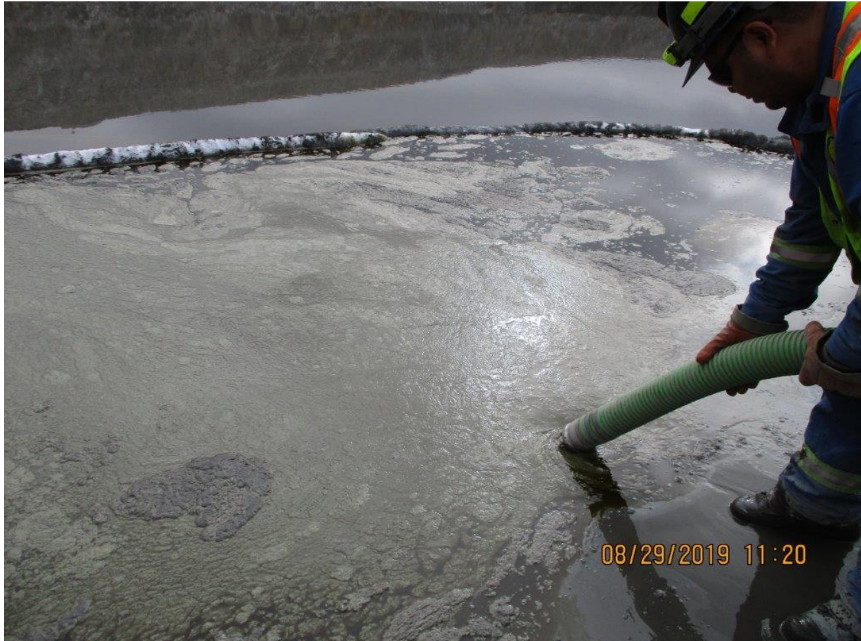
Figure 3. Vacuum truck used to recover hydraulic oil
