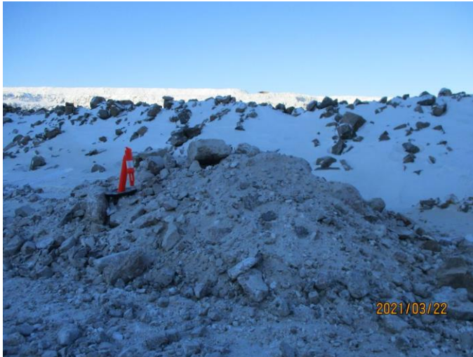
Figure 1. Spill 2021103 clean up in progress
