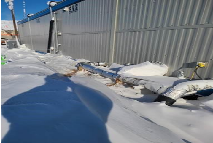
Photo 1: View of cracked pipe which resulted in the initial spill. Photo taken facing north on March 01, 2022.
