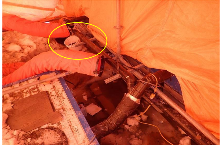
Photo 2: View of bucket placed under the pipe (to capture sewage) while it was repaired. Photo taken on March 01, 2022.
