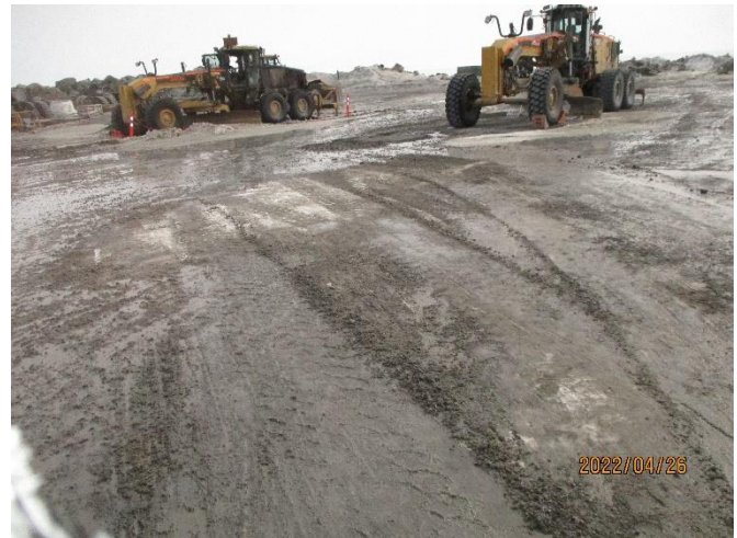
Photo 2: Sable Down Line – View of spill area after clean-up occurred.
