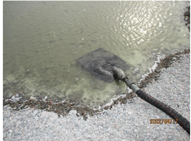
Photo 2: Sable Truck Park Area – View of sucker pump removing fuel from berm area shown in photo 1.
