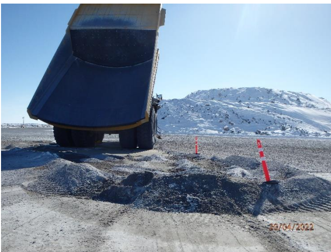
Photo 3: Sable Truck Park Area – View of crush placed down after the fuel was sucked up. The crush absorbed hydrocarbons.
