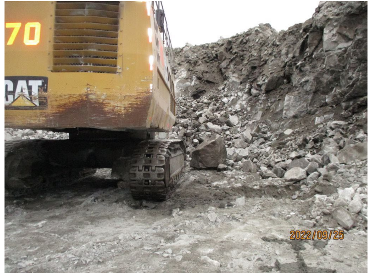
Photo 2: Sable Pit – Spill area next to shovel after the fuel tank had been drained.
