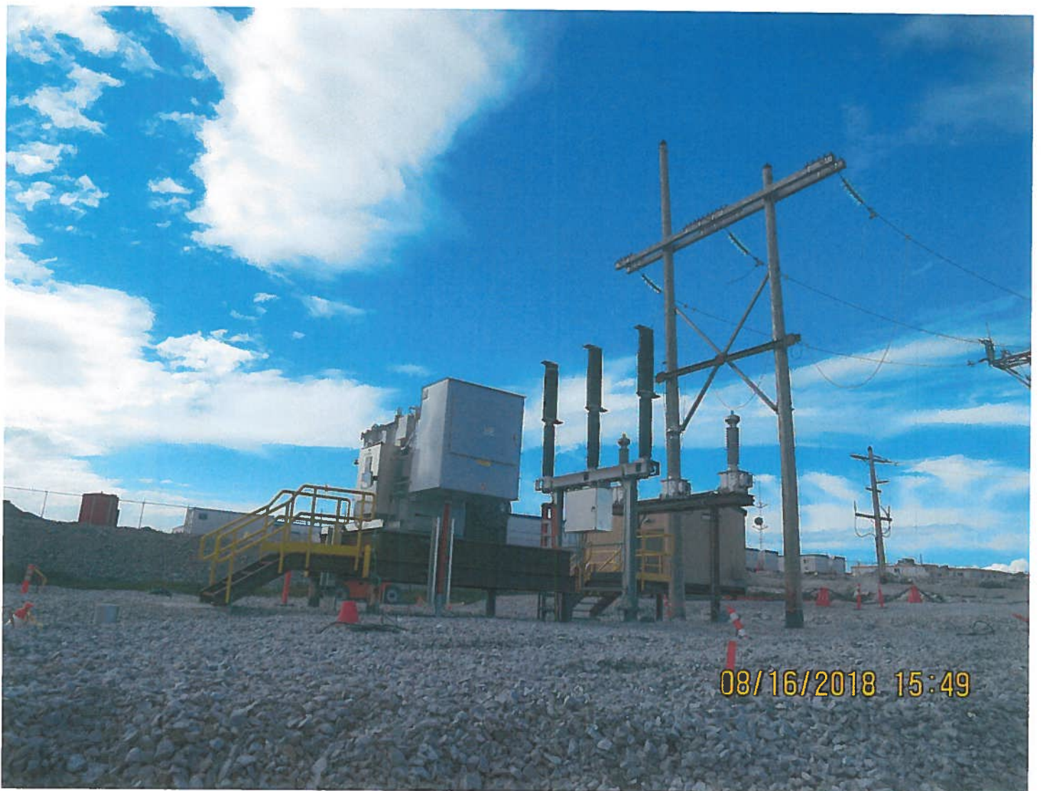
Photo 5: East of Misery camp - A 15 kv transformer located on the east side of Misery camp will be used to provide power to the Misery underground mining project.
