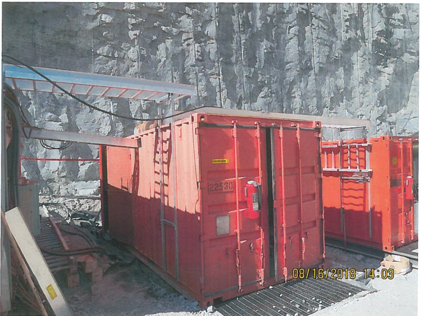
Photo 4: Misery Pit 2235 Level - Four generators have been placed in sea cans on the 2235 bench to provide power for the portal work.
