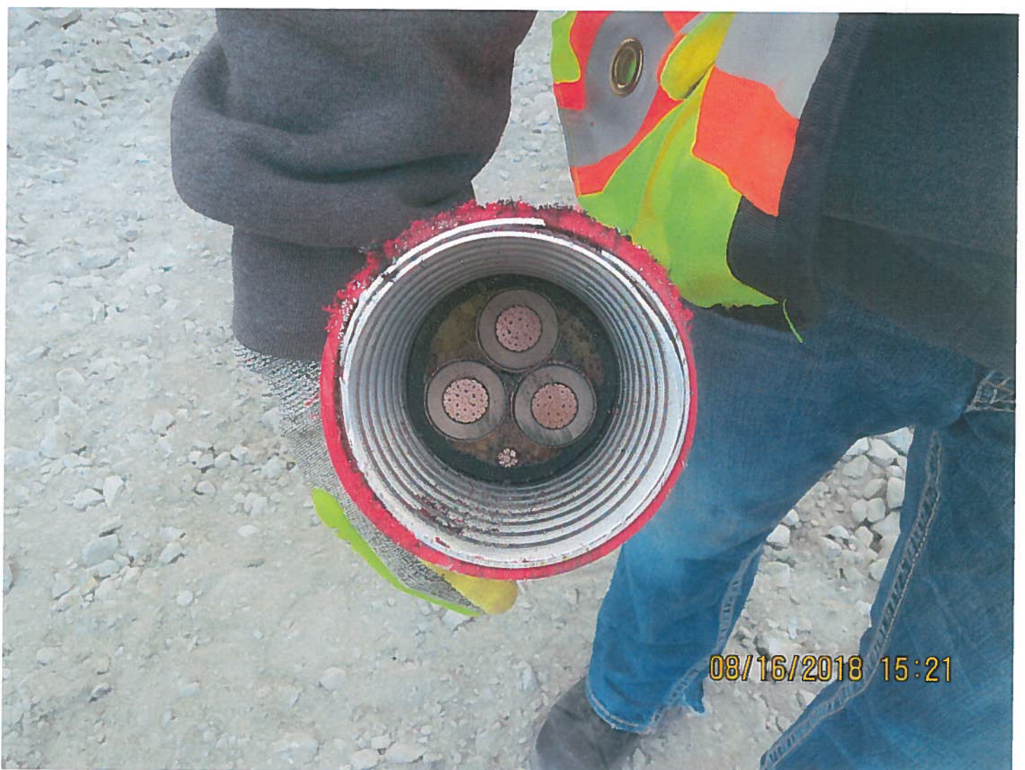
Photo 6: Misery FAR raise 440 bench - Insulated tech cable will transfer power from a transformer located east side of Misery camp to another transformer near the Fresh Air Raise ( FAR ) .
