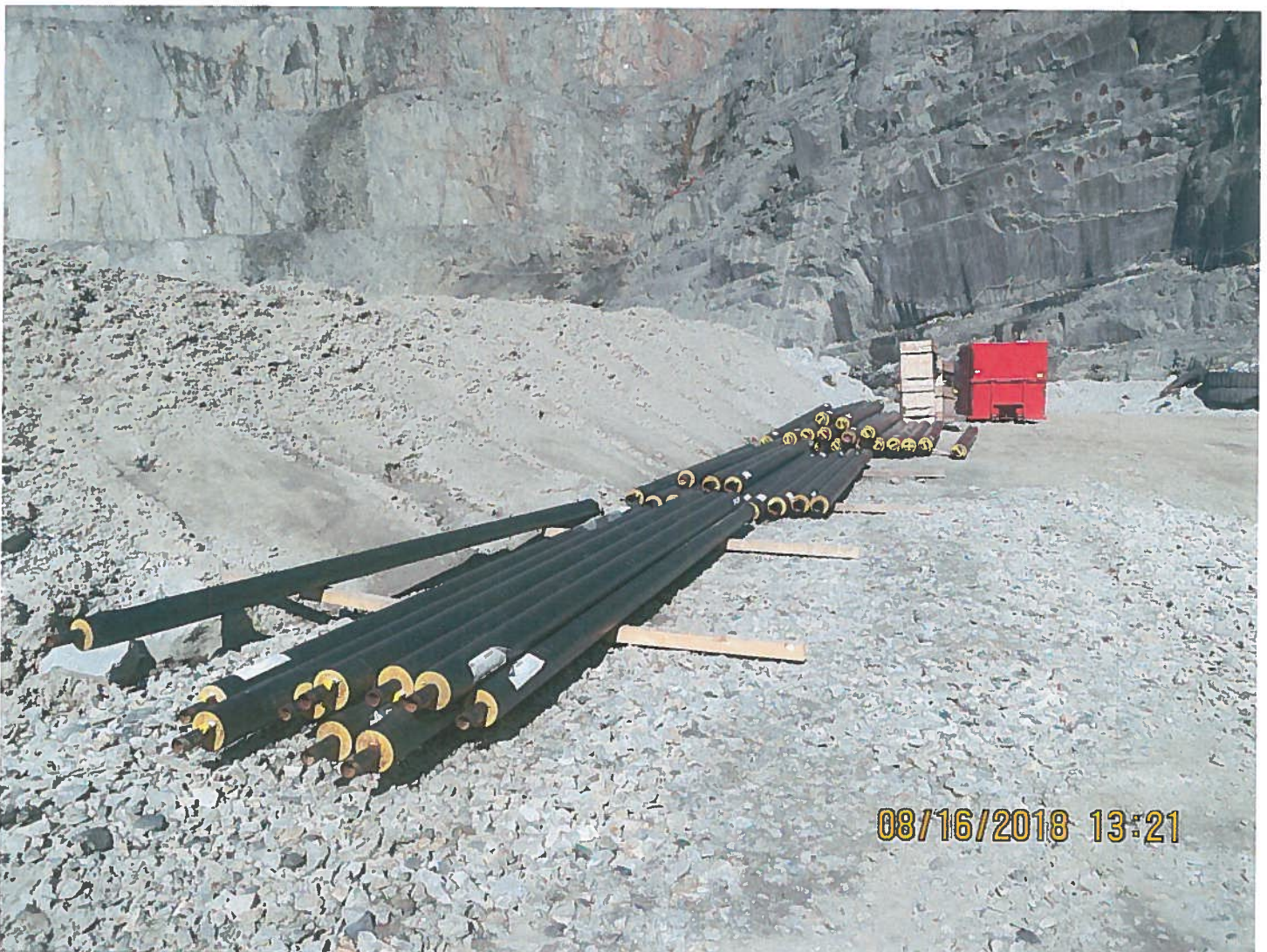
Photo 18: First Switch Back - Additional supplies are being stored on the first switch back in the Misery Pit. Air, water and discharge lines are currently stored at this location.
