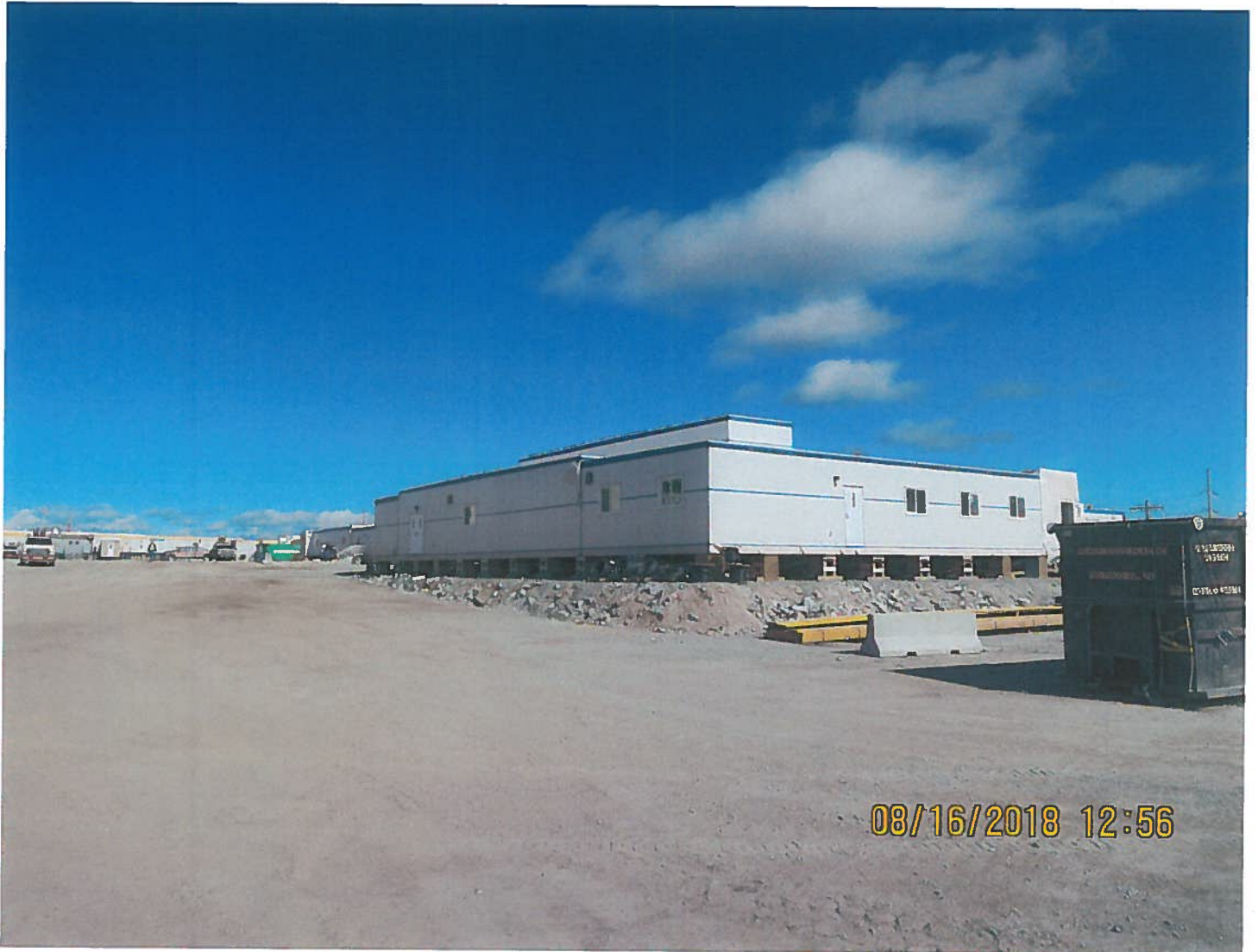
Photo 1: Misery Camp expansion - Accommodation expansion is currently underway at the Misery Camp. The additional prefabbed buildings have been attached to the older camp
