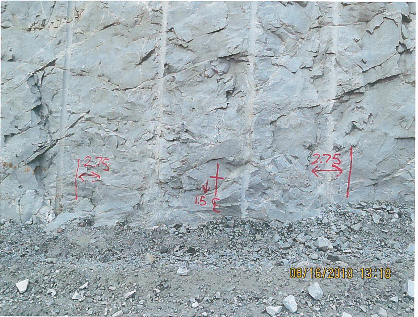
Photo 17: Level 2350 - An additional portal has been marked out on the Misery ramp road. This portal will be established in the future at around the 2350 bench mark.
