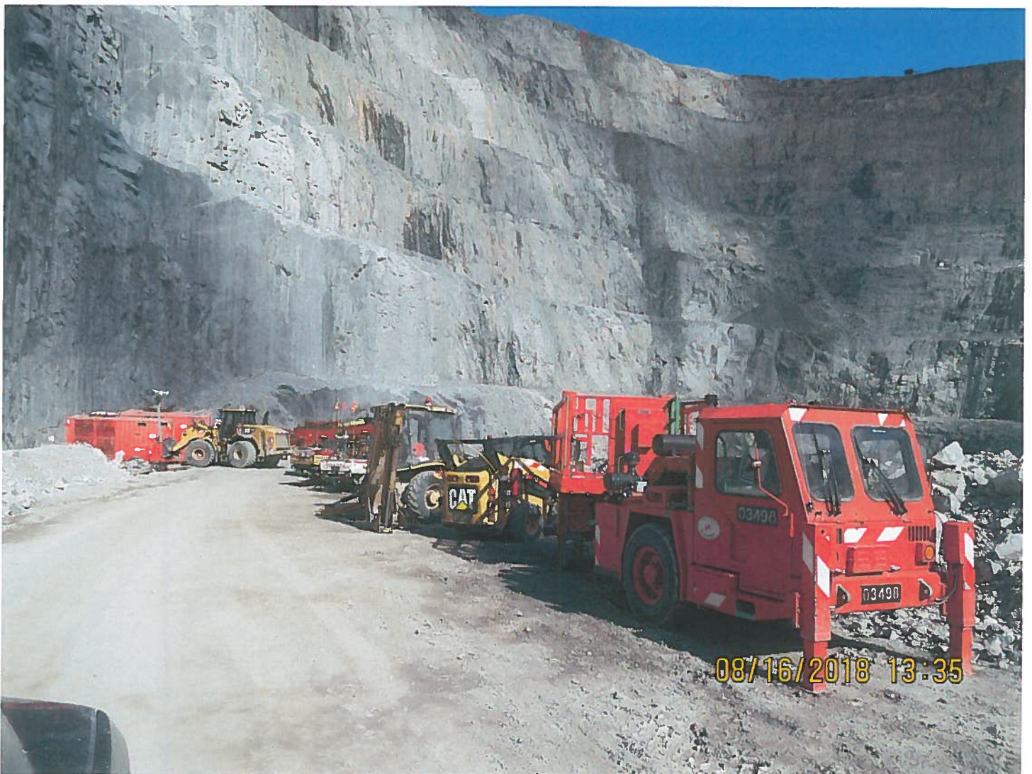
Photo 10: 2235 Portal - Equipment staged to the south of the 2235 portal. A catch berm is being constructed next to the pit walls to catch falling rocks.
