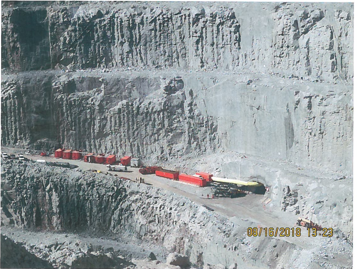
Photo 9: 2235 Portal - View of the 2235 portal from the first switch back on the east side of the Misery Pit.
