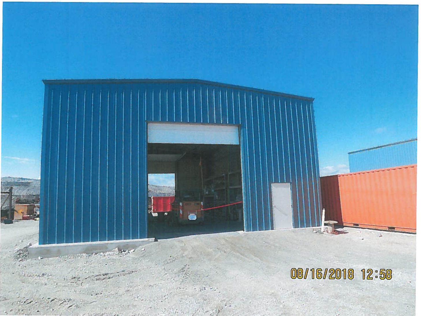
Photo 2: Misery Camp- Cold storage - A cold storage building is being constructed to house consumables for the underground project. ProCon will be storing parts and equipment within the building.
