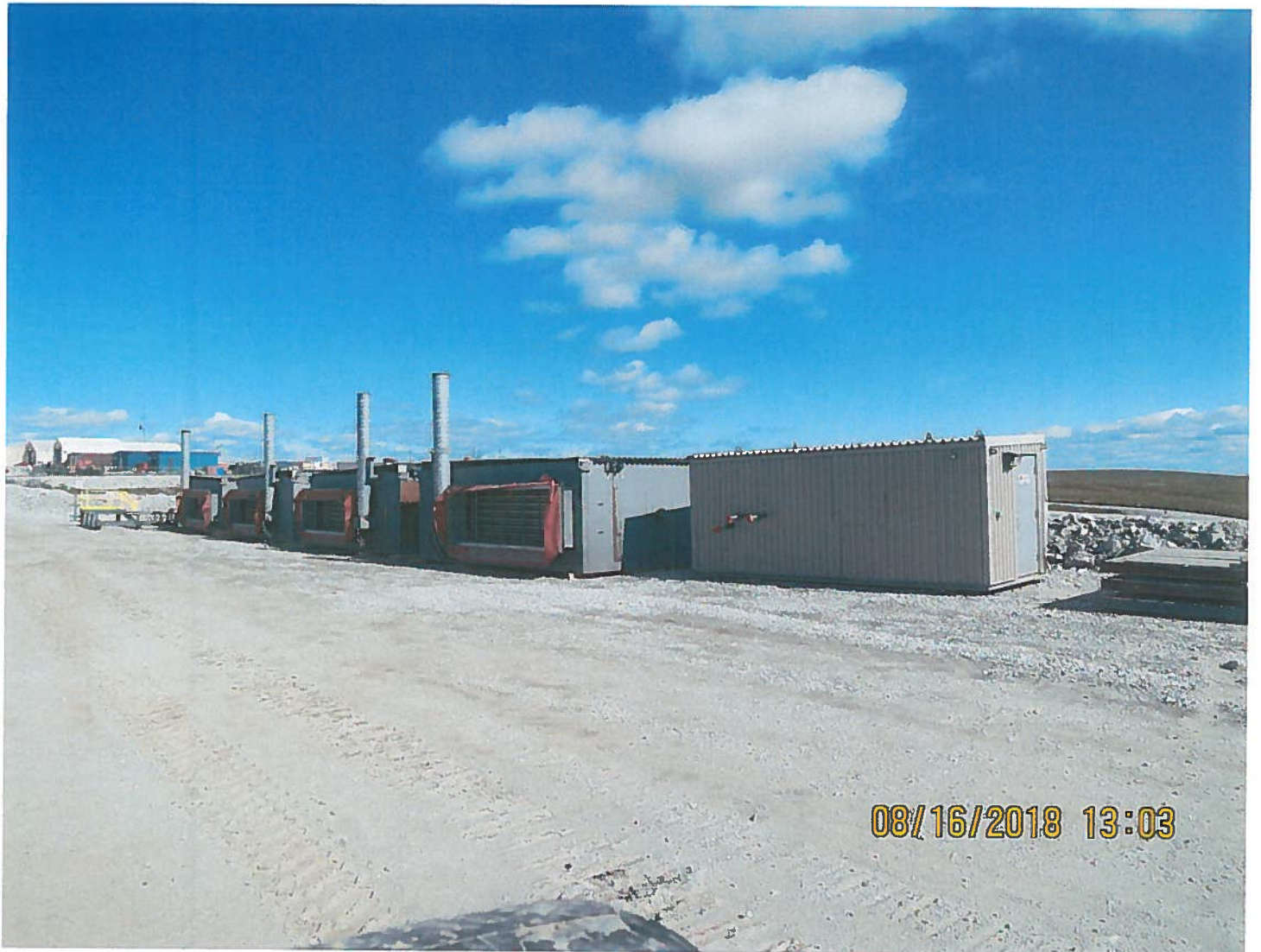
Photo 19: Misery Pit Laydown - Four air heaters that were used in the koala underground will be repurposed and installed at the 440 Bench on the Fresh Air Raise ( FAR) .
