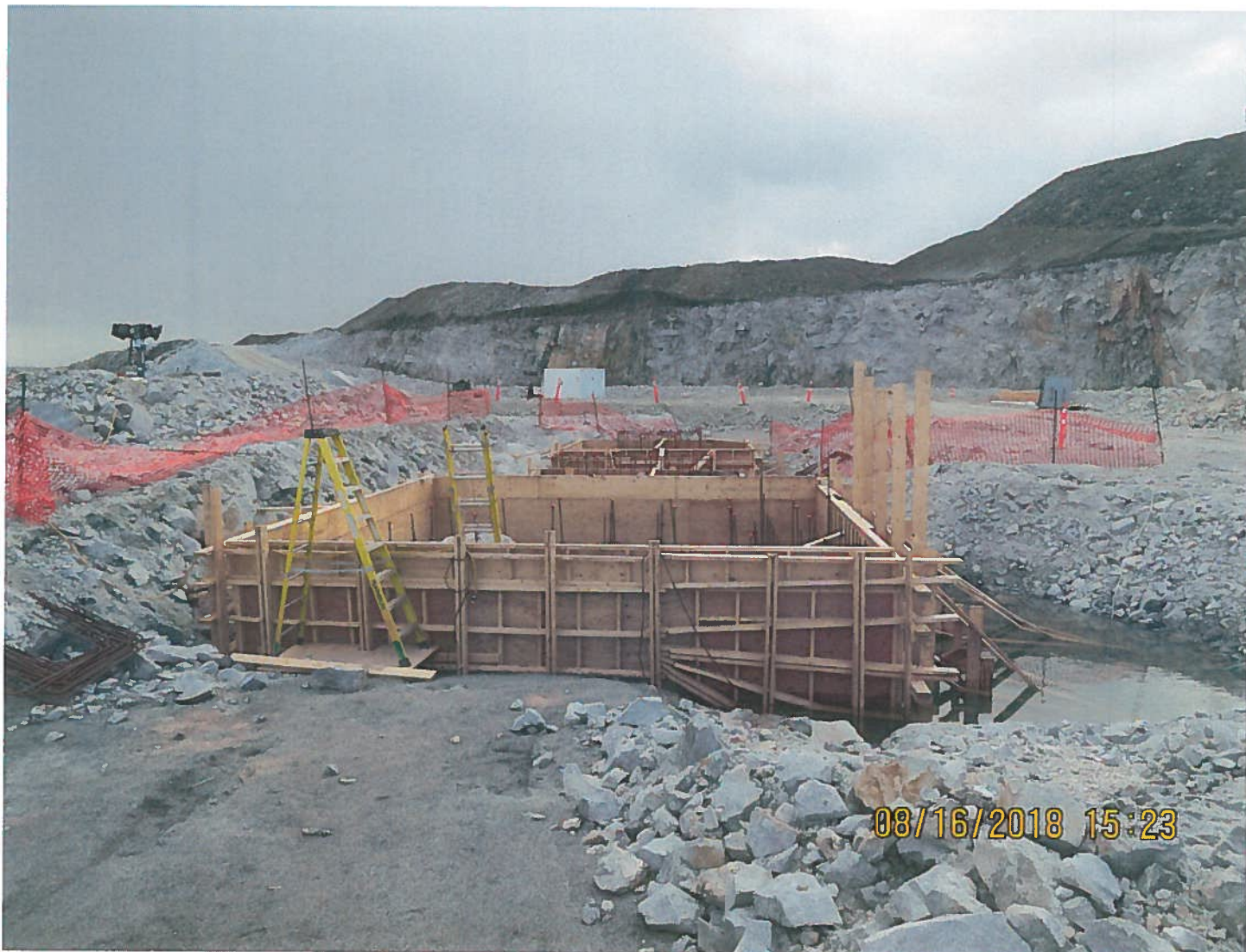
Photo 7: Fresh Air Raise - The fresh air raise foundation and supporting infrastructure foundation were being prepared for concrete pouring at the 440 Bench.
