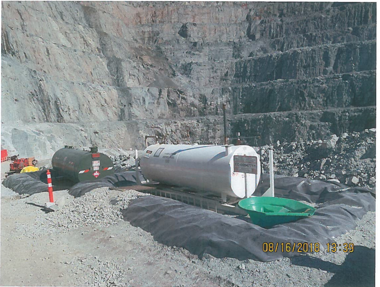
Photo 15: 2235 Portal - Two double walled fuel tanks ( 13,200L and 4530L) have been placed in a lined berm and are used to fuel the generators.
