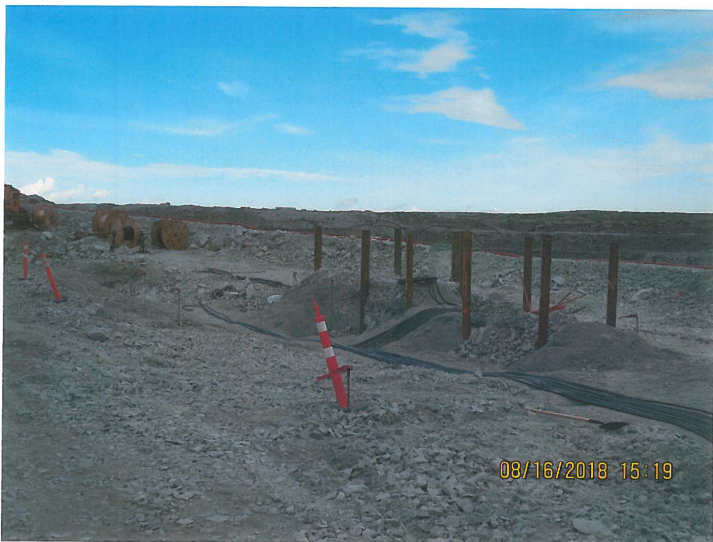
Photo 8: Fresh Air Raise 440 bench - The transformer that will supply power to the FAR was also under construction. Steel pilings and electrical cables were in position for the transformer platform.
