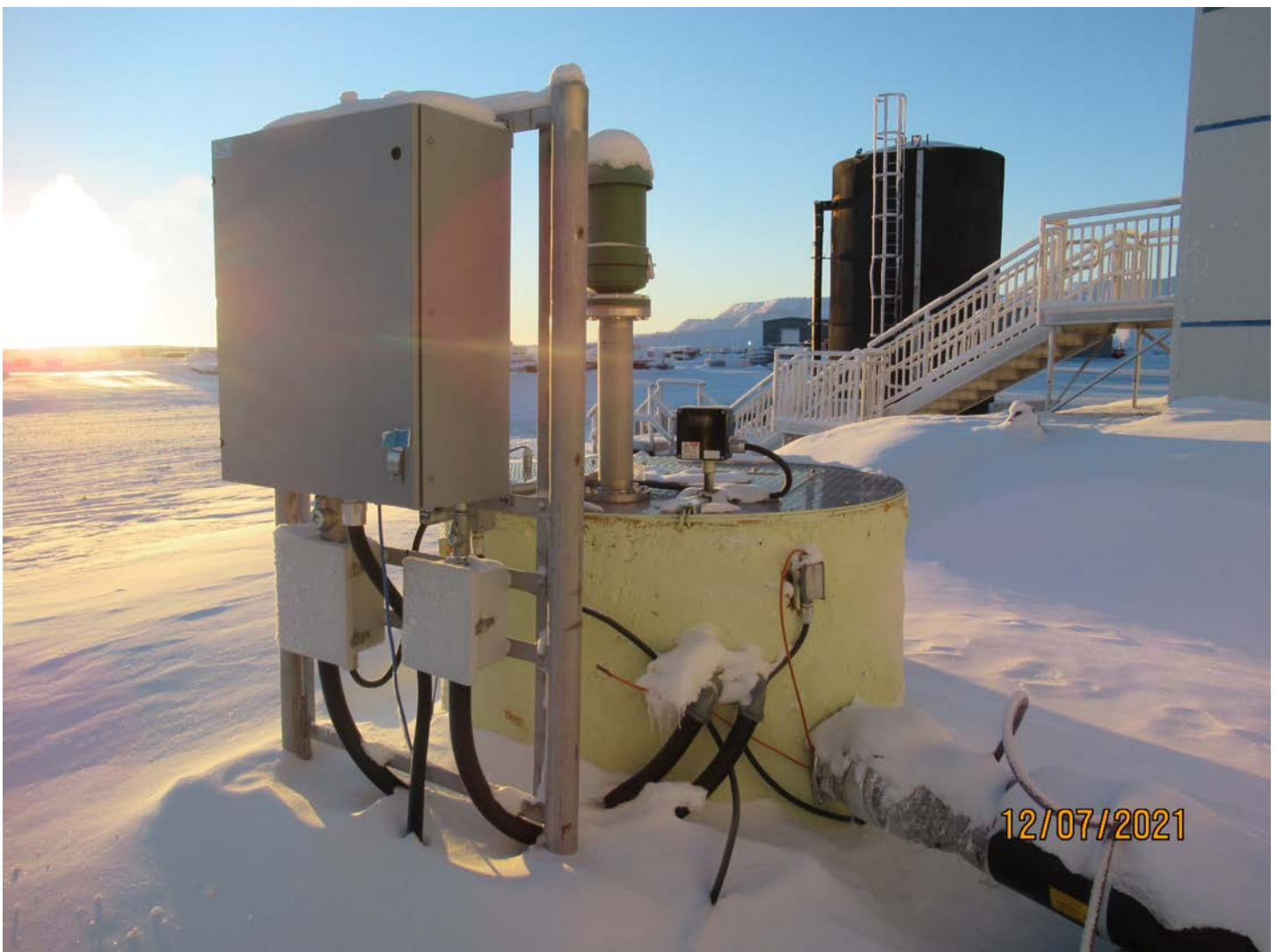
Photo 38: The sewage lift station located east of the sewage holding tank outside the camp buildings.
