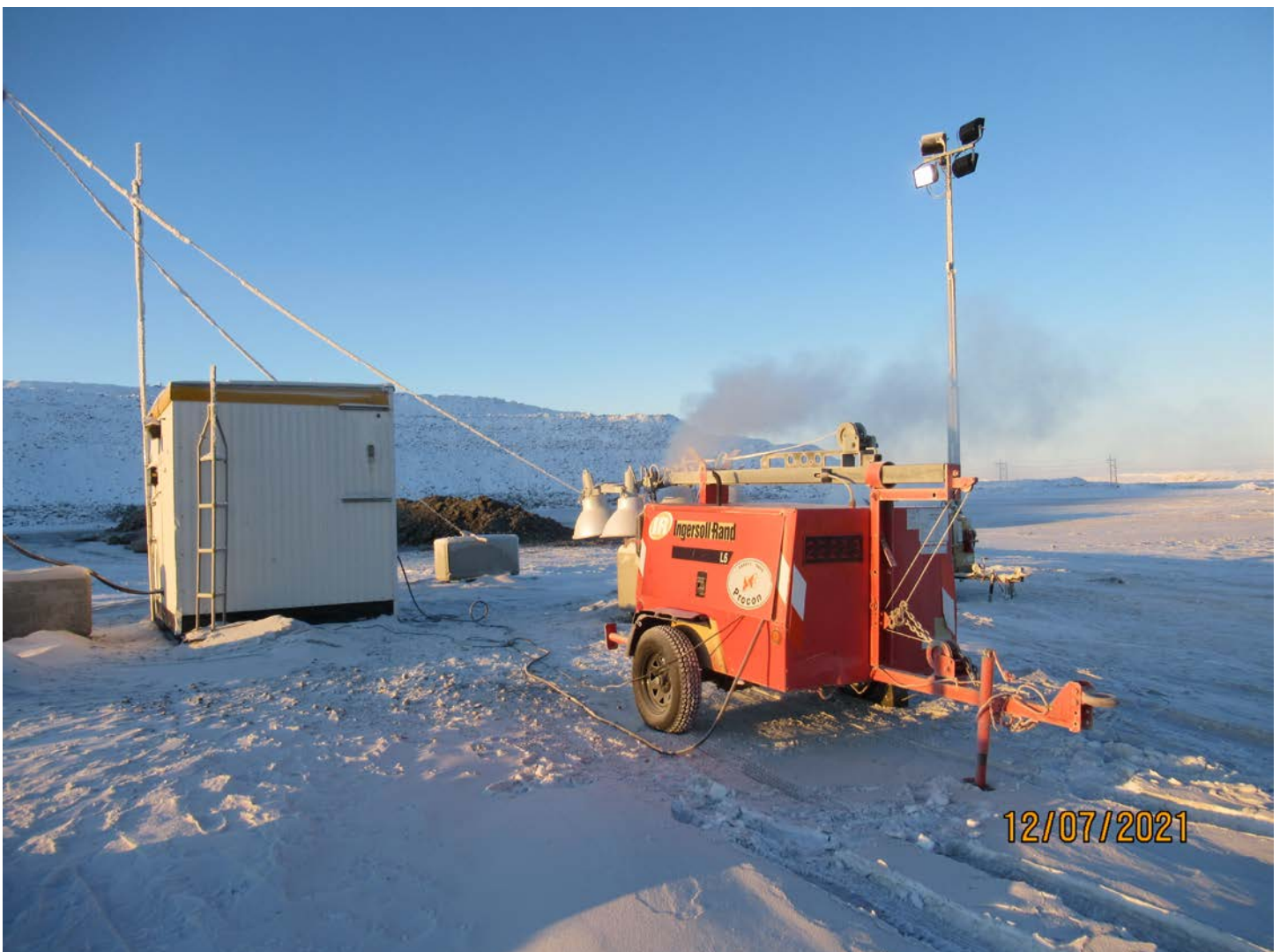
Photo 10: The light plants at the ore laydown also required secondary containment.
