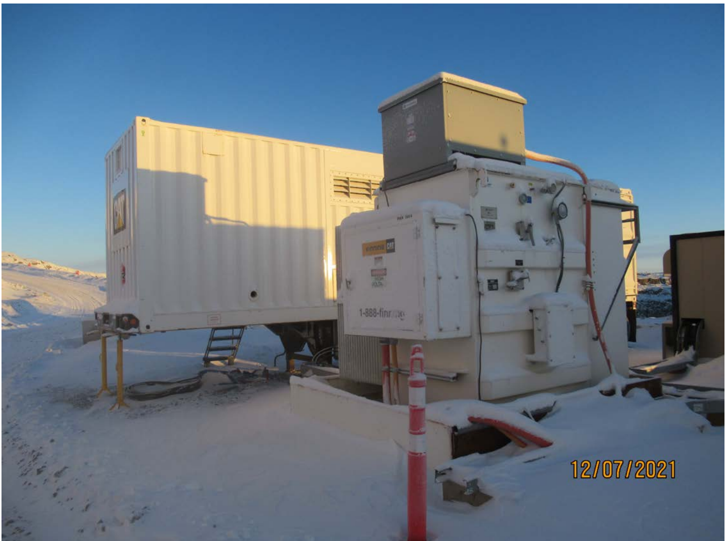
Photo 4: Generators staged on the Misery Pit 440 Bench.
