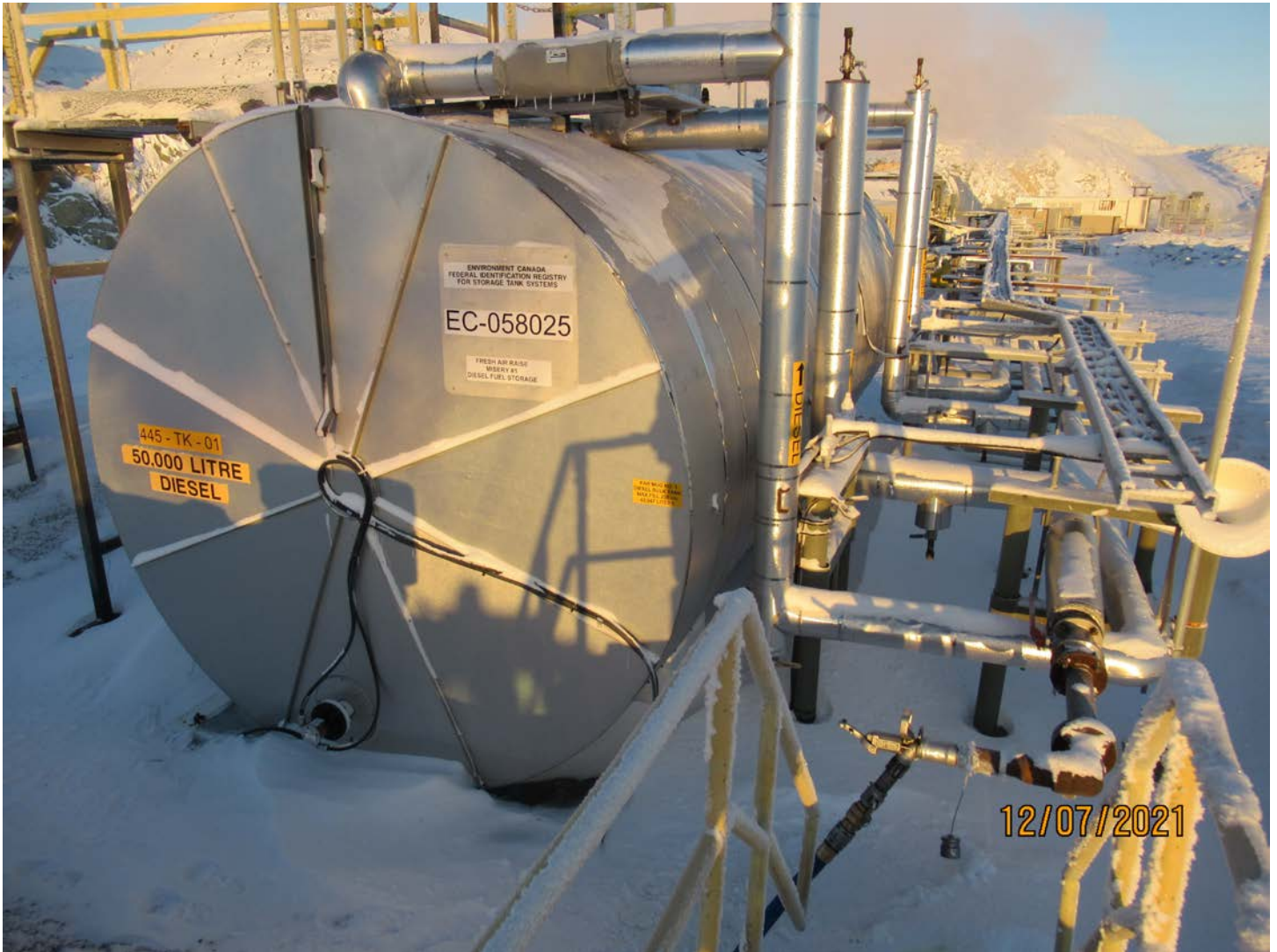
Photo 5: This 50,000 L diesel tank is used to supply the FAR station.
