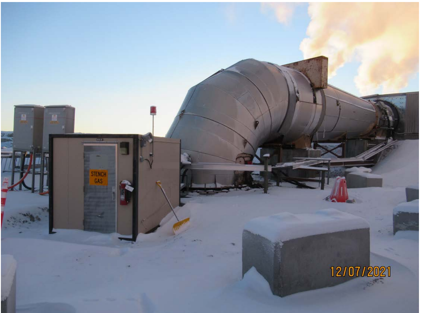
Photo 2: The FAR station pumps heated air into the underground. The electrical also runs through the borehole to the underground operations.
