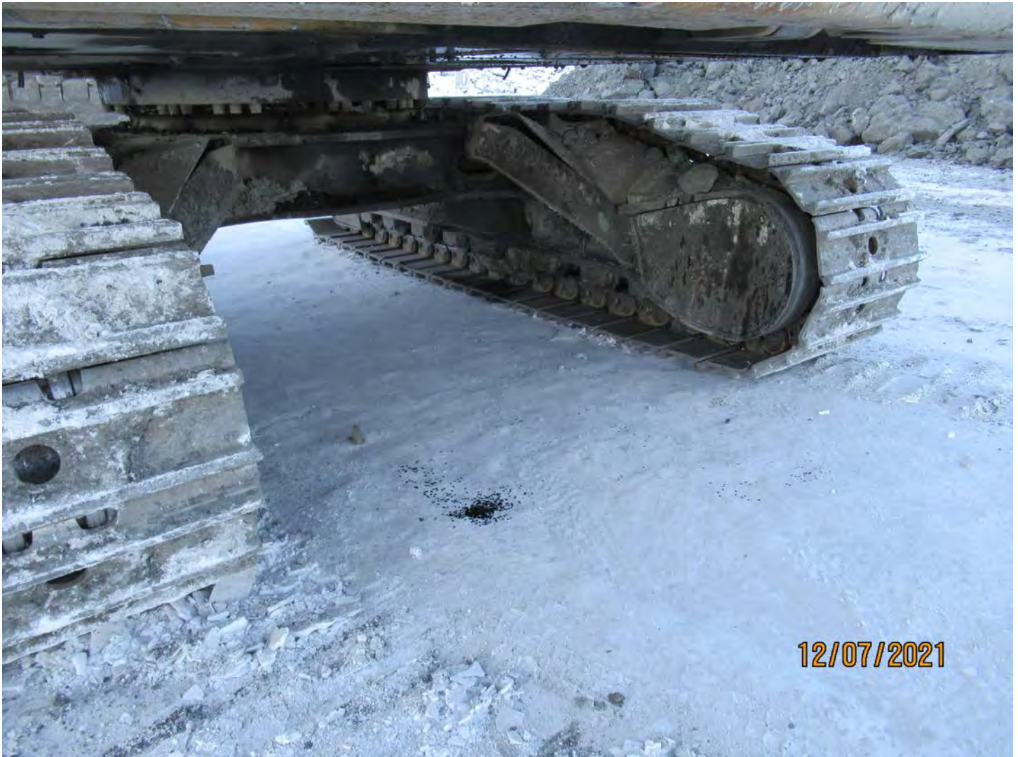
Photo 9: As seen, there was no secondary containment placed under the parked equipment and hydrocarbons were dripping onto the ground.
