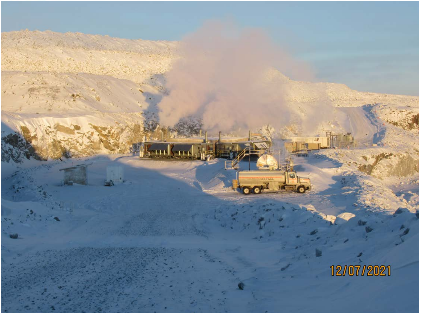
Photo 1: Looking north at the FAR station and related underground infrastructure staged at the Misery Pit 440 Bench.
