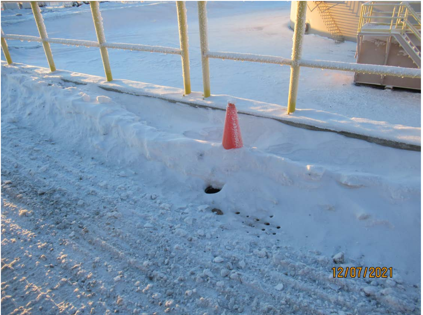
Photo 23: The sumps on the fueling ramps must be diligently monitored and cleared of snow & ice throughout the winter season.
