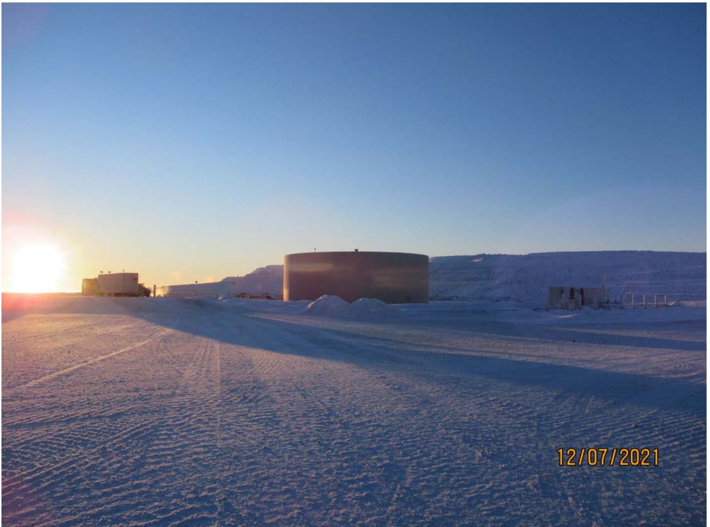
Photo 16: The Misery Pit bulk fuel tank, bulk fuel offload station (right) and the vehicle fueling area (left).
