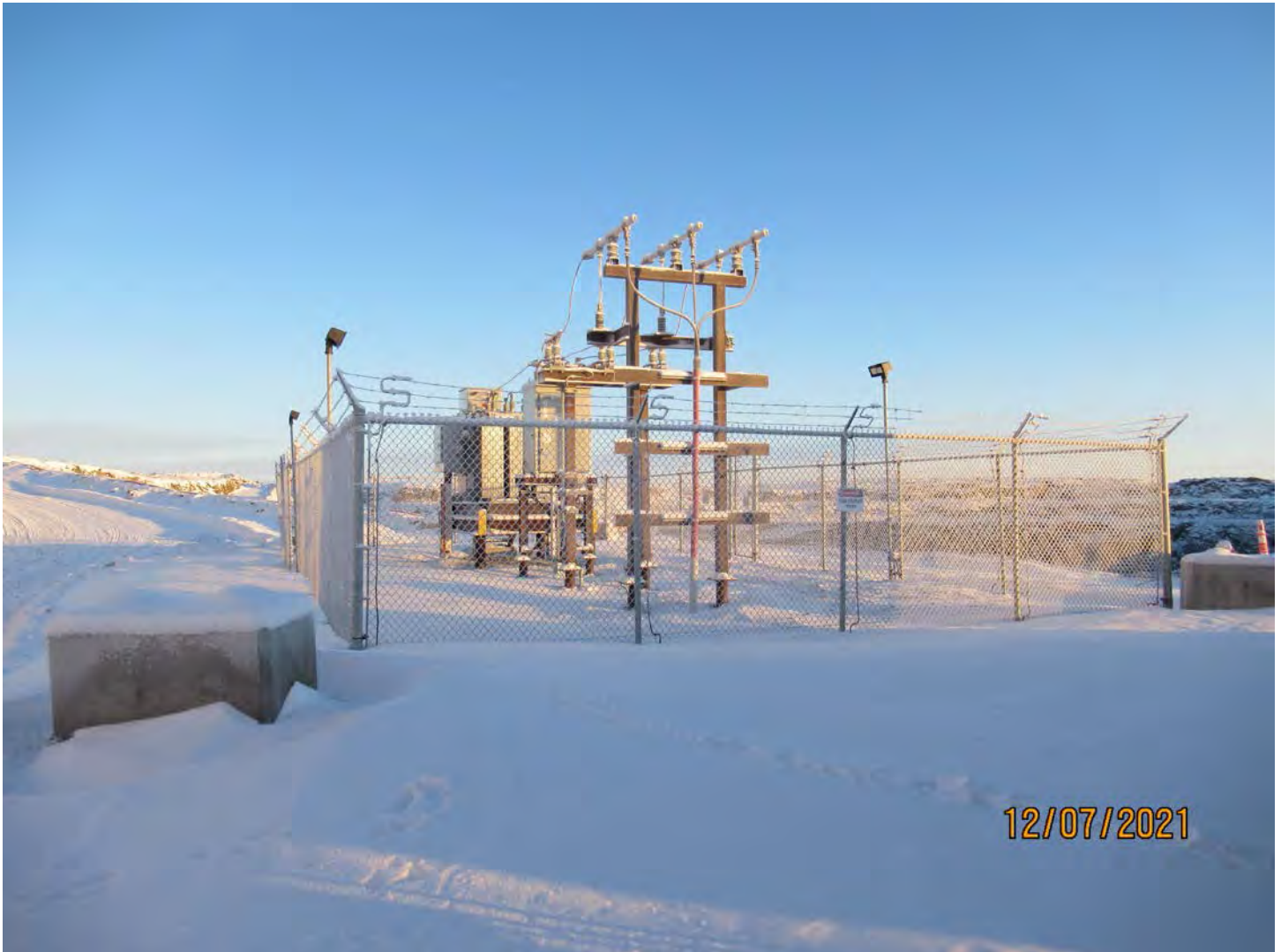
Photo 3: Looking at the electrical sub-station on the Misery Pit 440 Bench.
