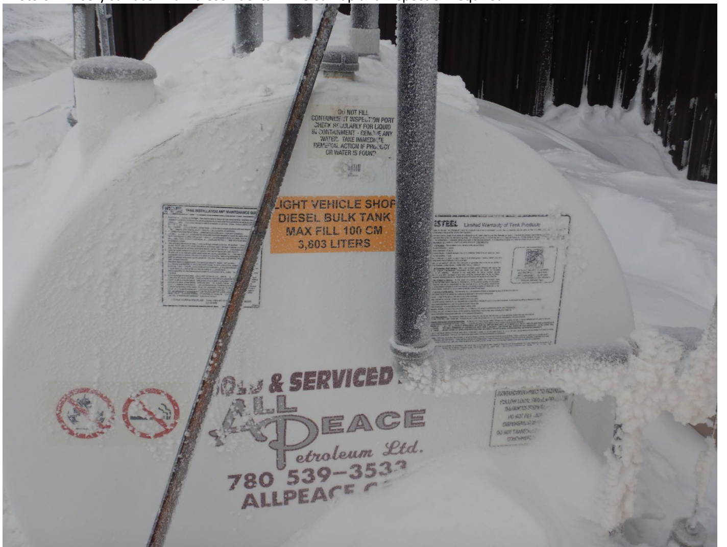
Photo 6 – Misery surface - Bulk diesel fuel tank – Clean-up and inspection required.
