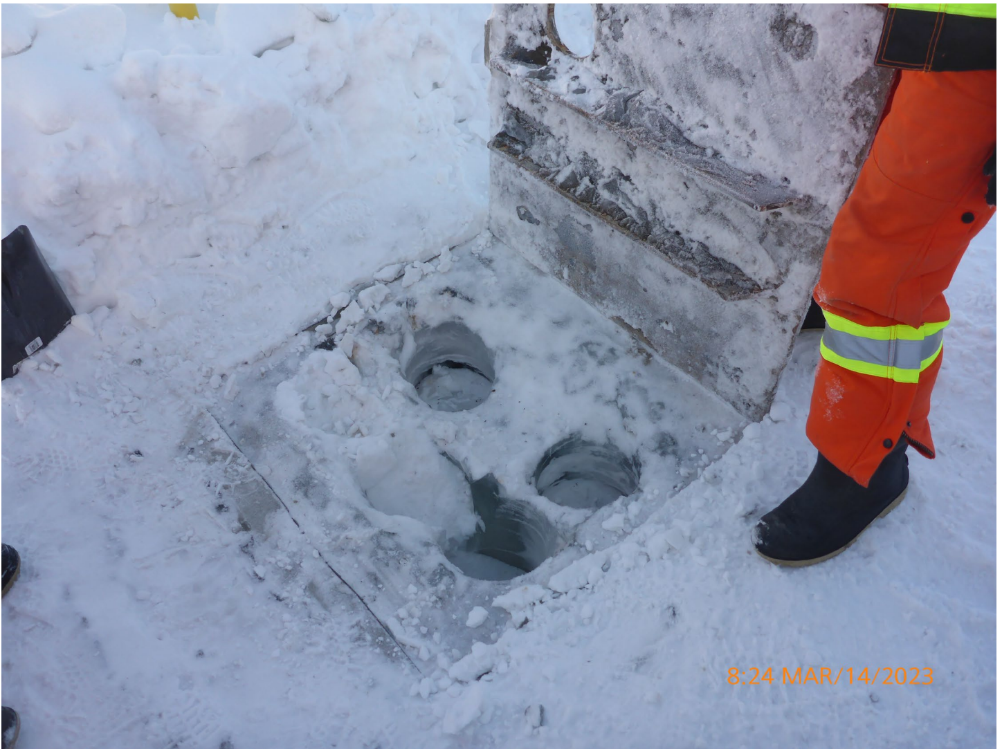
Photo 5 – Misery Refueling Station – Follow-up inspection revealed that the sump was still frozen in. Some capacity was available from some holes that were drilled in the ice, but further action is required to ensure proper spill containment. The sump will need to be thawed out and free of ice before freshet.
