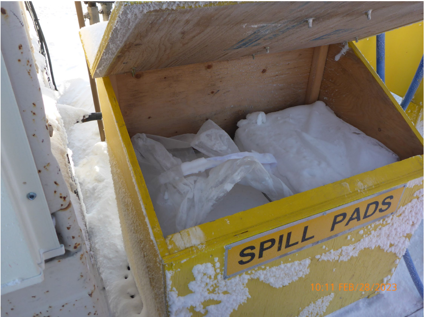
Photo 2 – Misery Refueling Station – Spill pads were well stocked to respond to minor spills.
