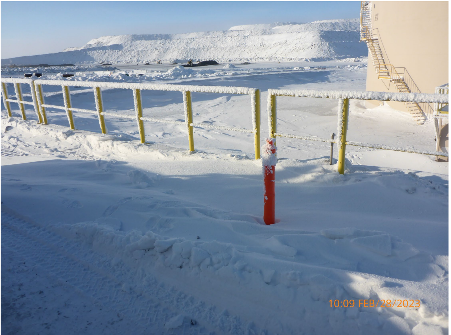
Photo 4 – Misery Refueling Station – The spill containment sump was snowed in and not functional.
