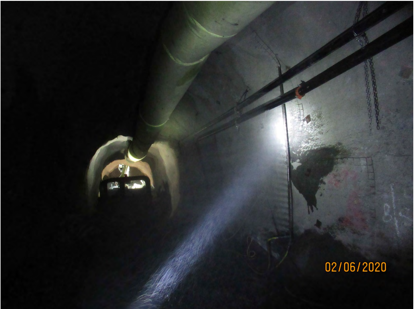
Photo 9: As part of their ground support operations, crews at the UG 2100 Level were spraying shotcrete on the surface of this drift known as Drawpoint 3. As seen in the foreground, a spray bar was being used to help suppress dust levels in the work area.
