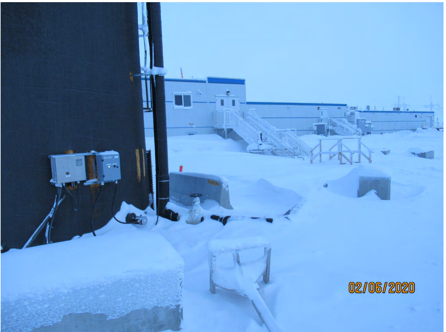
Photo 24: Sewage lines at the camp septic tank appeared intact and no spills were noted by the Inspector.
