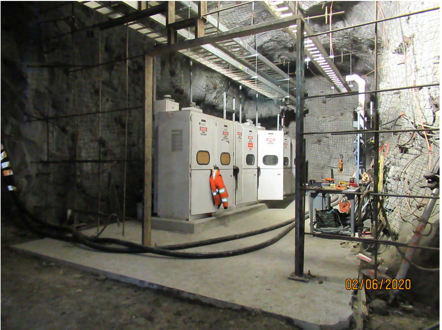
Photo 1: This electrical sub-station at the UG 2150 Level will step down electricity from an electrical transformer located on the Misery Pit 440 Bench.
