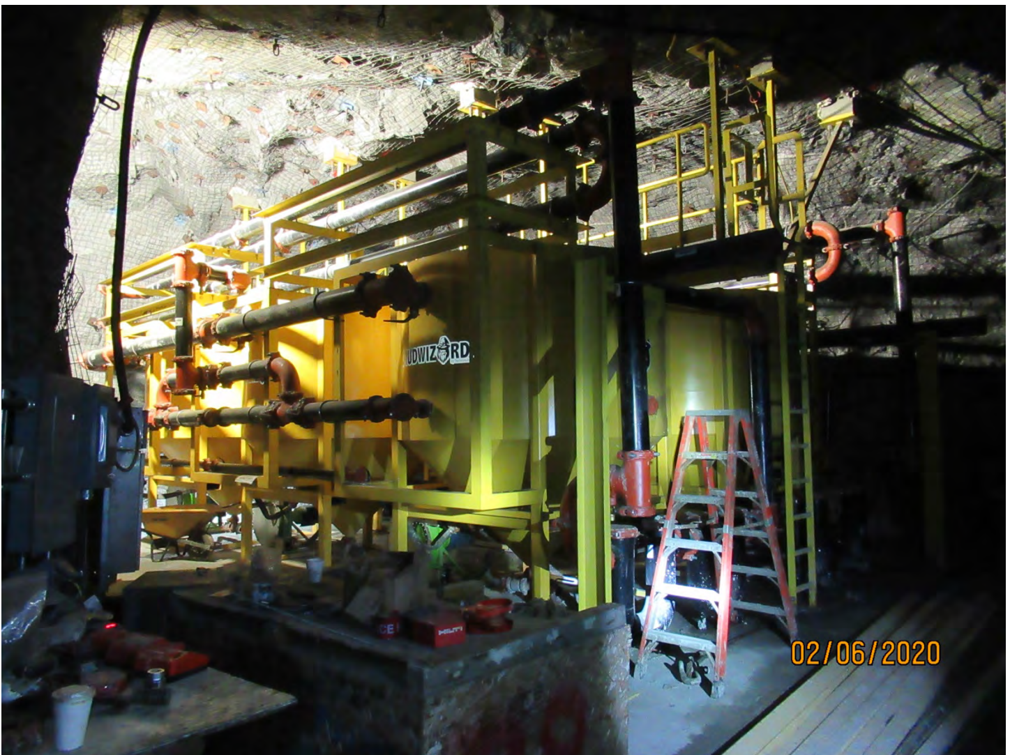
Photo 4: This MudWizard mud treatment system was being installed at the UG 2150 Level.
