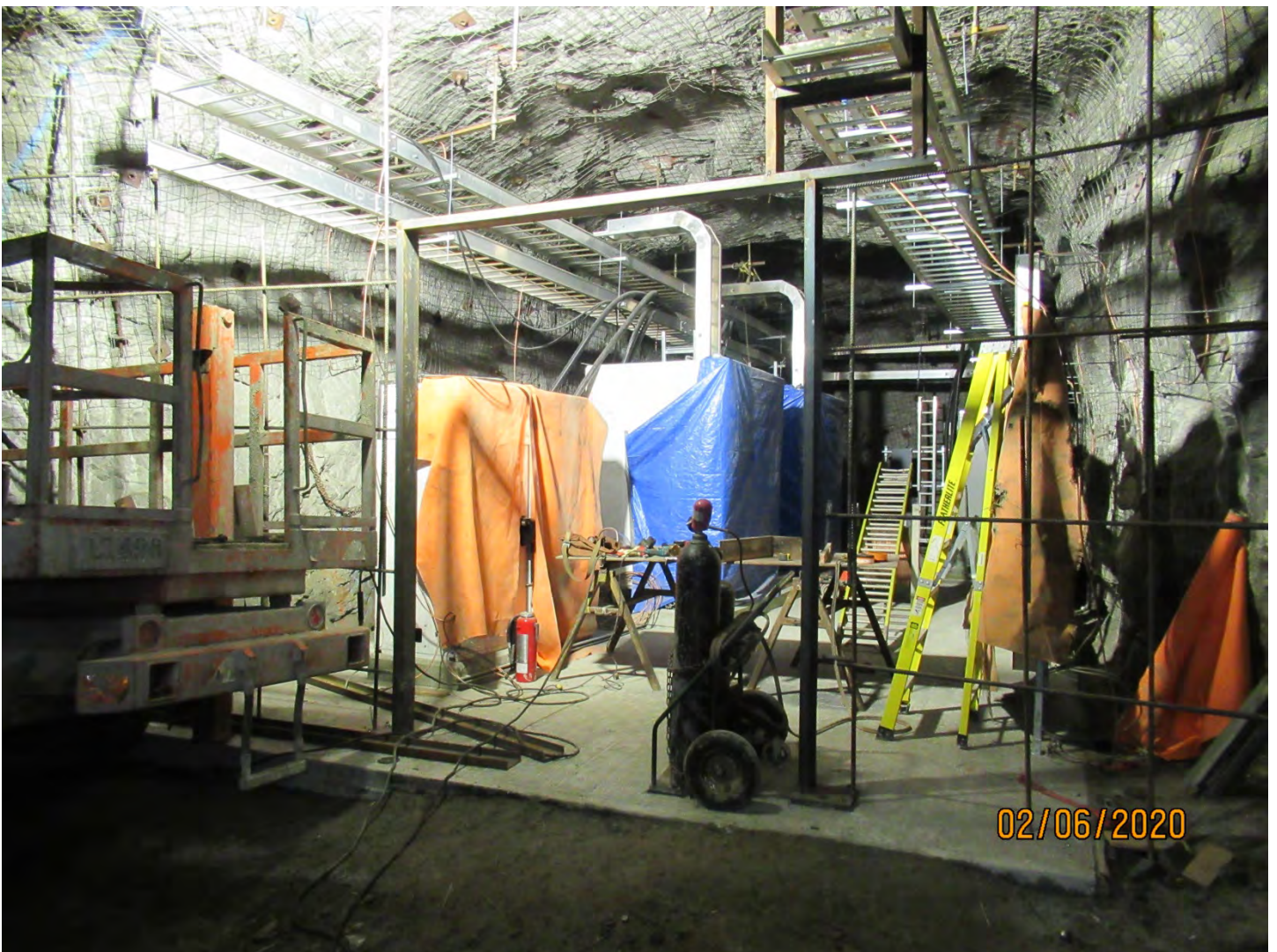
Photo 2: Electricity from the sub-station in Photo 1 reports to this electrical distribution station. Electricity will then be directed throughout the underground to support mining operations.
