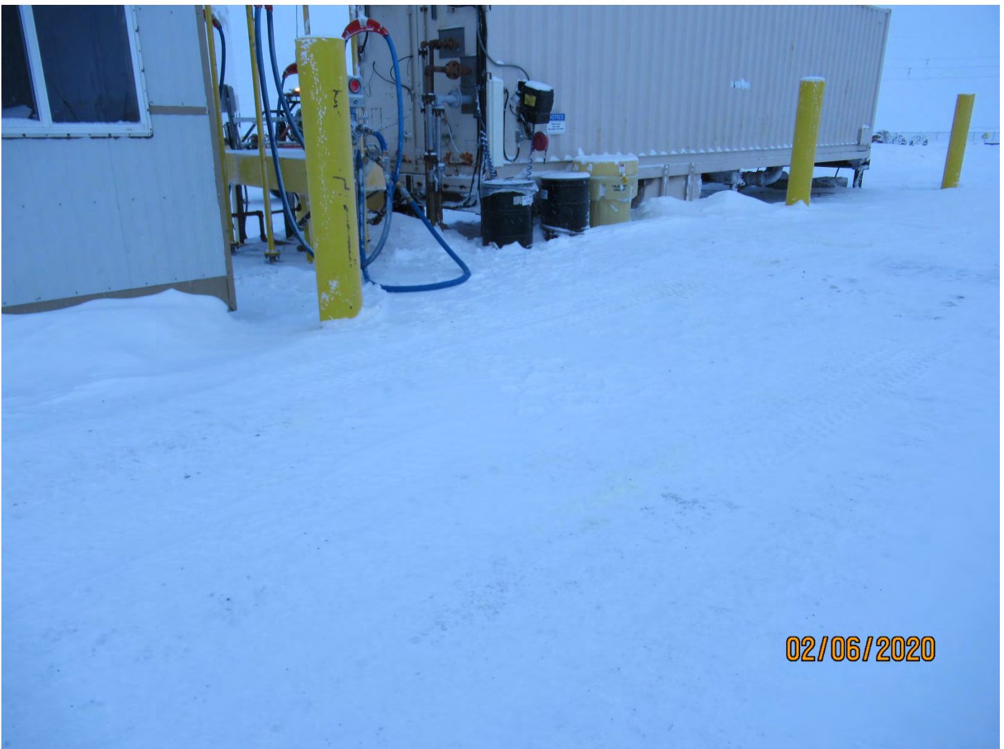
Photo 22: Though hard to see in this photo, there were hydrocarbons on the ground at the Misery Camp fuel transfer station. All spilled hydrocarbons must be cleaned up and properly disposed in a timely manner.
