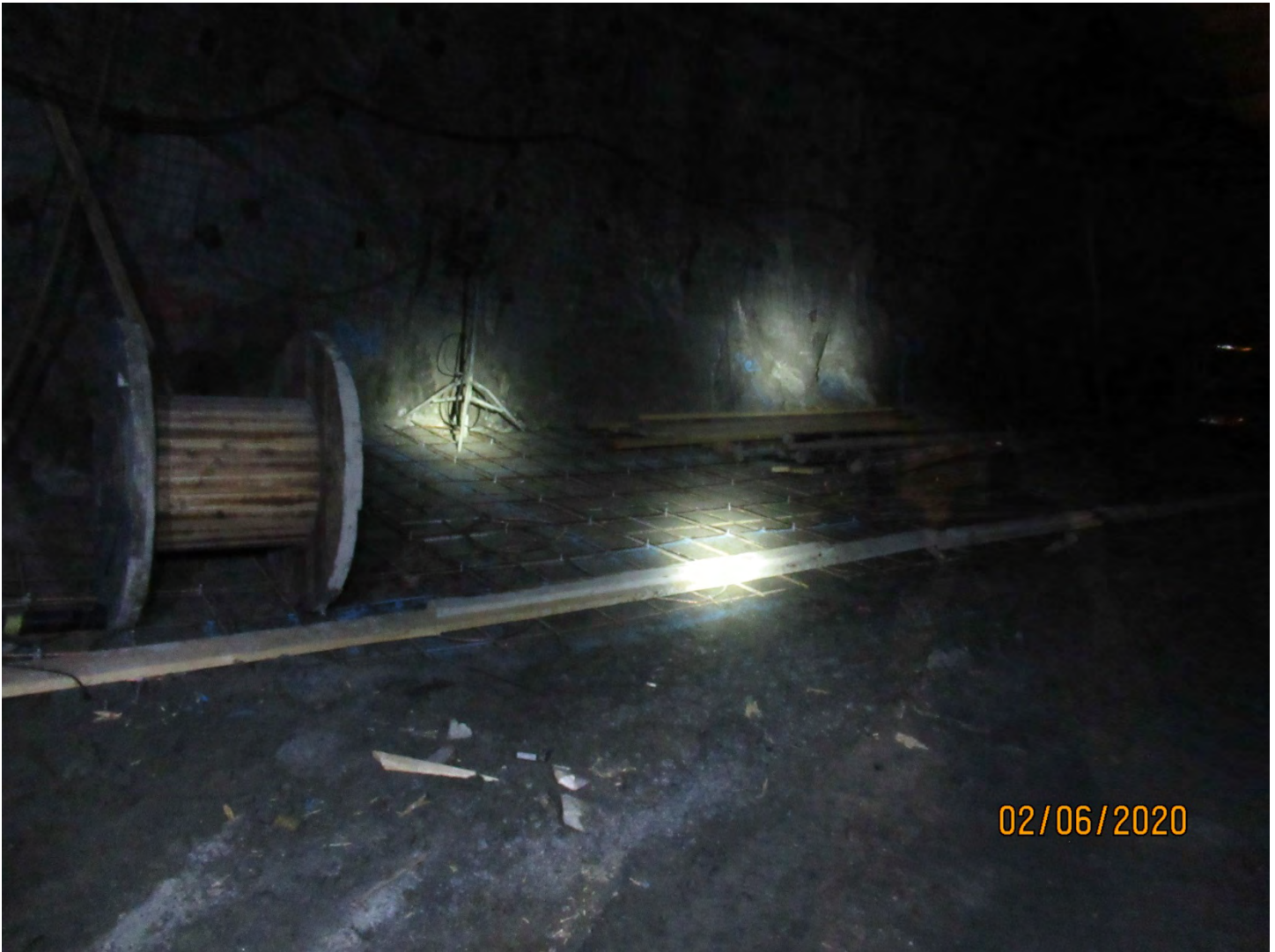
Photo 3: A concrete pad for the underground compressor station was being construction at the UG 2150 Level.
