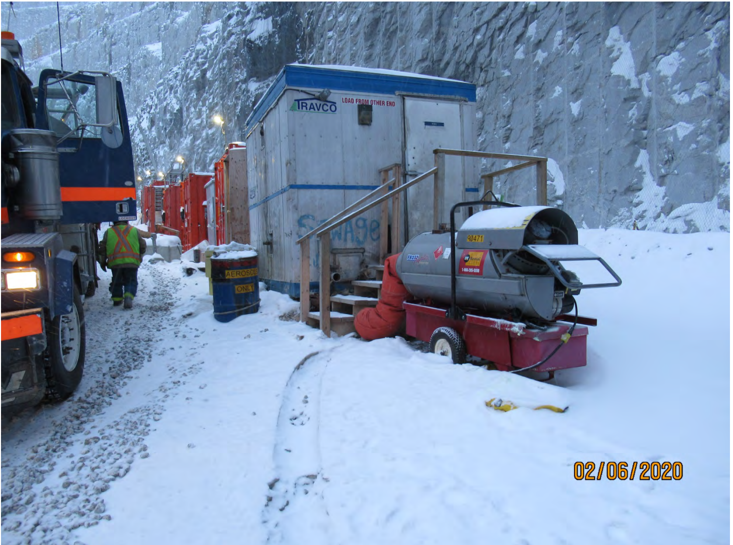
Photo 17: As seen, the secondary containment tray under this Frost Fighter was filled with snow and required maintenance.
