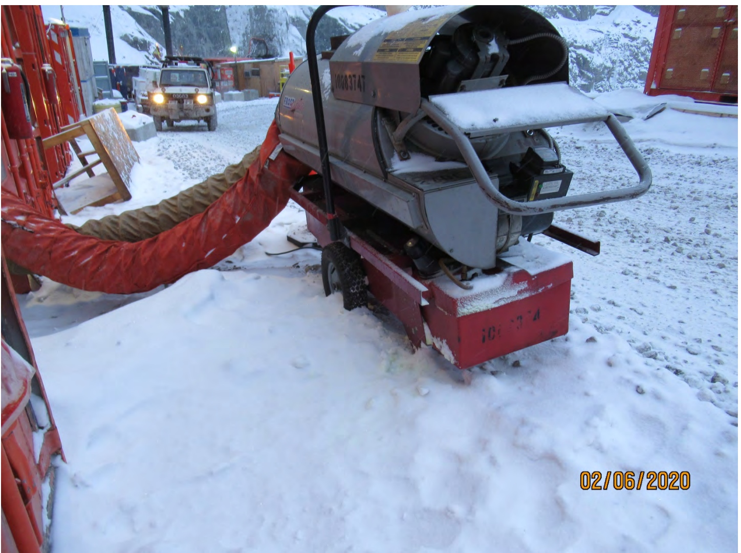
Photo 18: There was not secondary containment under this Frost Fighter and hydrocarbons were present on the ground under the area of the refueling nozzle.
