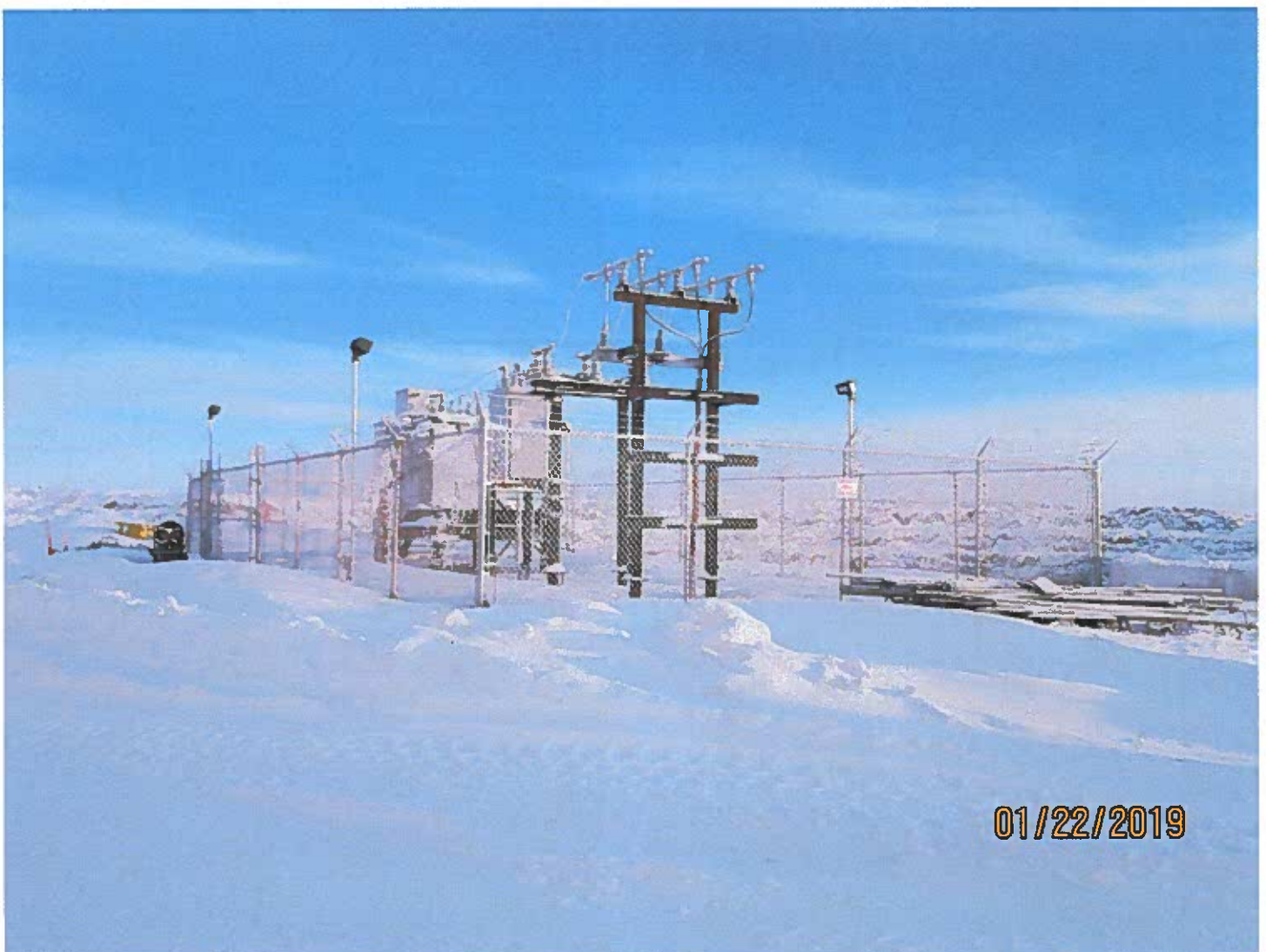
Photo #18 - W2017D0004 The Inspector was informed the 440 Bench electrical transformer is ready for operation.
