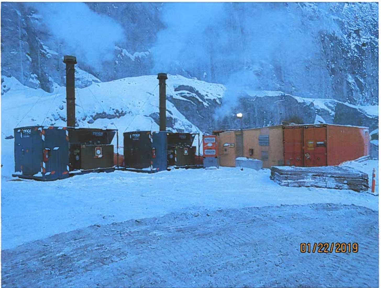
Photo #5 - W2017D0004 The underground air heaters and fan system.
