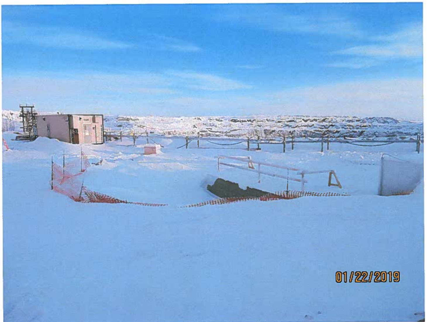
Photo #20 - W2017D0004 Though covered in snow, the concrete pad for the raise bore can be seen in this photo.
