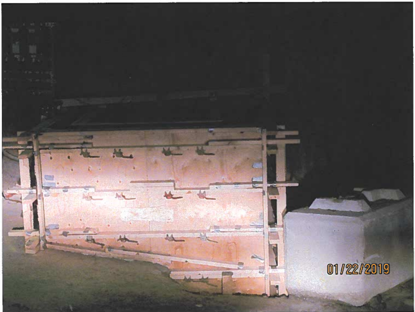
Photo #10 - W2017D0004 Concrete barriers are being put in place to protect electrical lines.
