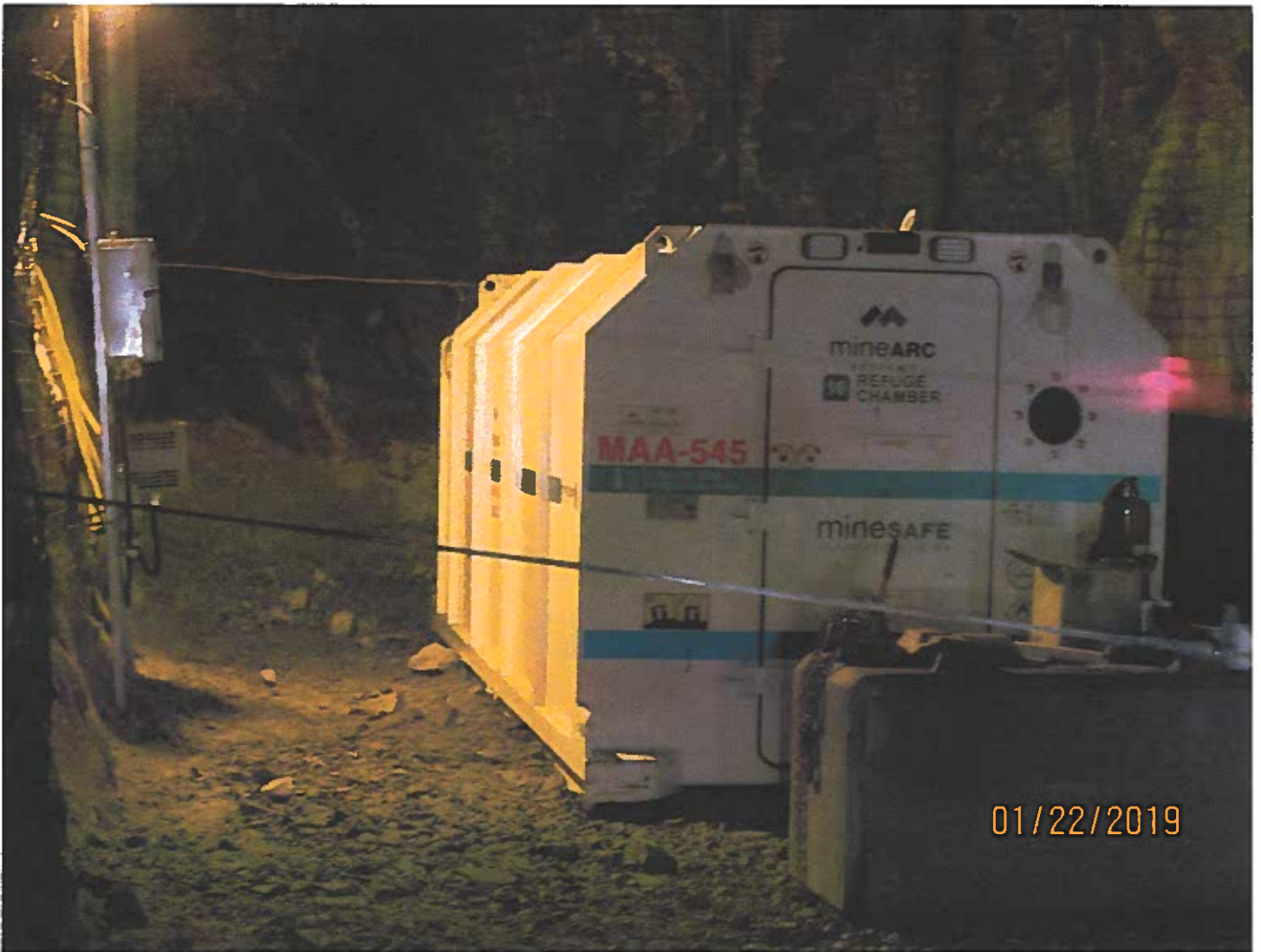
Photo #15 - W2017D0004 This MineArc refuge station is in place on the decline from the 2235 Portal in the area of the 2nd Remuck.
