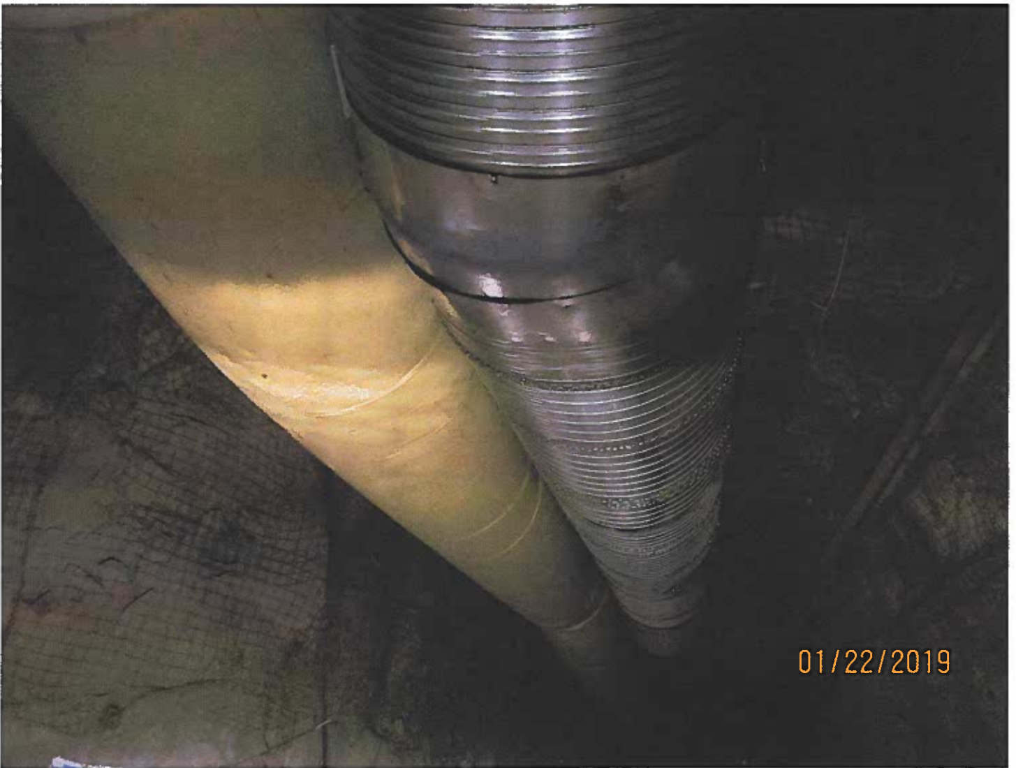
Photo #7 - W2017D0004 Air tubing within the underground is being replaced with hardline.
