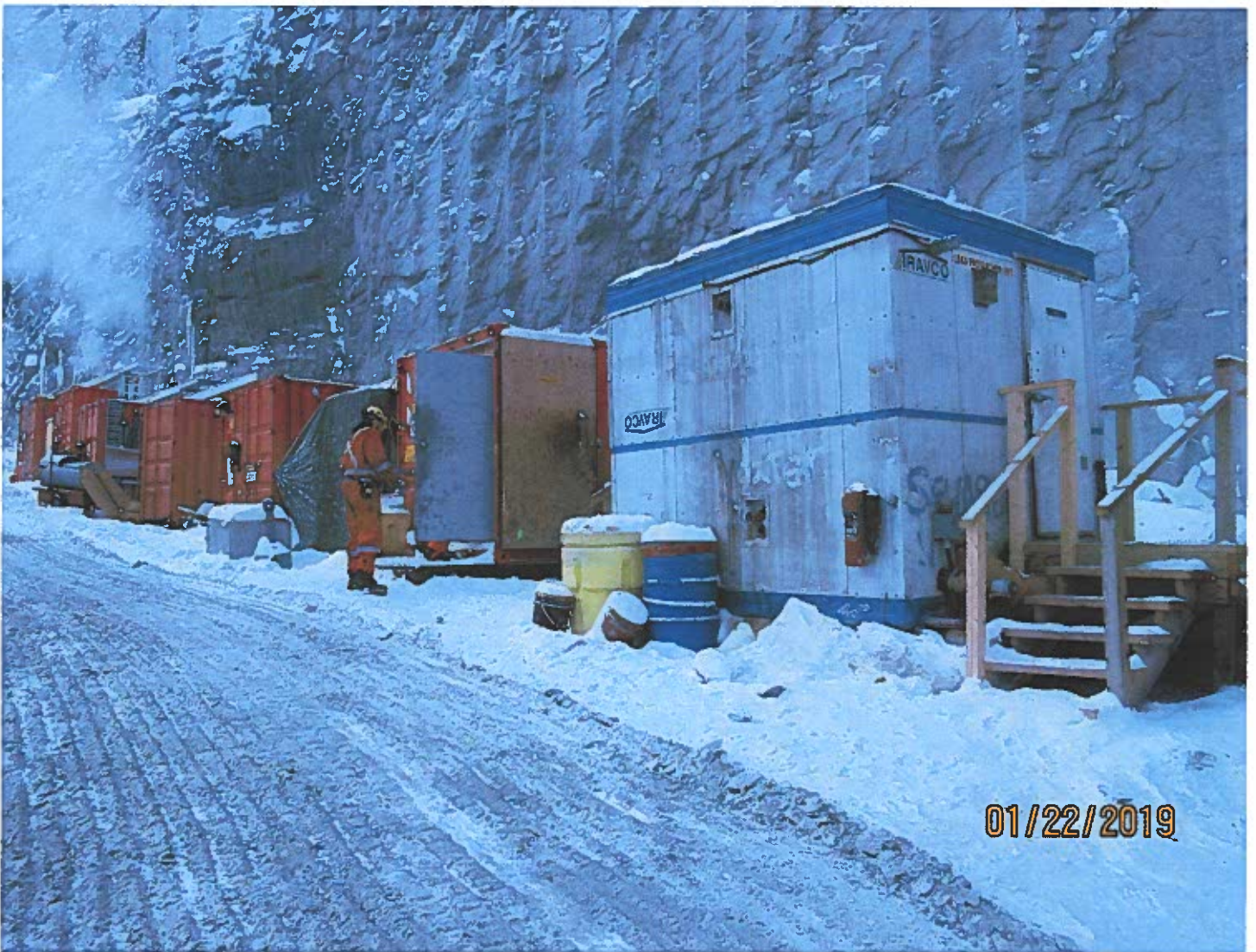
Photo #3 - W2017D0004 Another look at some of the infrastructure staged on the ramp adjacent to the 2235 Portal.
