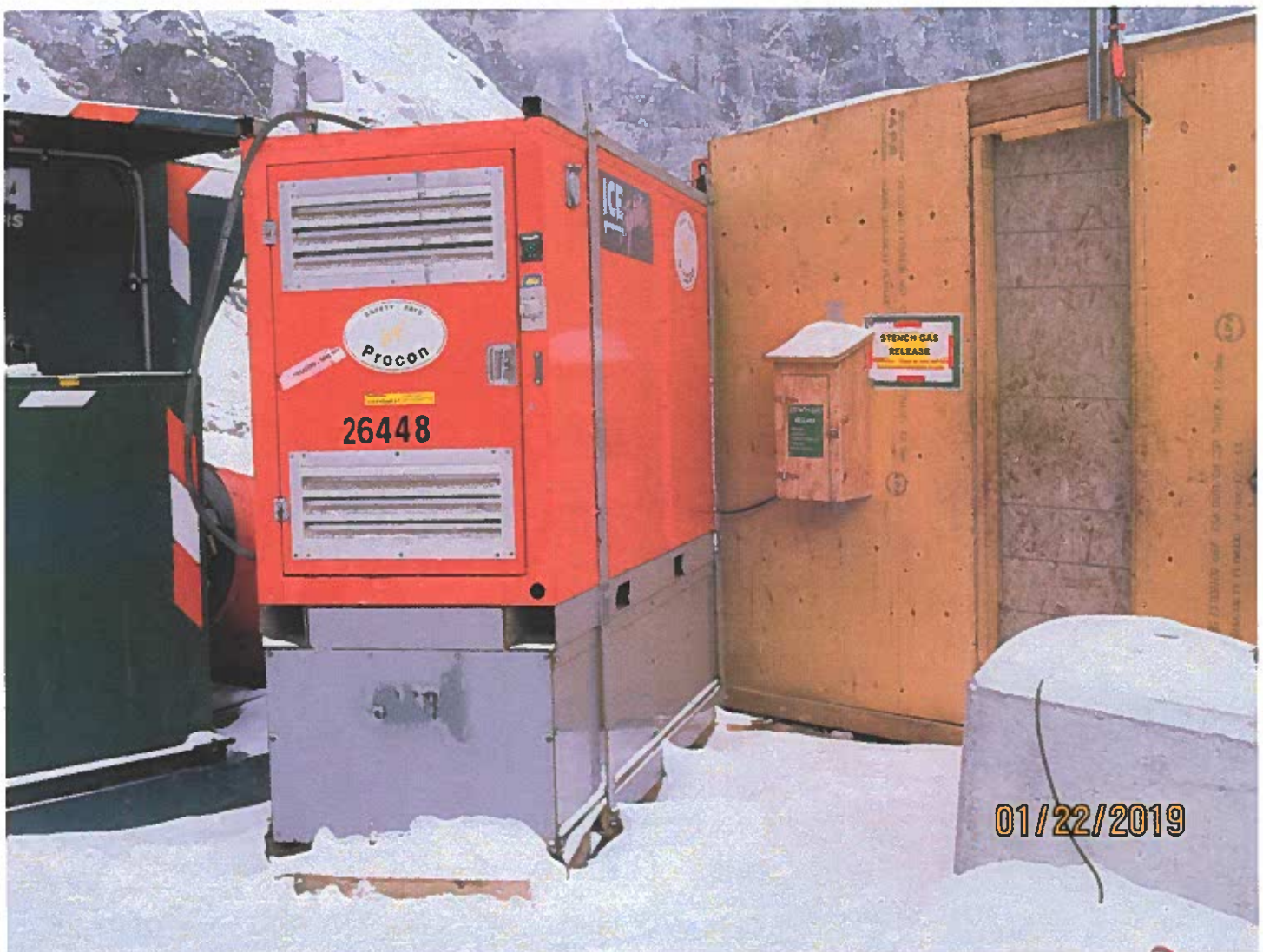
Photo #6 - W2017D0004 The added air heater (orange box) and stench gas box can be seen in this photo.
