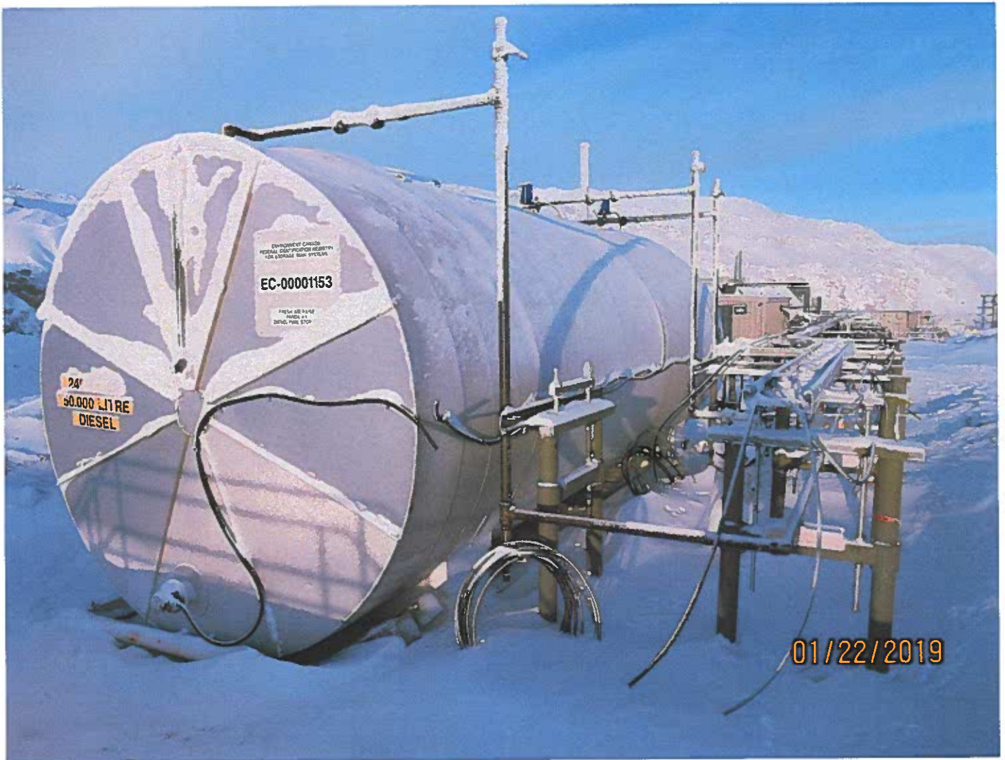
Photo #19 - W2017D0004 A 50,000 diesel tank has been put in place and will be plumbed in once the FAR becomes operational.
