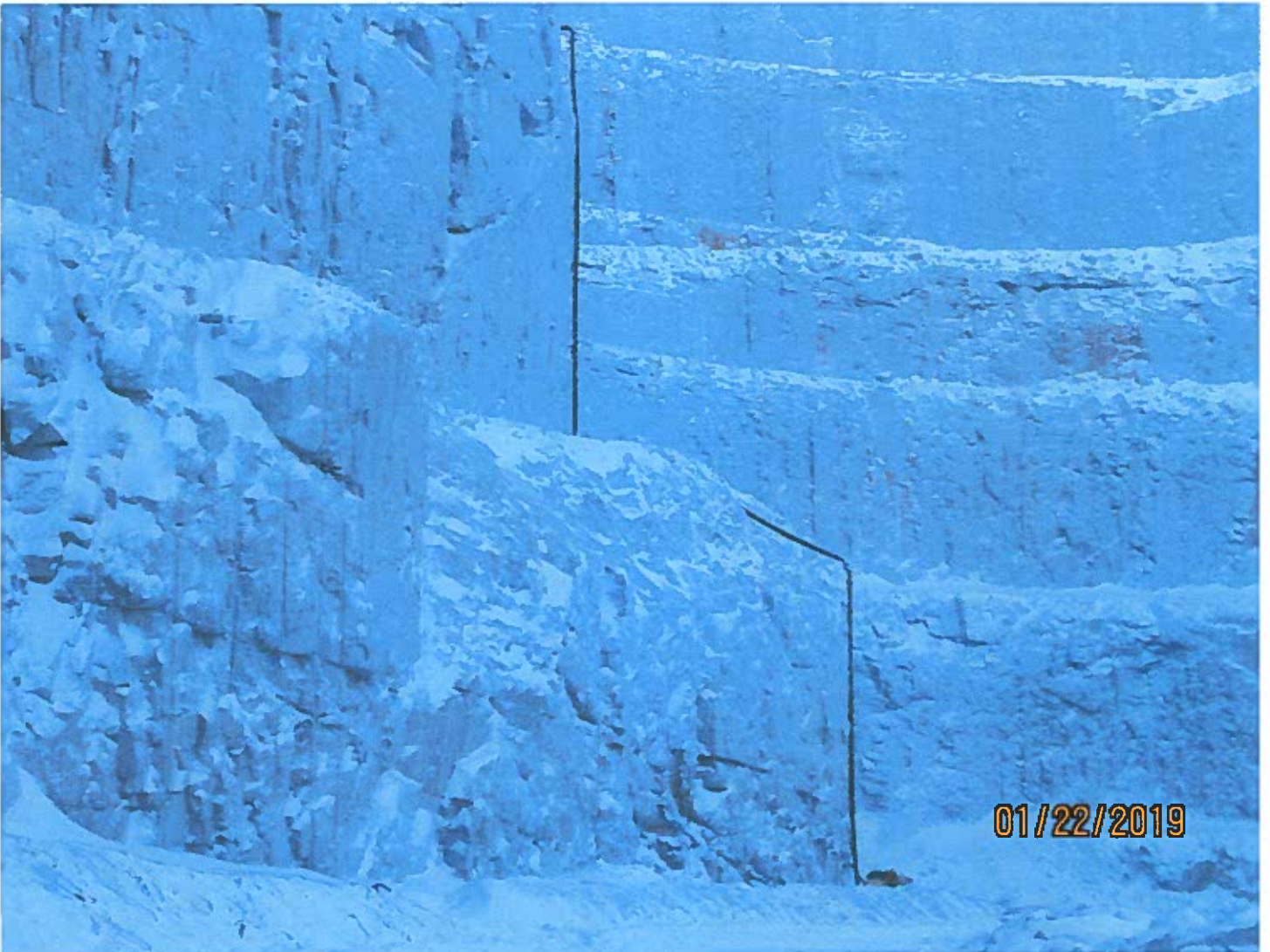
Photo #8 - W2017D0004 A dewatering line has been installed and water passed through will eventually end up in King Pond.
