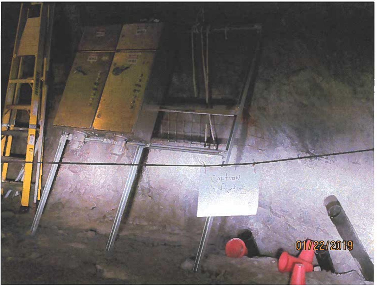
Photo #11 - W2017D0004 Electrical lines between the underground levels will be passed through protective tubing.
