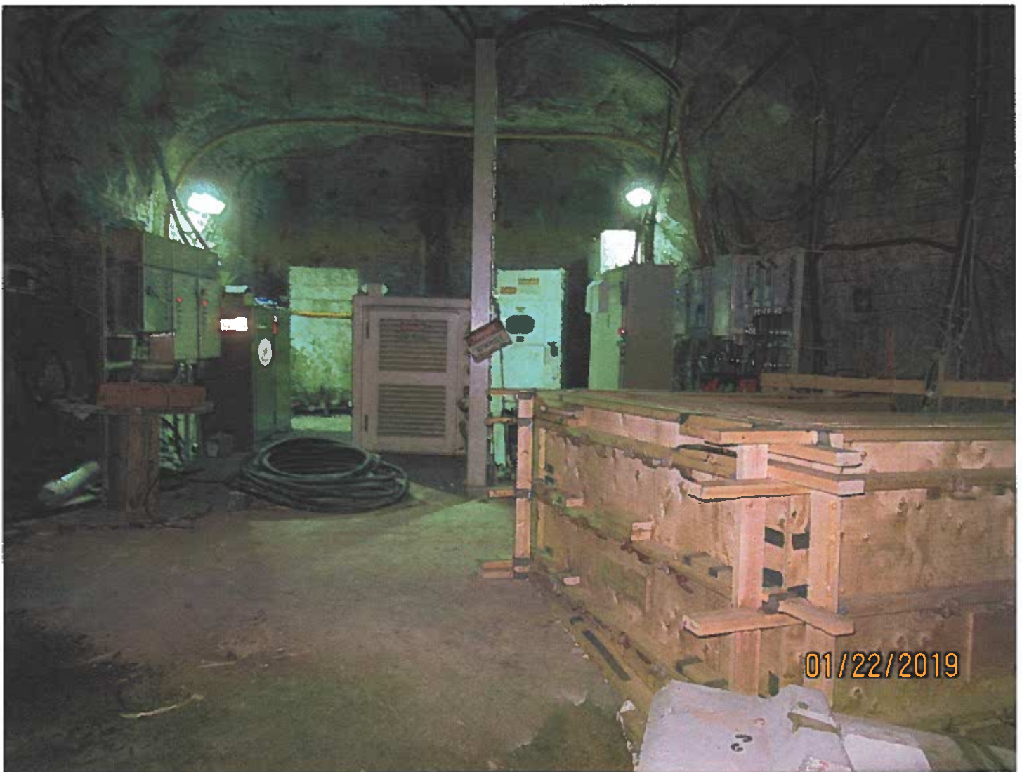
Photo #9 - W2017D0004 Electrical sub-stations are being established in key locations in the underground.
