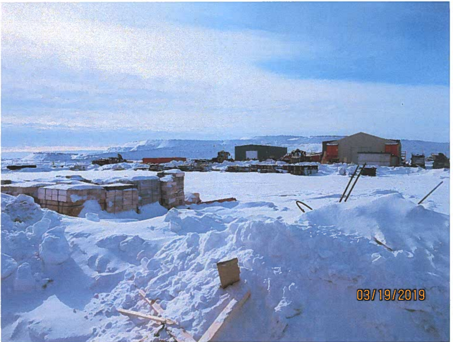
Photo #21 - W2017D0004 MUG Project This laydown behind the camp welding shop appeared organized.
