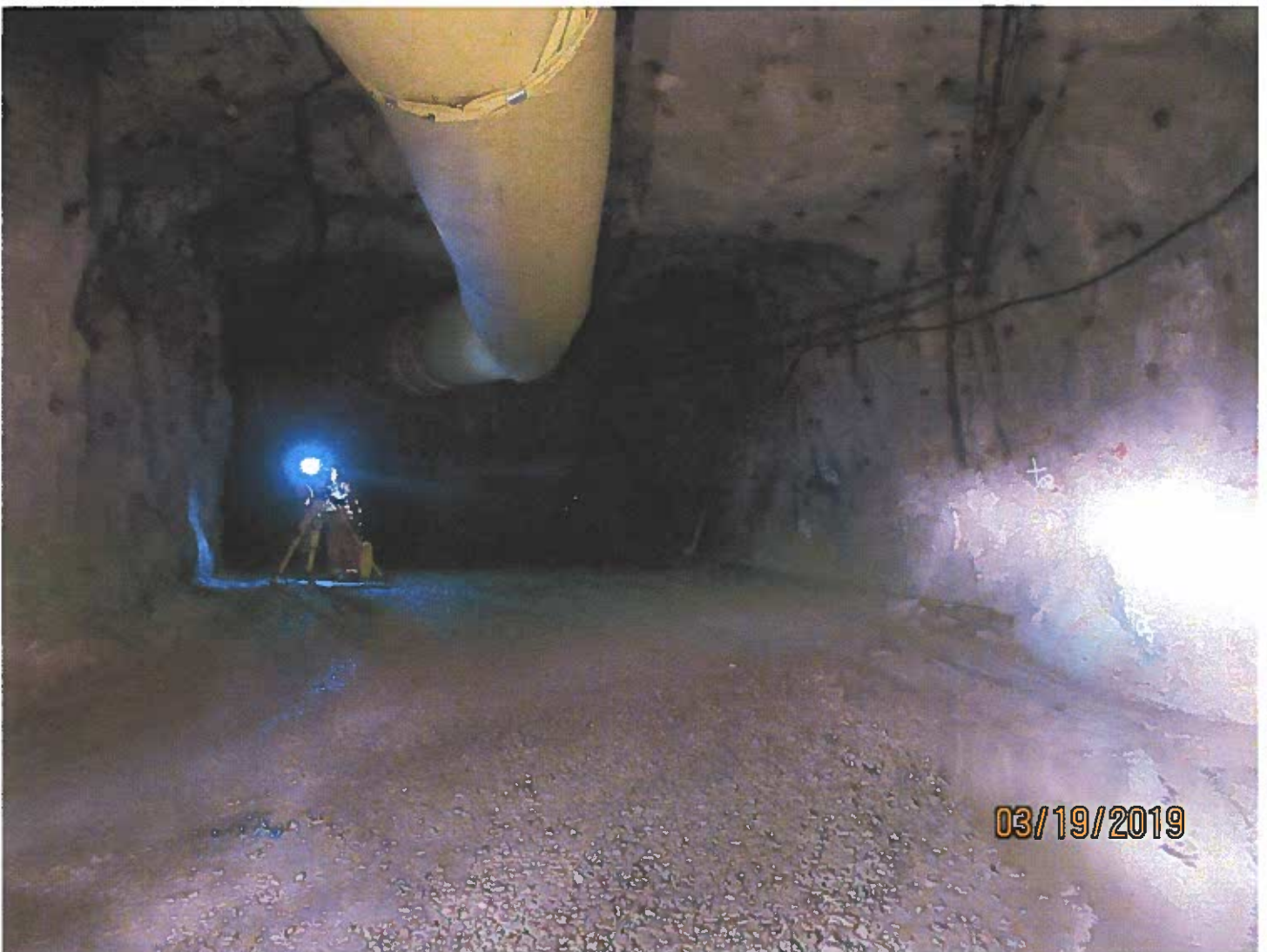
Photo #4 - W2017D0004 MUG Project Crews surveying the area for the compressor pad at the underground 2150 Level
