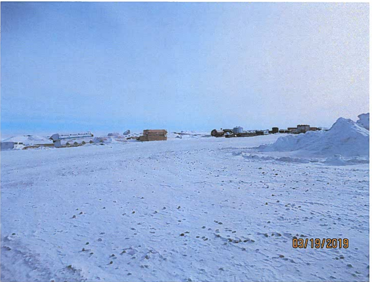
Photo #19 - W2017D0004 MUG Project The underground laydown at the top of the Misery Pit ramp.
