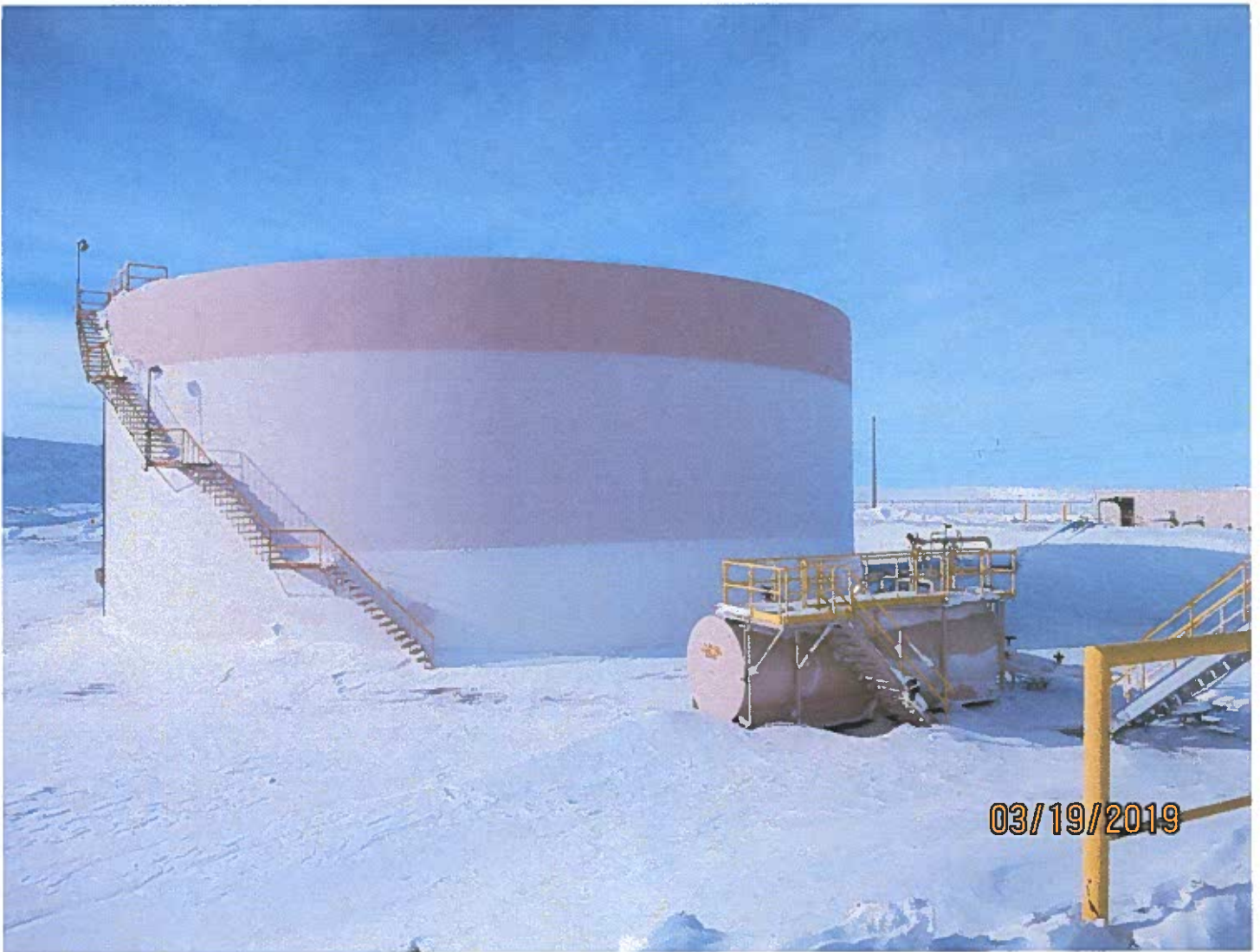
Photo #13 - W2017D0004 MUG Project The fuel tanks at the Misery Camp fuel transfer facility.
