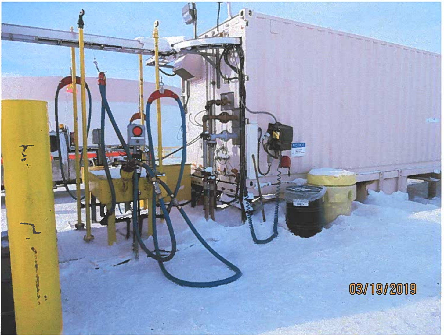
Photo #17 - W2017D0004 MUG Project Nozzles were in secondary containment and there were adequate clean up & response materials.
