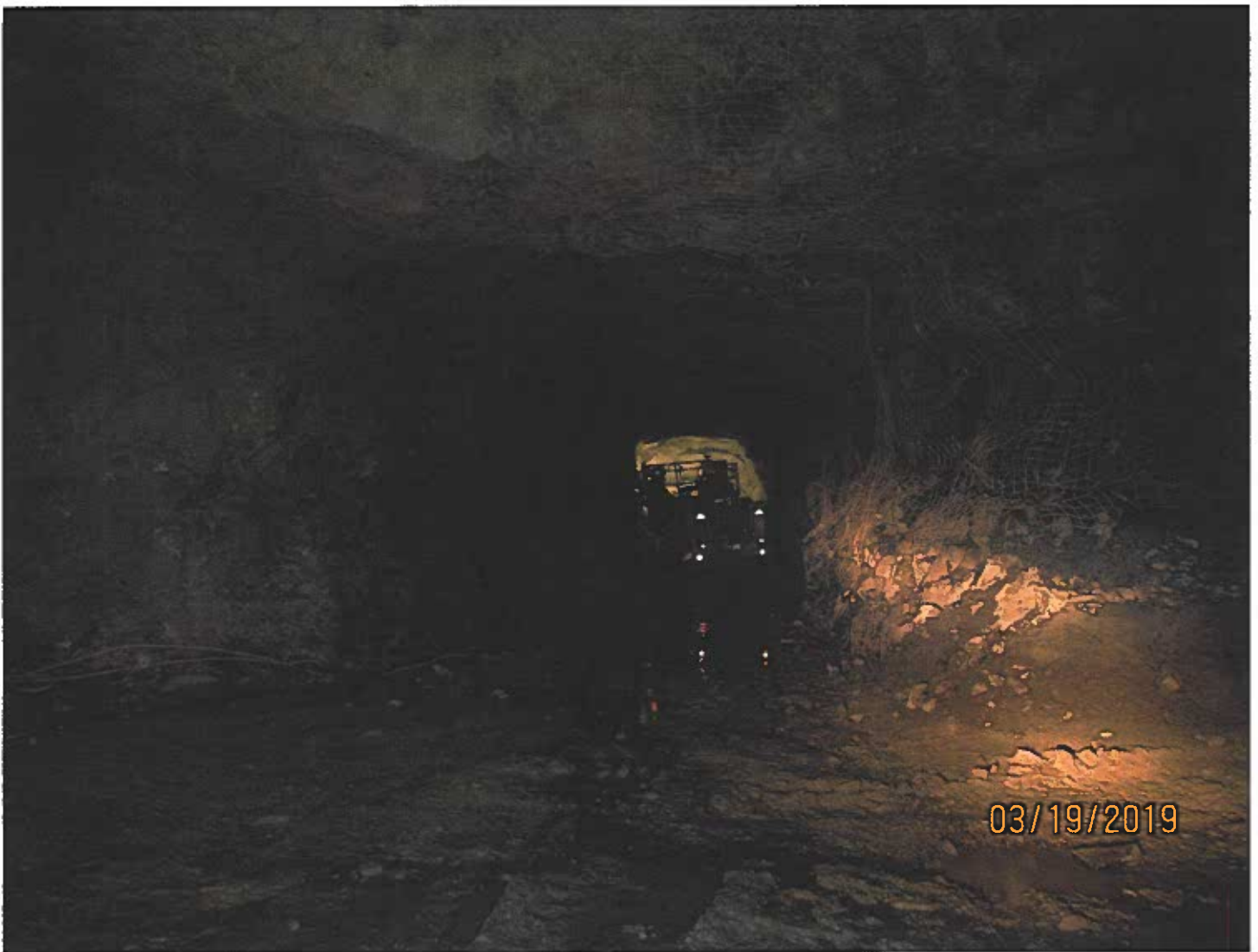
Photo #5 - W2017D0004 MUG Project Crews were establishing this dewatering drift on the 2155 Level.
