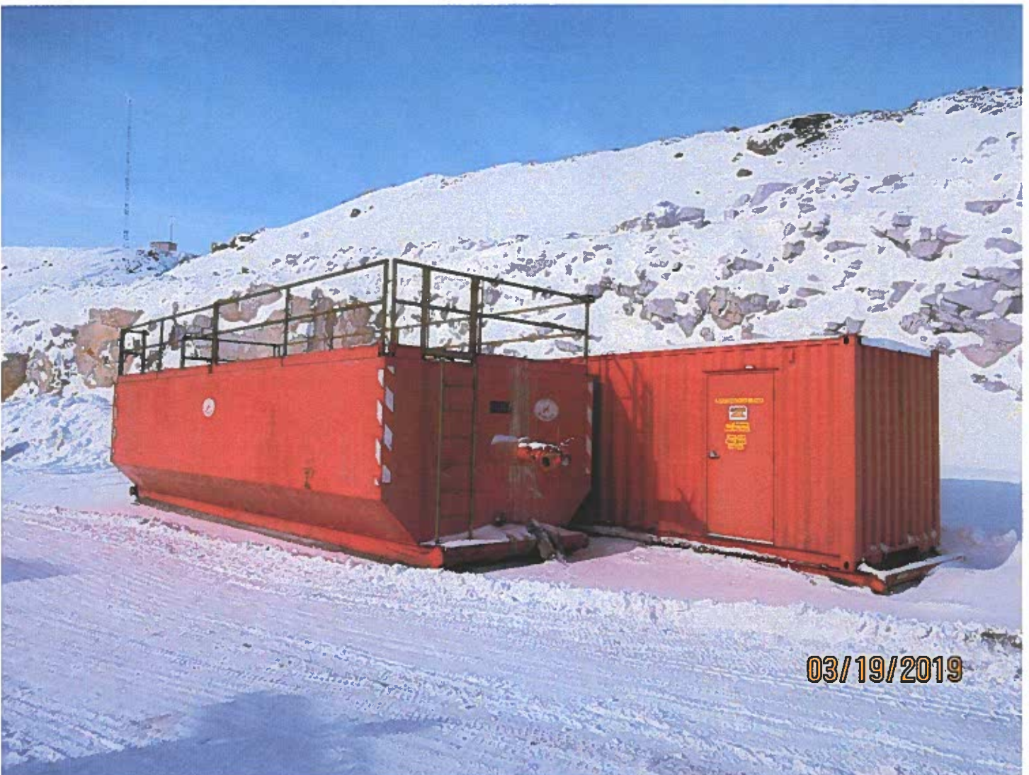
Photo #2 - W2017D0004 MUG Project This brine tank will be used during the raise bore drilling activities.
