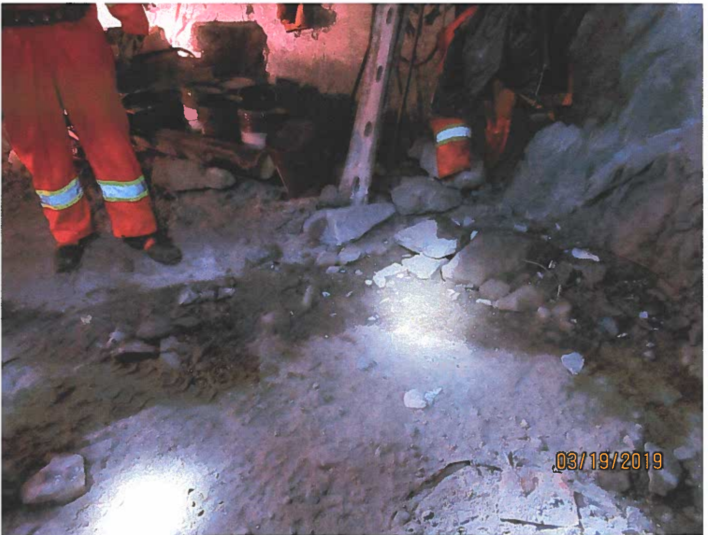
Photo #7 - W2017D0004 MUG Project Hydrocarbons were spilled on the ground as a result of improper storage.
