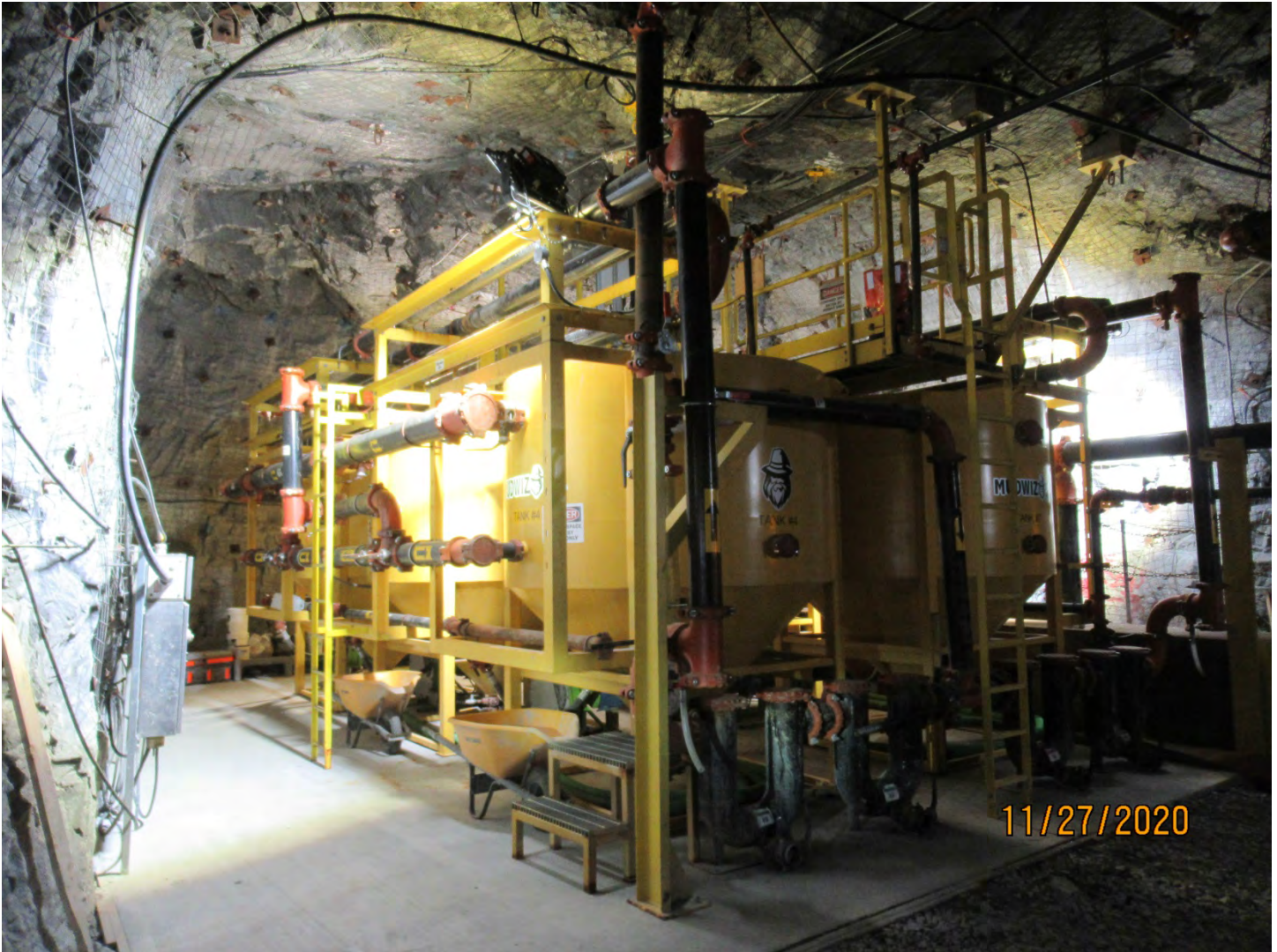
Photo 13: The MudWizard water treatment system is fully commissioned at the U/G 2150 Level.
