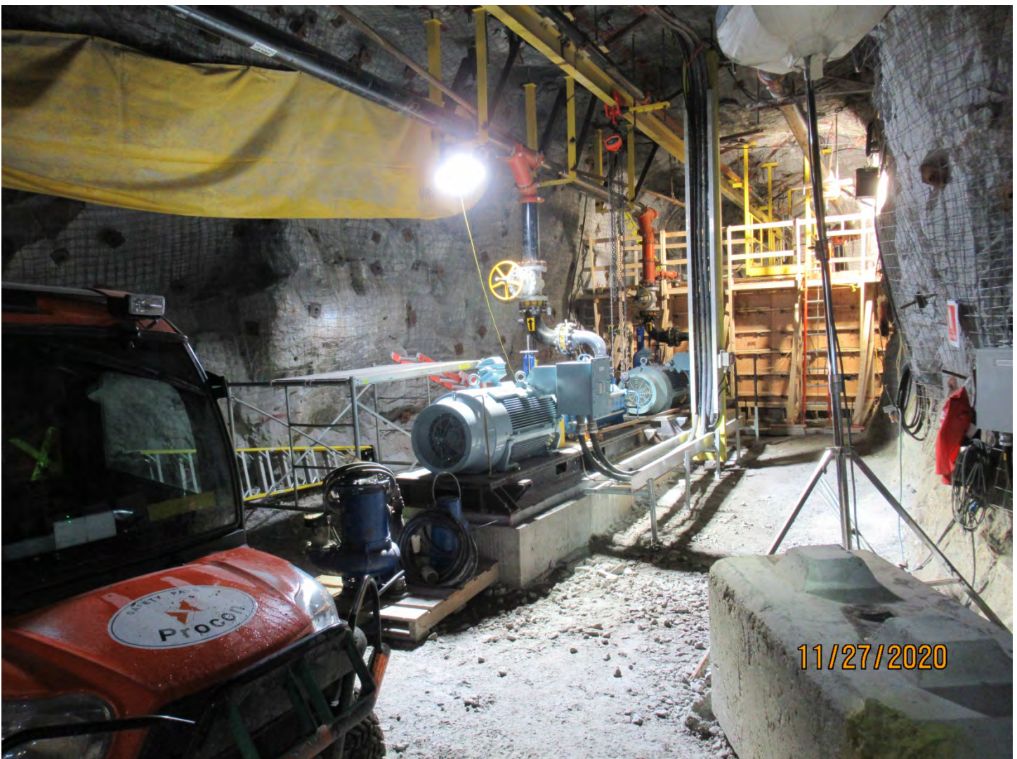
Photo 14: These 500 hp pumps are used to pump water to King Pond. In the background, concrete is being formed to establish one of the two water holding tanks.
