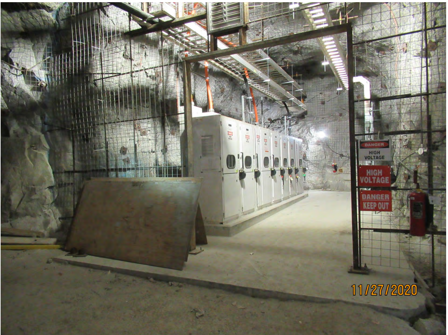
Photo 12: The electrical distribution unit at the U/G 2150 Level.
