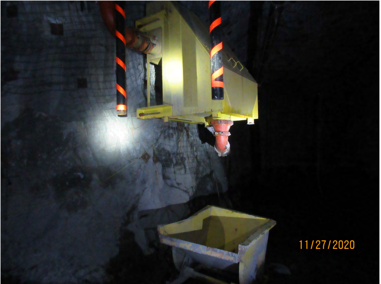
Photo 19: This screen is used to separate sediments and other debris from water in the underground.
