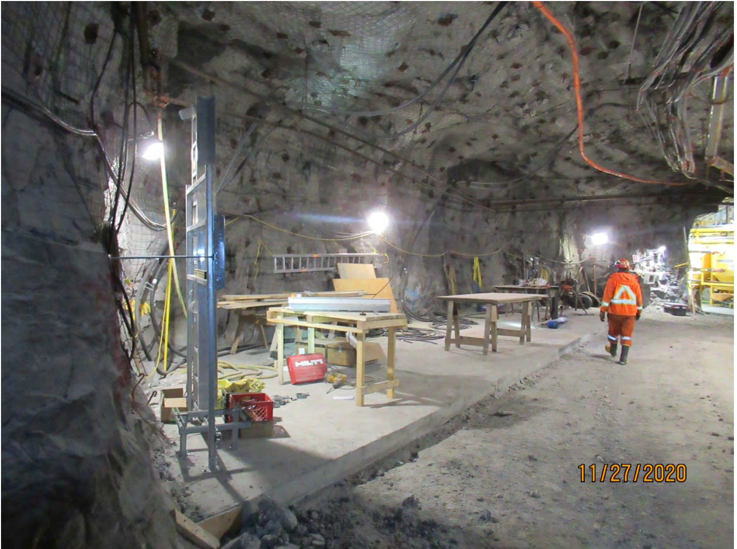
Photo 17: A compressor station will be installed on this concrete pad at the U/G 2150 Level.
