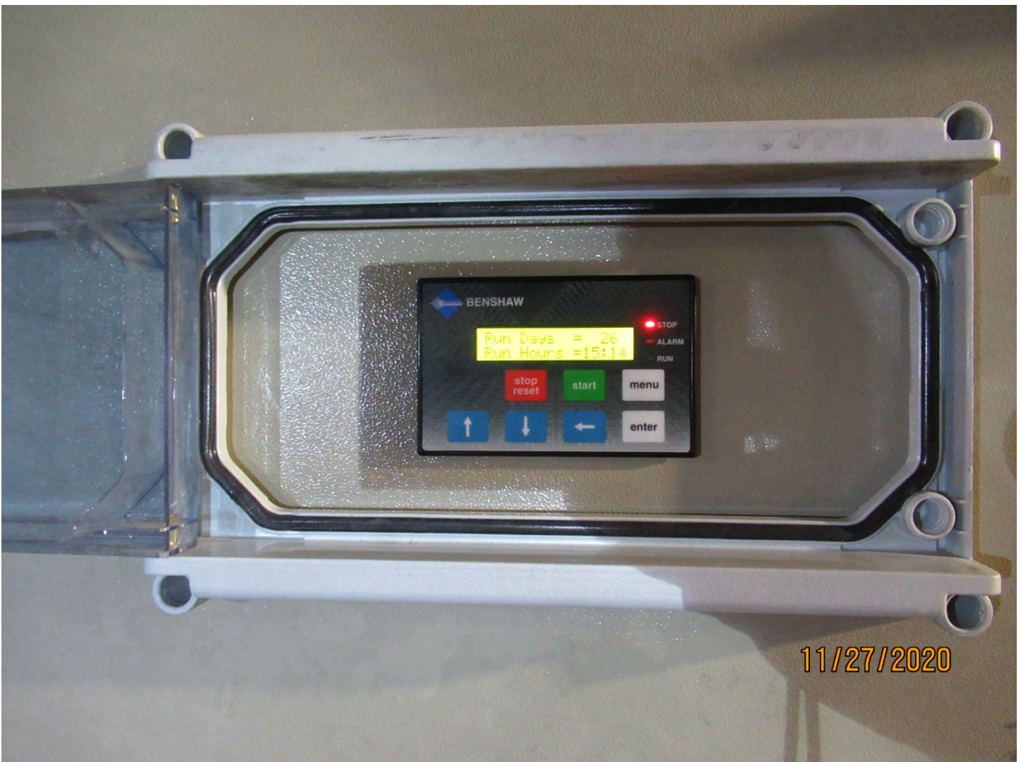
Photo 16: Water volumes pumped in the underground are currently calculated using these readings until flow meters are installed.
