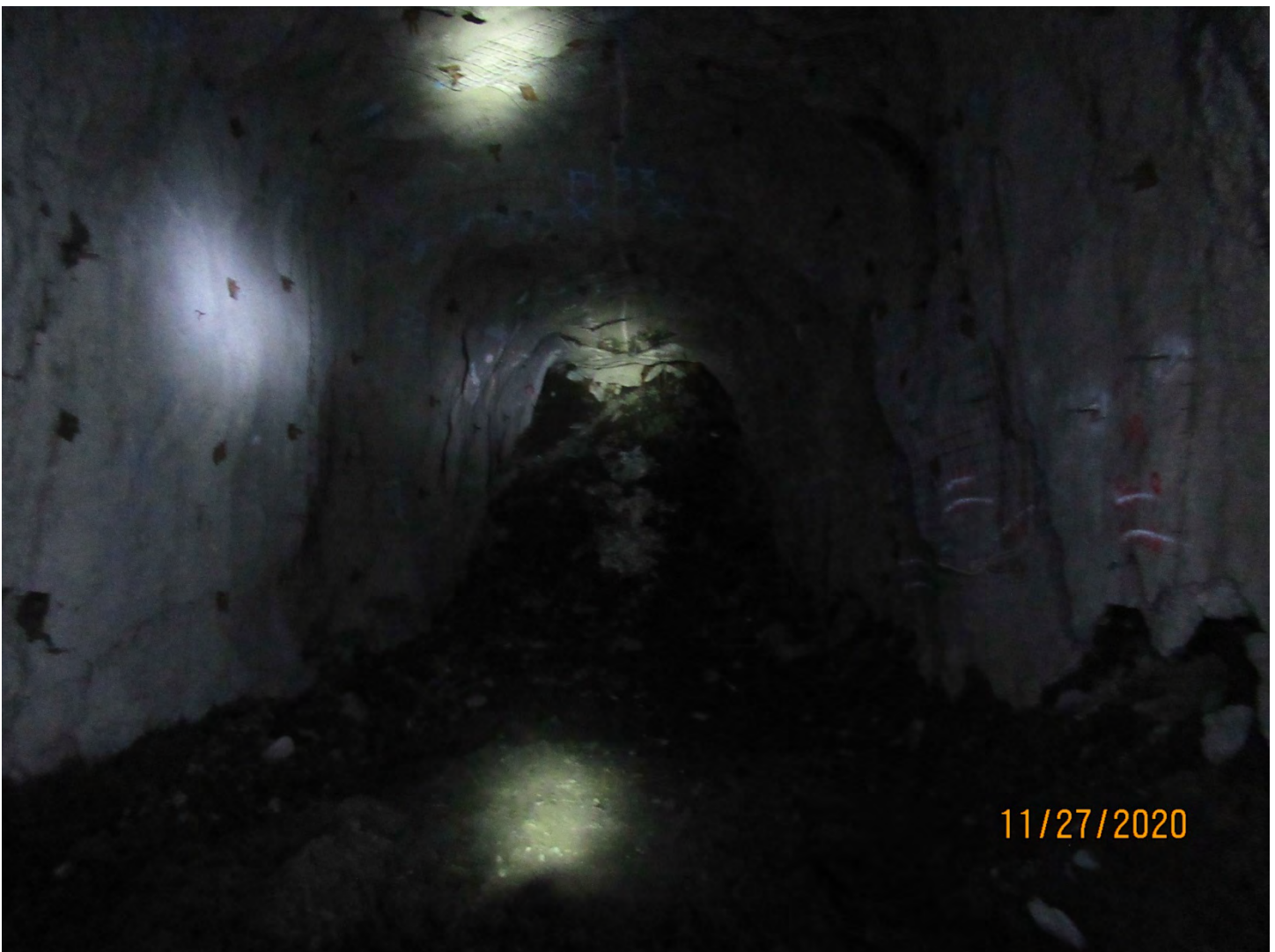
Photo 24: Blast patterns will be re-established at this production drift at the U/G 2100 Level.
