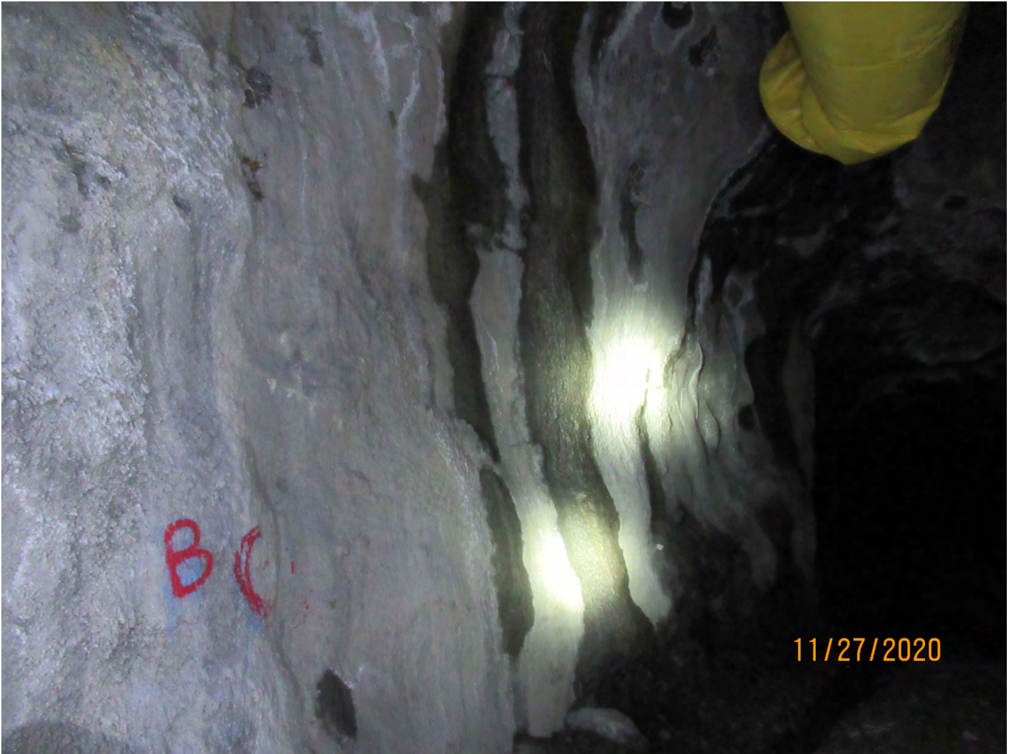
Photo 21: As seen, shotcrete was being used to stabilize production drifts at the U/G 2100 Level. Soft vent lines are installed to ensure a proper air supply in working areas of the underground.
