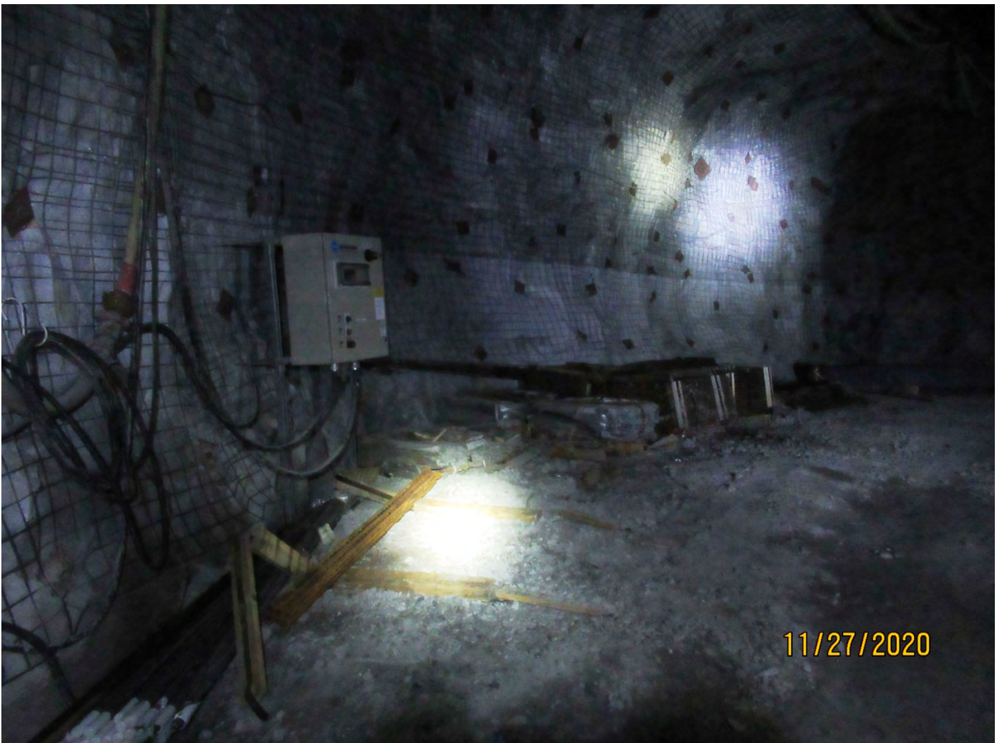
Photo 22: These supplies used in drift rehabilitation activities are staged at the U/G 2120 Level.
