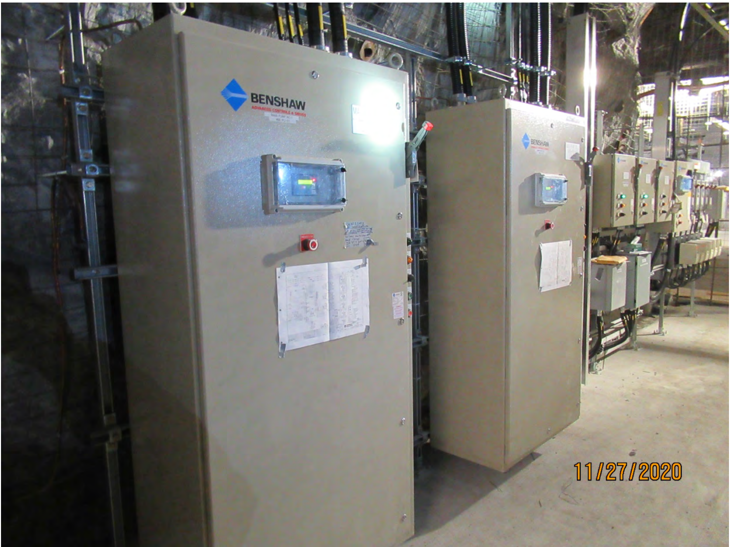
Photo 15: These control centres are used to operate the pumps in Photo #14. There is a dedicated control for each pump.
