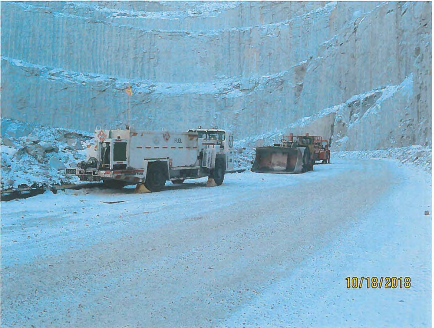
Photo #19 - W2017D0004 MUG Project Underground heavy equipment staged on the ramp adjacent to the 2235 Portal.
