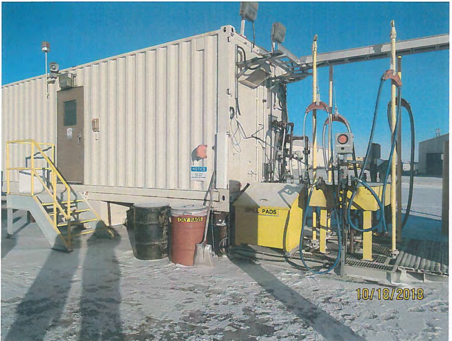
Photo #21 - W2017D0004 MUG Project There were readily available spill reponse materials present at the station.
