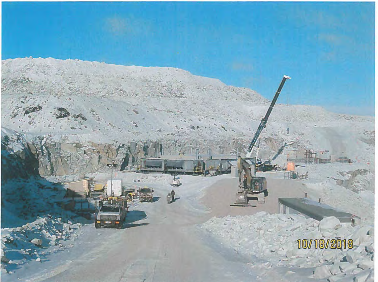
Photo #10 - W2017D0004 MUG Project Construction of the FAR building and electrical transformer (far right) along the Misery Pit 440 Bench.
