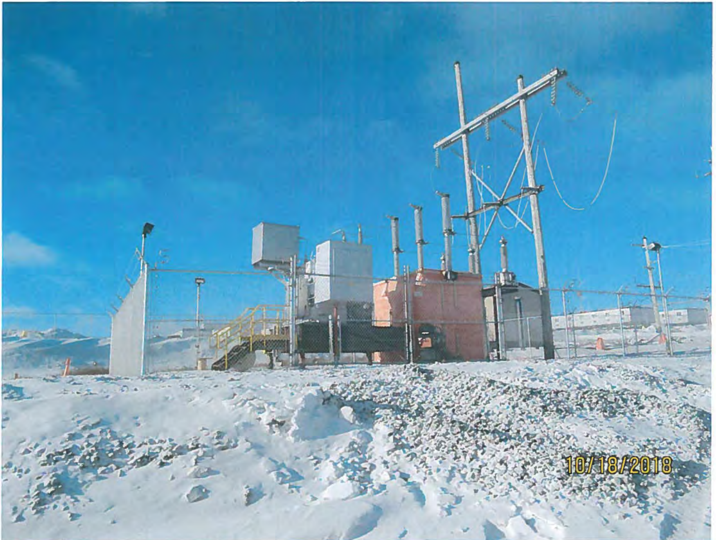
Photo #9 - W2017D0004 MUG Project Electricity from the main camp reports to this transformer and is stepped down to five (5) kilovolts prior to use in the MUG Project.
