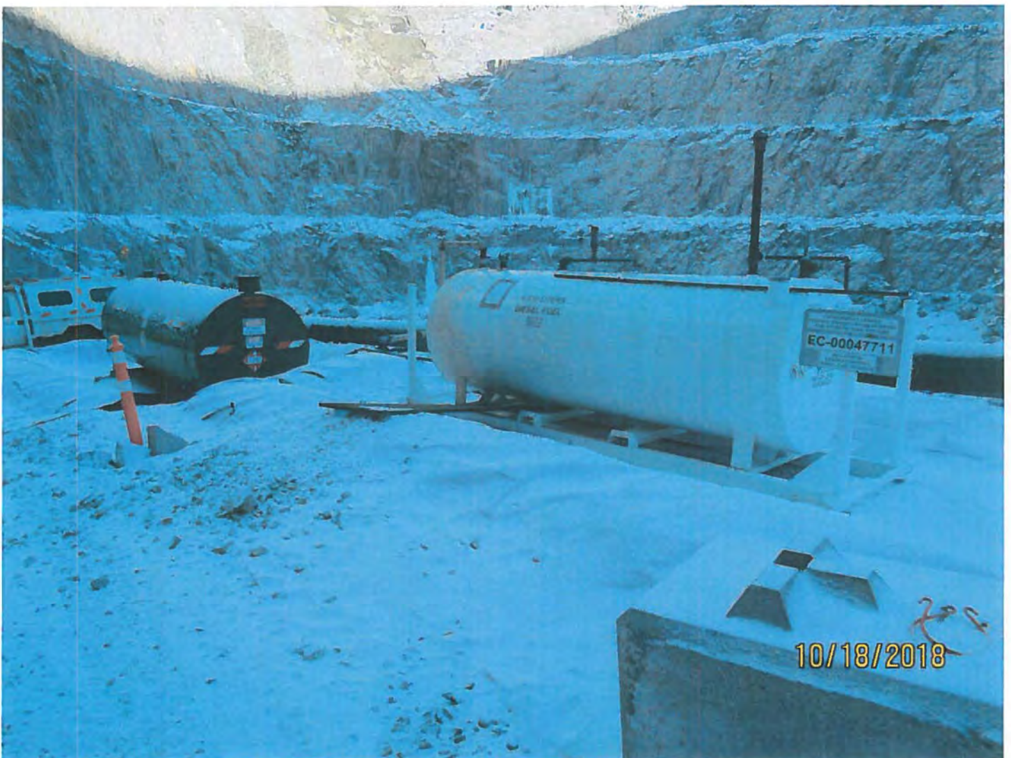
Photo #12 - W2017D0004 MUG Project The 4,530 L tank staged on the ramp adjacent to the 2235 Portal (right) will be decommissioned & removed.
