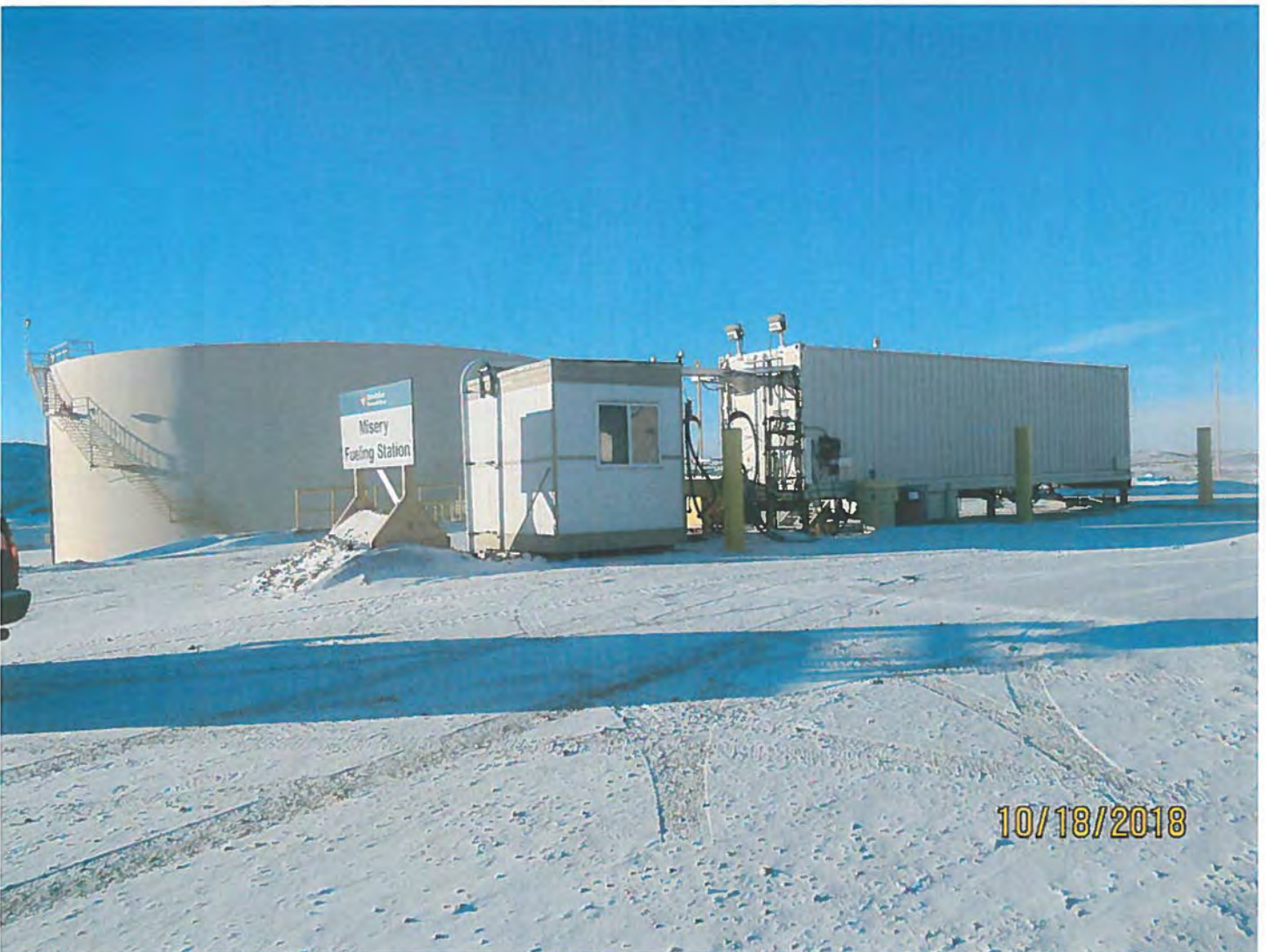
Photo #20 - W2017D0004 MUG Project Looking north at the Misery Camp fuel transfer station and bulk diesel tank.
