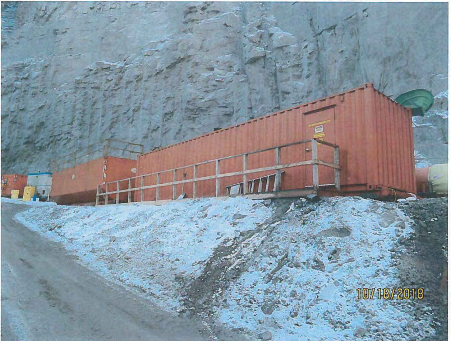
Photo #13 - W2017D0004 MUG Project The mud (left) & brine (right) tanks used for underground water management activities.
