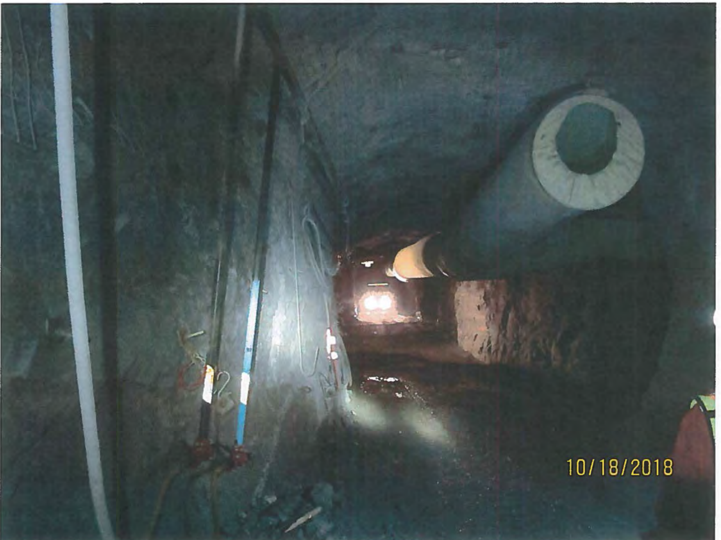
Photo #16 - W2017D0004 MUG Project The vent tubing carrying warm air into the mine and water lines on left used in the underground water management.
