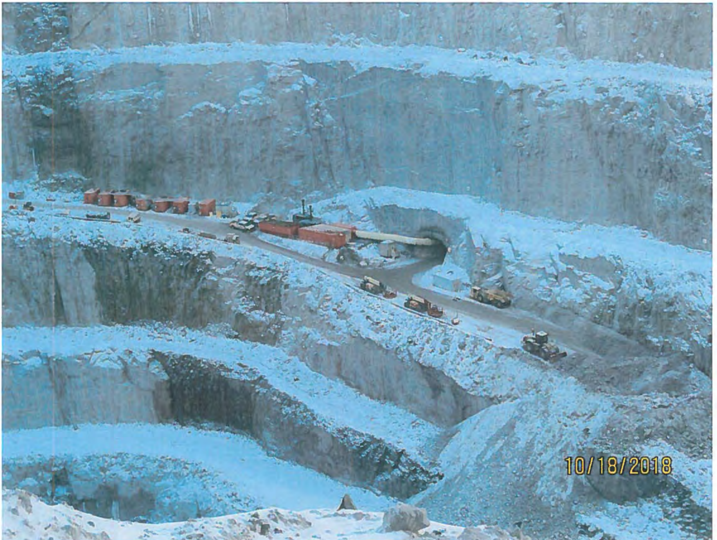
Photo #11 - W2017D0004 MUG Project Looking down at the 2235 Portal. A rock disposal area into Misery Pit can be seen in the bottom-right of the photo.
