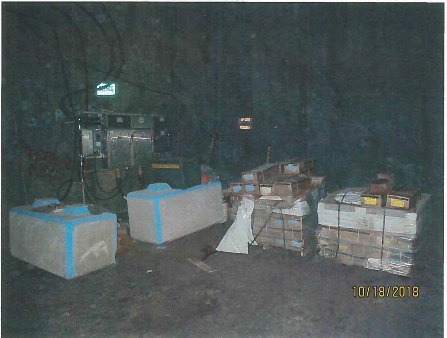
Photo #17 - W2017D0004 MUG Project An underground electrical conduit station and epoxy used to cement bolts into place.
