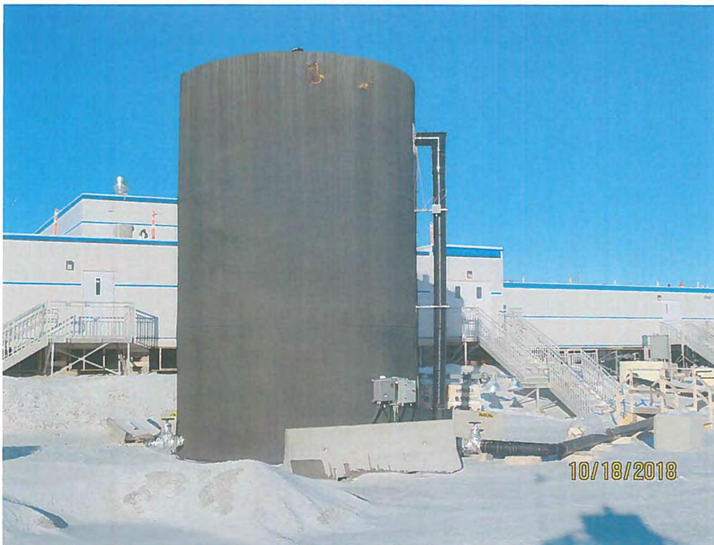
Photo #3 - W2017D0004 MUG Project This sewage holding tank is located west of the new accommodations buildings.
