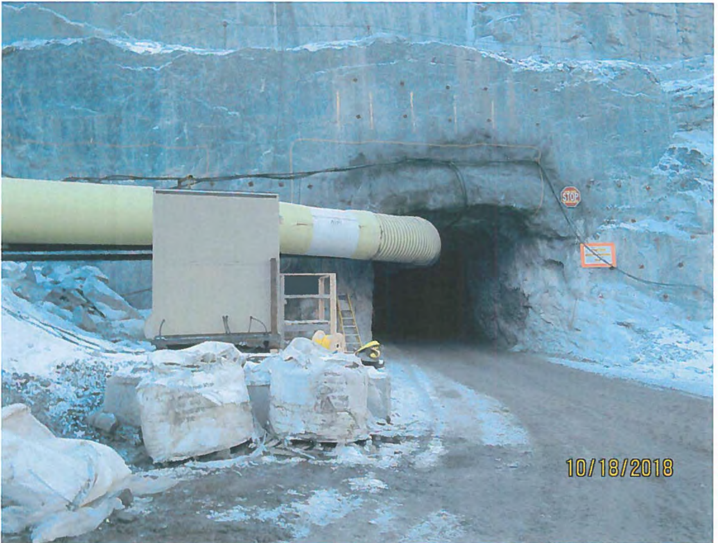
Photo #15 - W2017D0004 MUG Project The fresh air vent tubing going into the 2235 Portal and staged sodium chloride used in underground operations.
