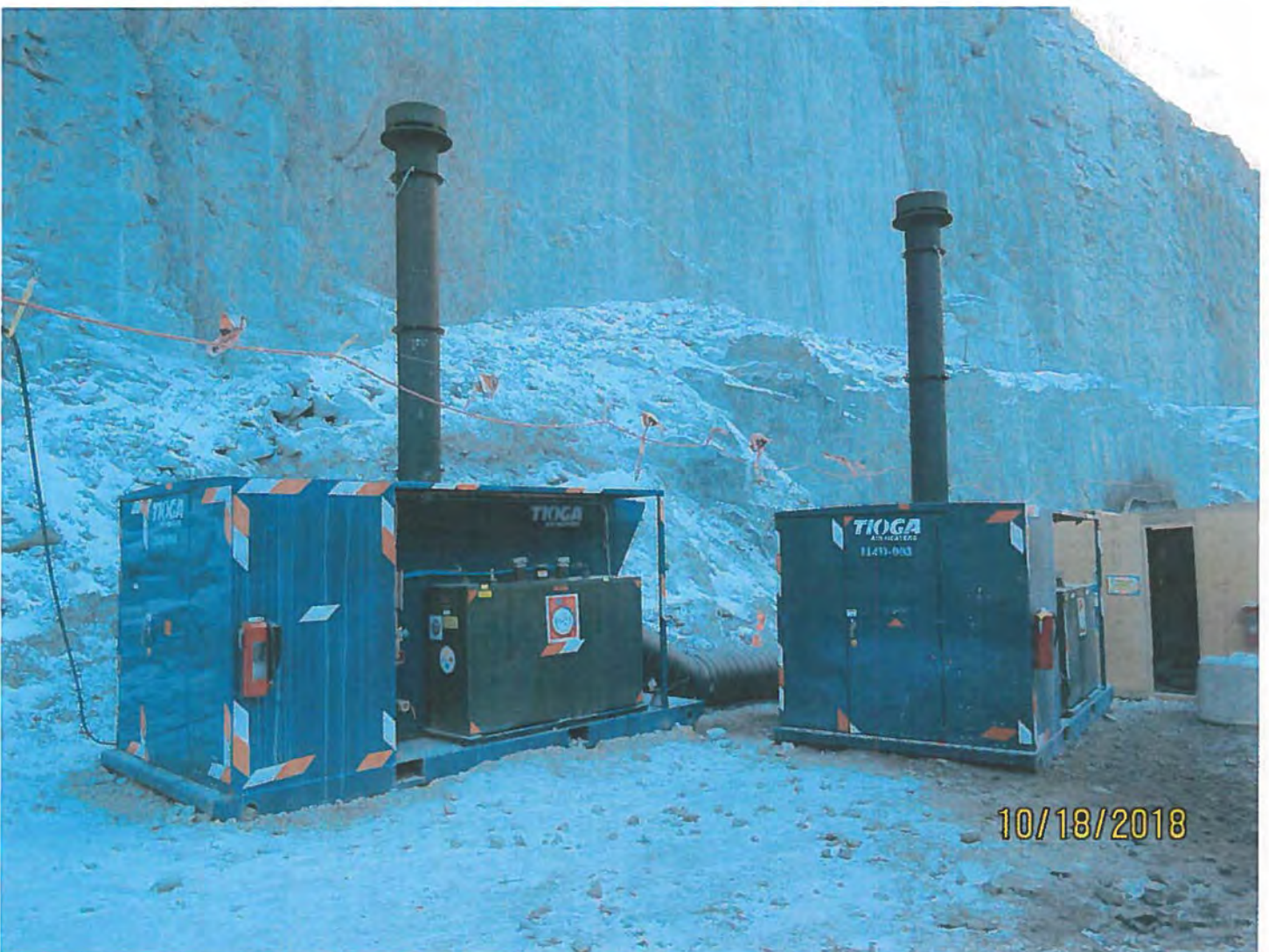
Photo #14 - W2017D0004 MUG Project These heaters are used to heat the air that is being pumped into the underground.
