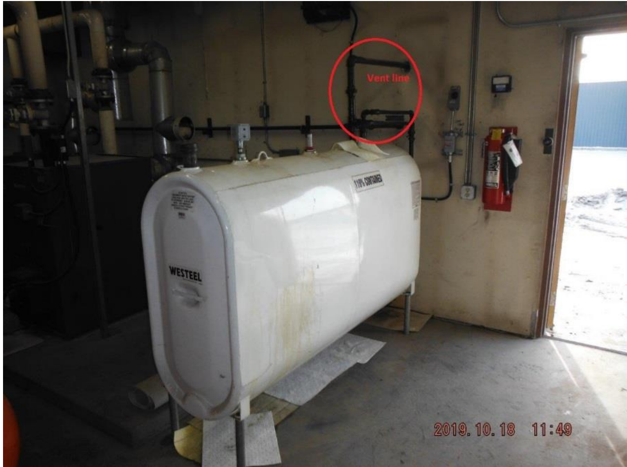
Figure 2. Day tank inside Misery Light Duty Shop
