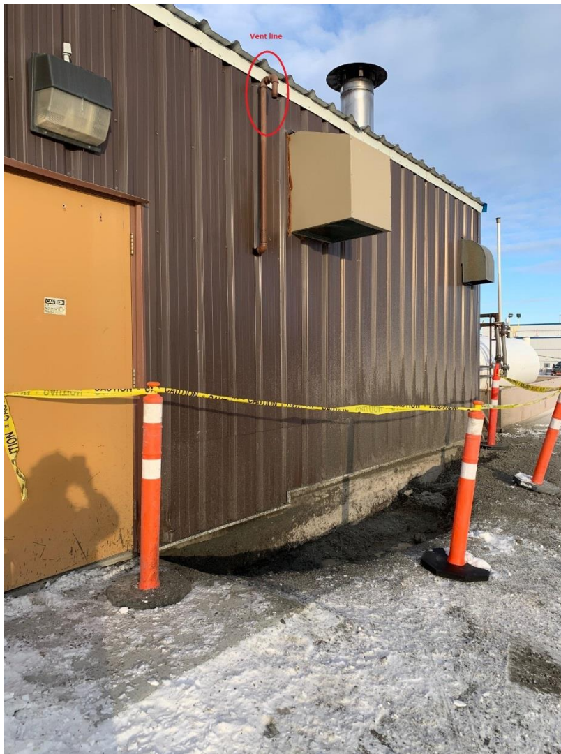
Figure 3. Vent line and spill excavation outside of Light Duty Shop
