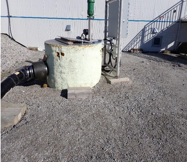
Photo 1: Misery Camp Lift Station – View of cleaned up spill site after enzymes application and evaporation.
