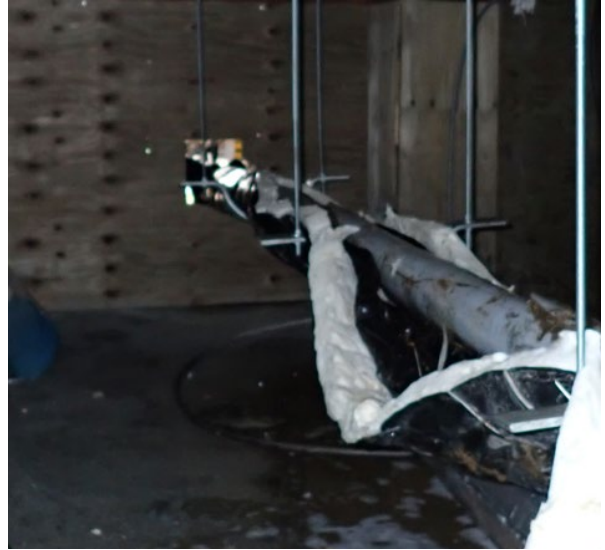
Photo 2: Men's Dry Area – View of spill area (14m 2 ) after clean-up. Fluid on ground is the bio-engineered enzyme cleaning solution.
