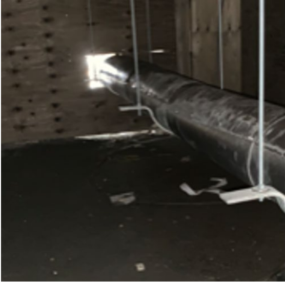
Photo 1: Men's Dry Area – View of sewage pipe after spill had occurred.
