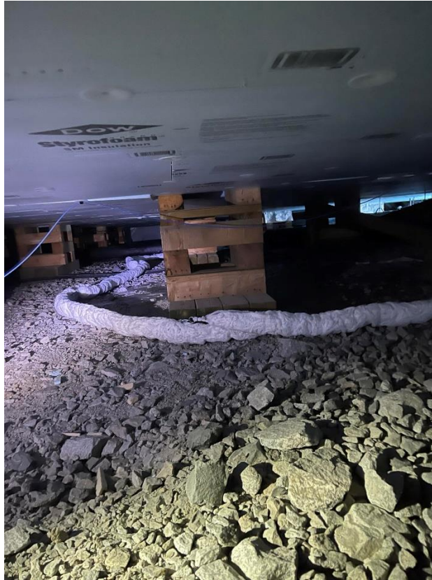
Photo 2: After photos of Spill-2024042 at Misery Camp.
