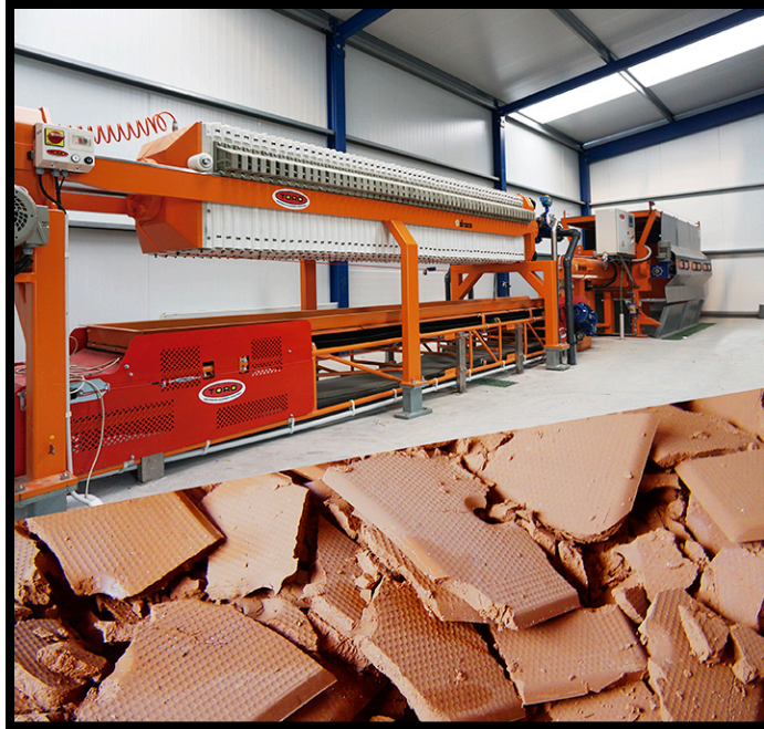
Figure 9. Solid wastes dewatering by a plate filter press (Toro Equipment, 2015)
