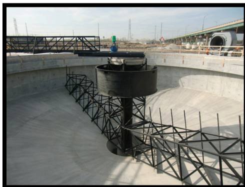
Figure 3. Circular gravity thickening tank equipped with scrapers (GSPS Engineering, 2017)
