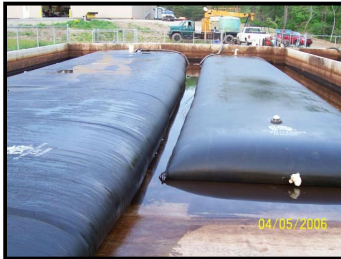
Figure 12. Geotubes for SFBW Treatment at Ohio WTP (Mastin et al., 2008).
