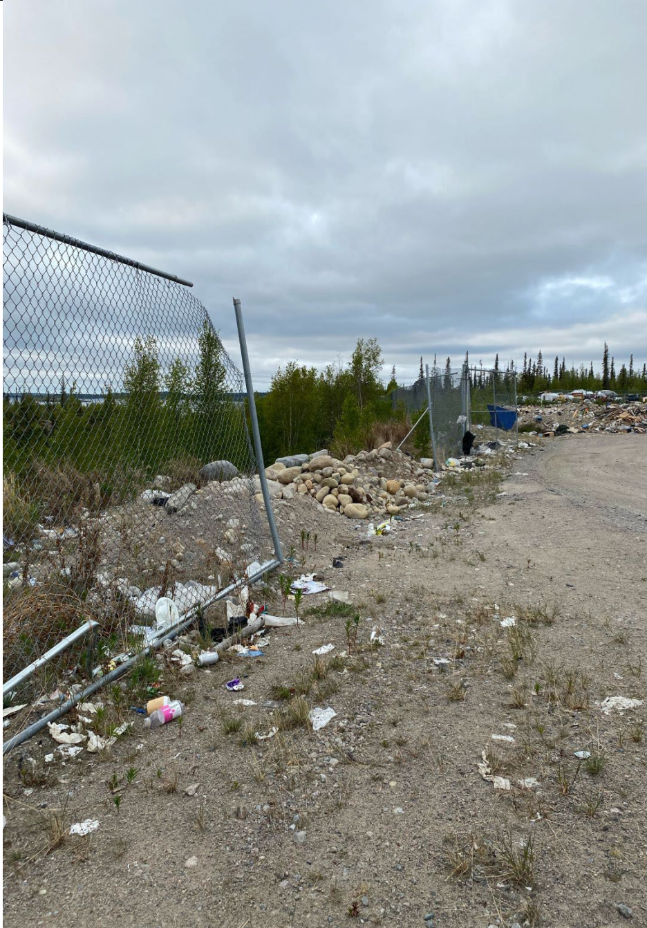
Solid waste facility fencing in need of repair
