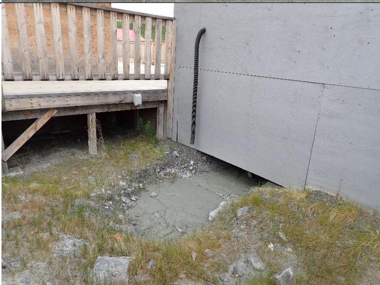
Photo #4: Grey water sump from core cutting building
