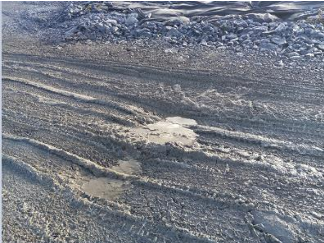
Area Requiring Repair
