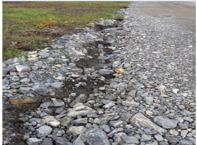
Damaged/Sliding Area of Road
