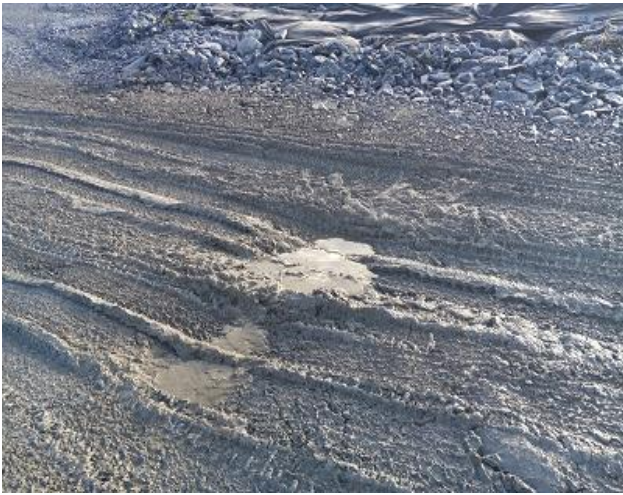
Area Requiring Repair
