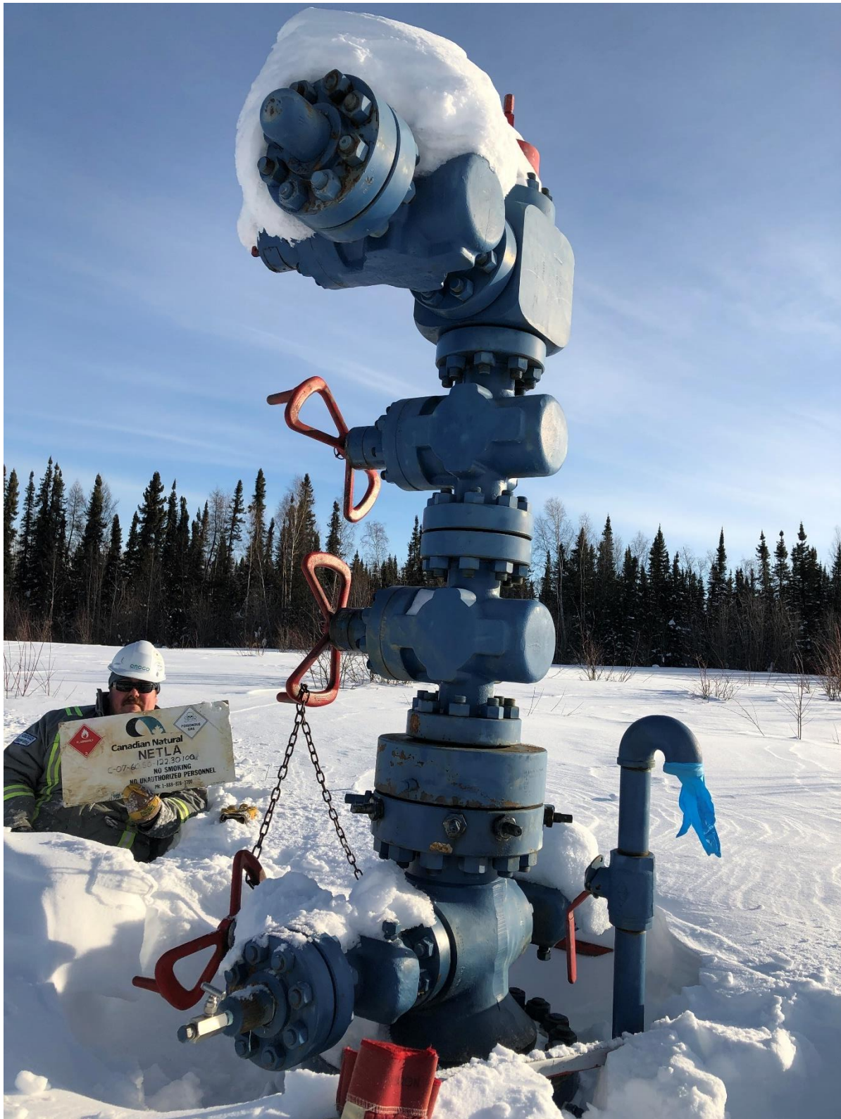
Photo #3: Netla C-07 - Well head identification sign not secured - Surface casing vent glove test
