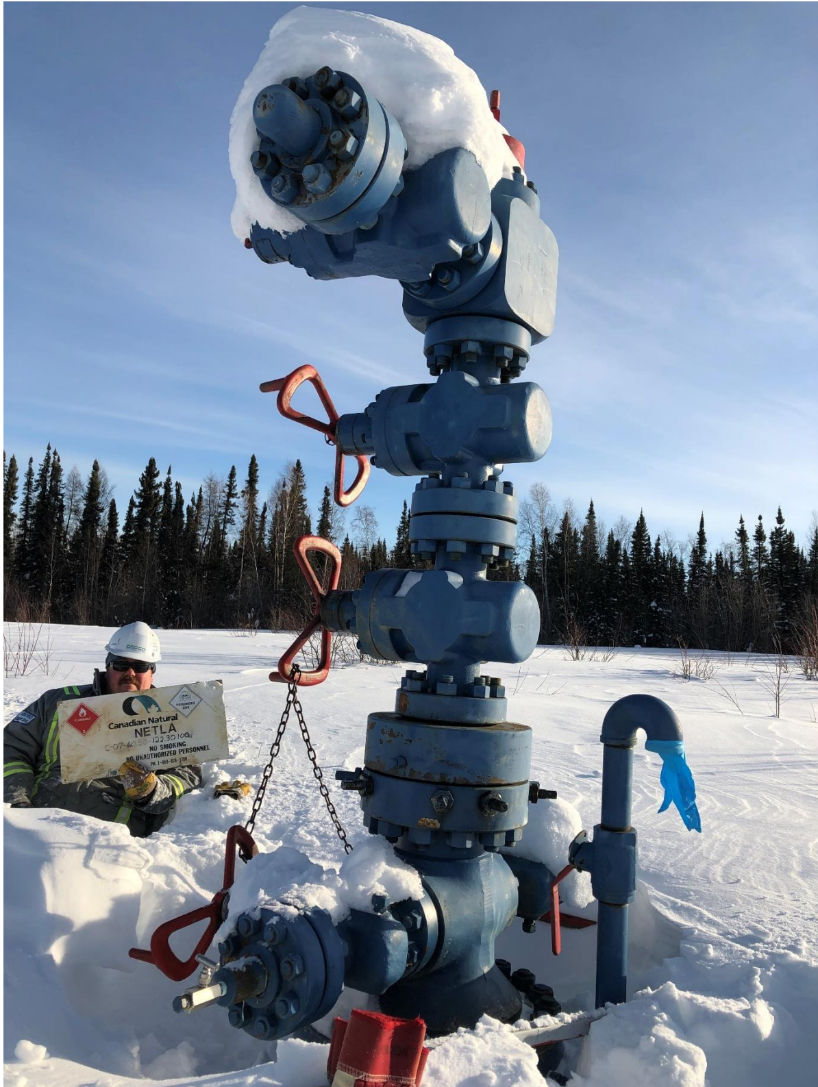
Photo #3: Netla C-07 - Well head identification sign not secured - Surface casing vent glove test
