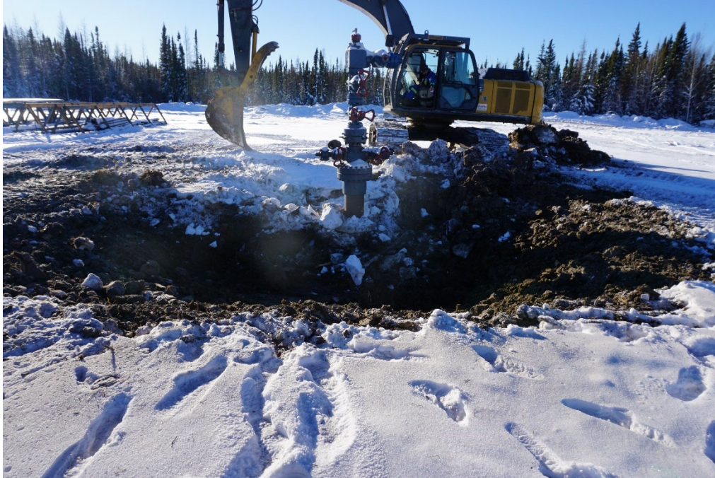
PHOTO #1: View of the C-07 wellhead being exposed for cut and cap operations.
