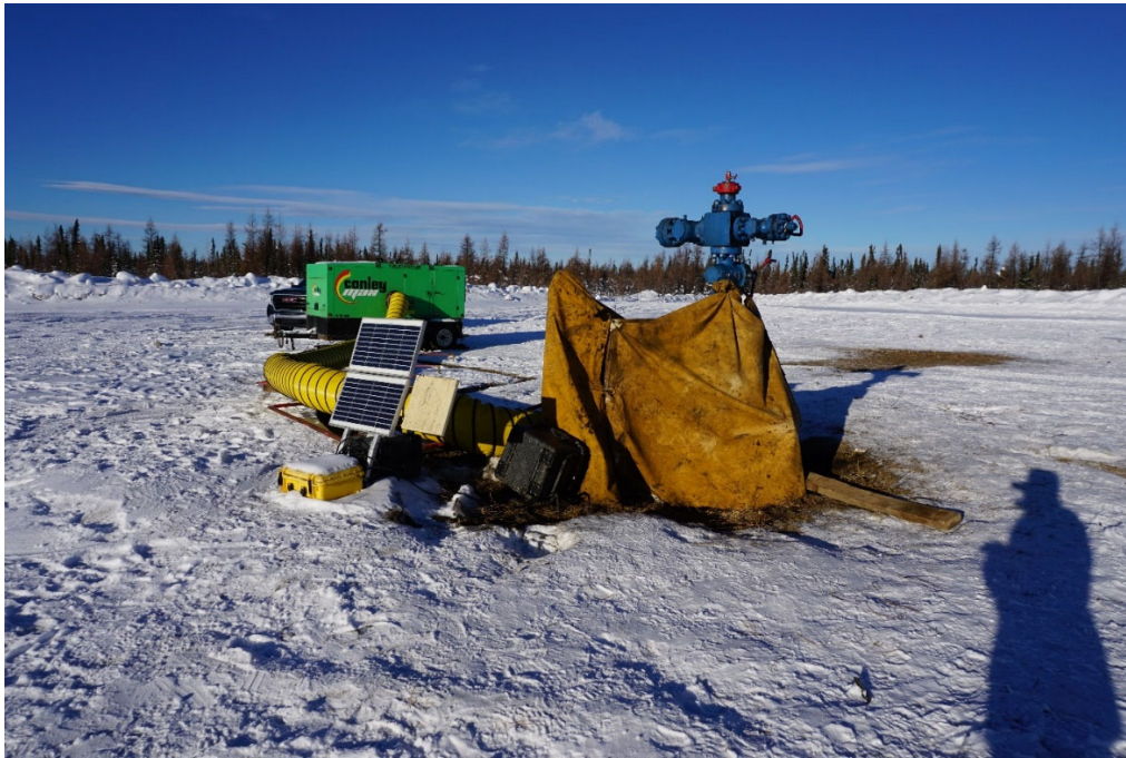
PHOTO #1: View of the A-77 wellhead monitoring for surface casing vent flow after completing the casing expansion intervals.
