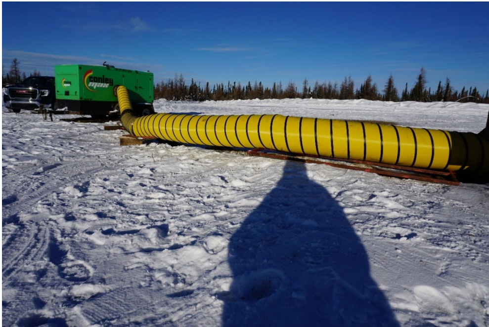
PHOTO #3: Heated air tubing was elevated off the ground surface and no concerns were noted.
