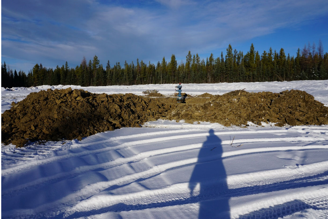
PHOTO #1: View of the I-75 wellhead being exposed for cut and cap operations.
