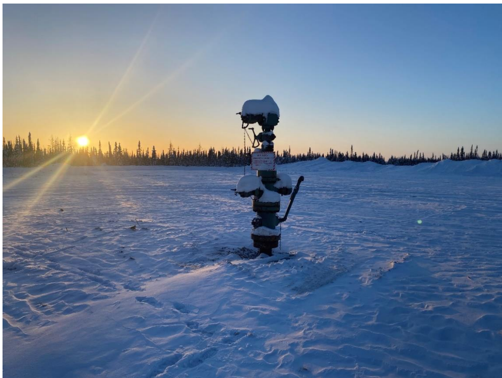
Photo 2: Nogha K-14 (WID 2006) Wellhead with valves chained and well identification signage in place.
