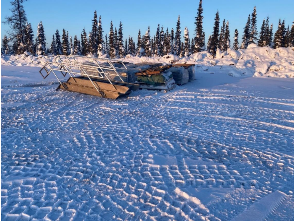
Photo 1: Pallets of G class cement and metal stairs on site to support abandonment operations.
