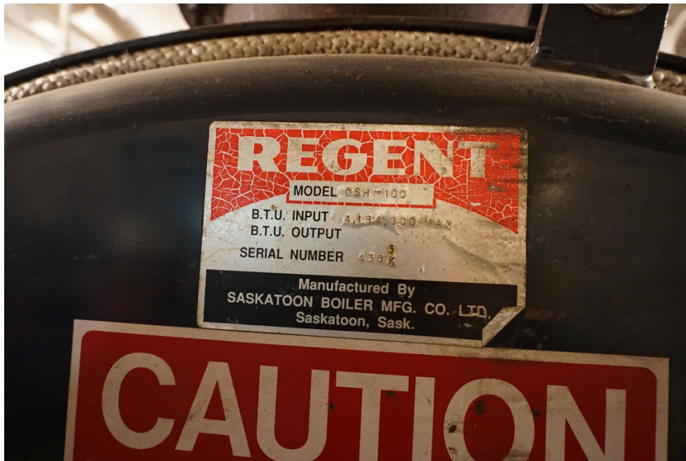
PHOTO #3: View of the Boiler with Serial number 4363.
