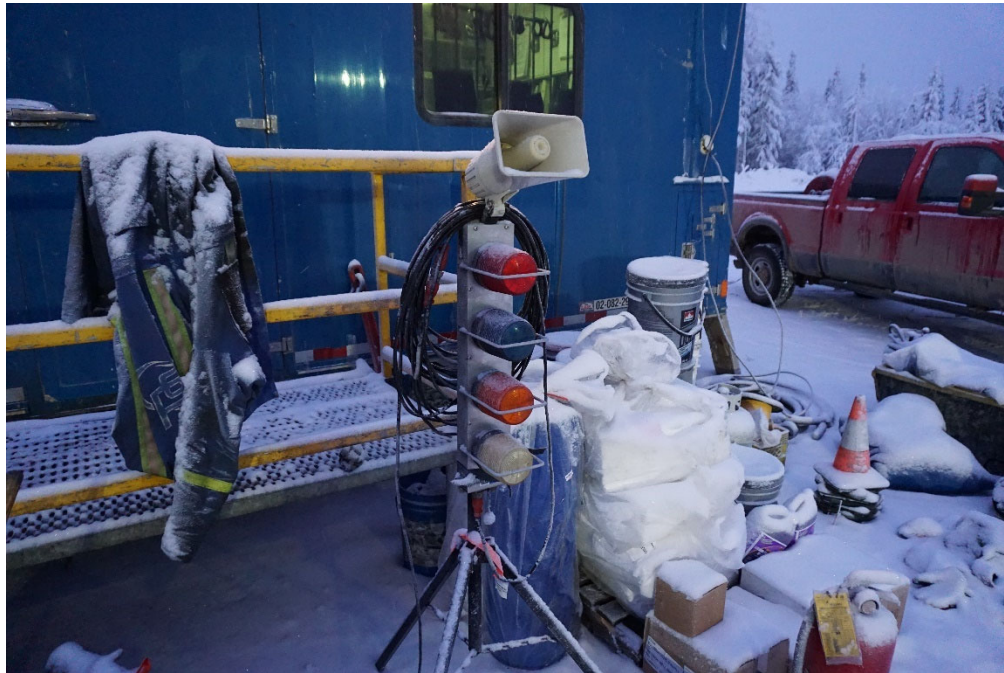
PHOTO #9: H 2 S sensors sound an alarm and lights illuminate indicating where the hazard is present.
