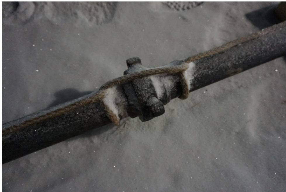
PHOTO #4: Pressurized line from the P-tank to the Flare stack was secured with continuous anchor line on either side of the segment coupling.
