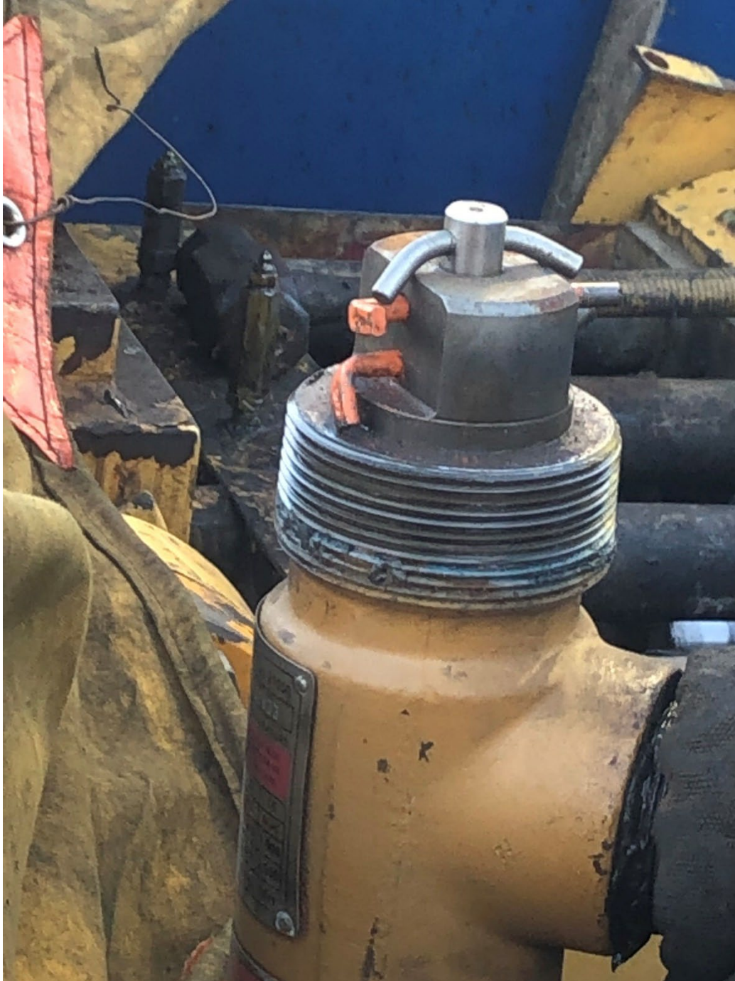
Photo #7: Rig Tank Pump with OTECO Pressure Relief Valve set with 2 orange shear pins = 34.4 MPa.
