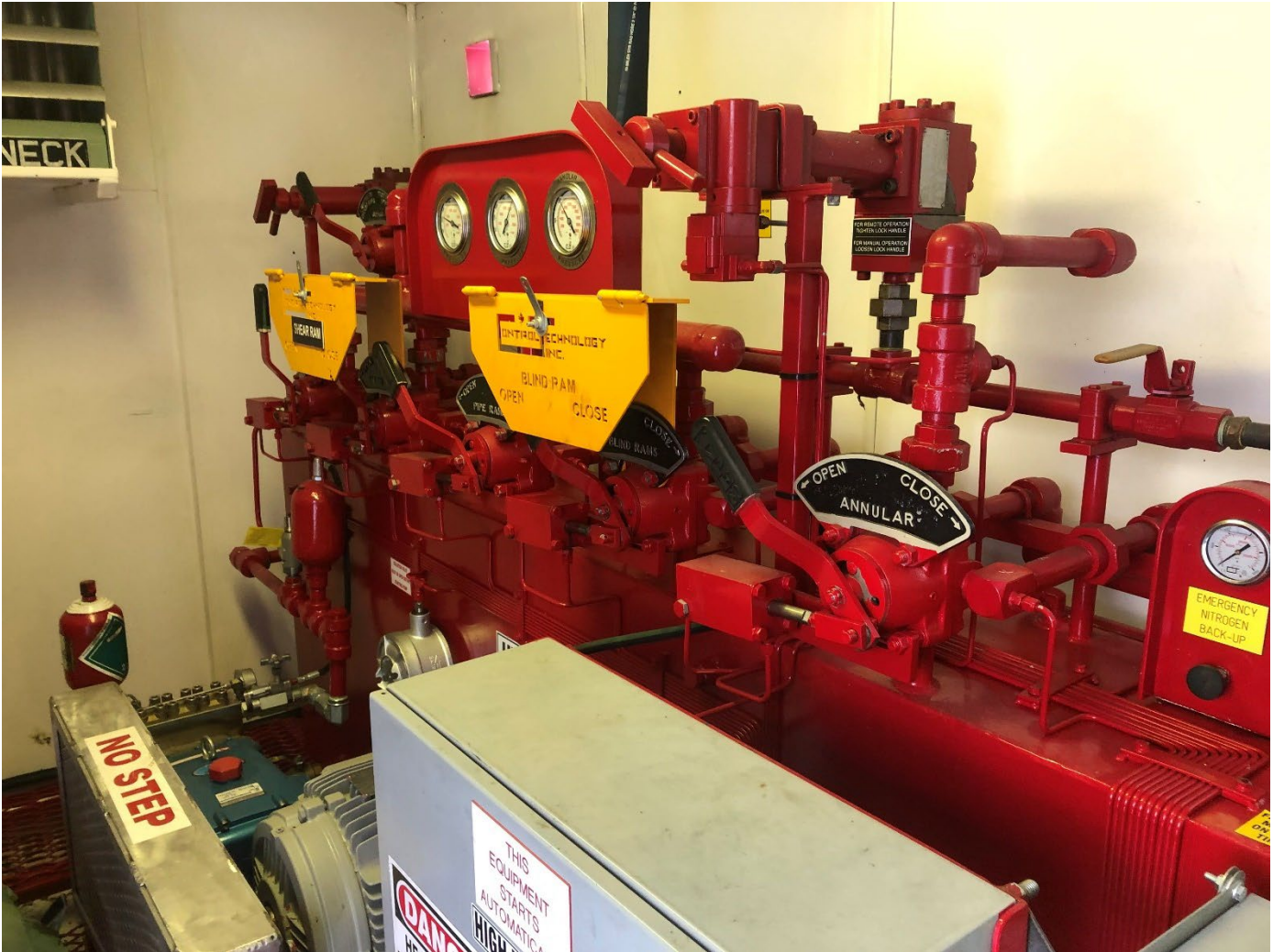
Photo # 2: Accumulator post January 25, 2022 function test.
