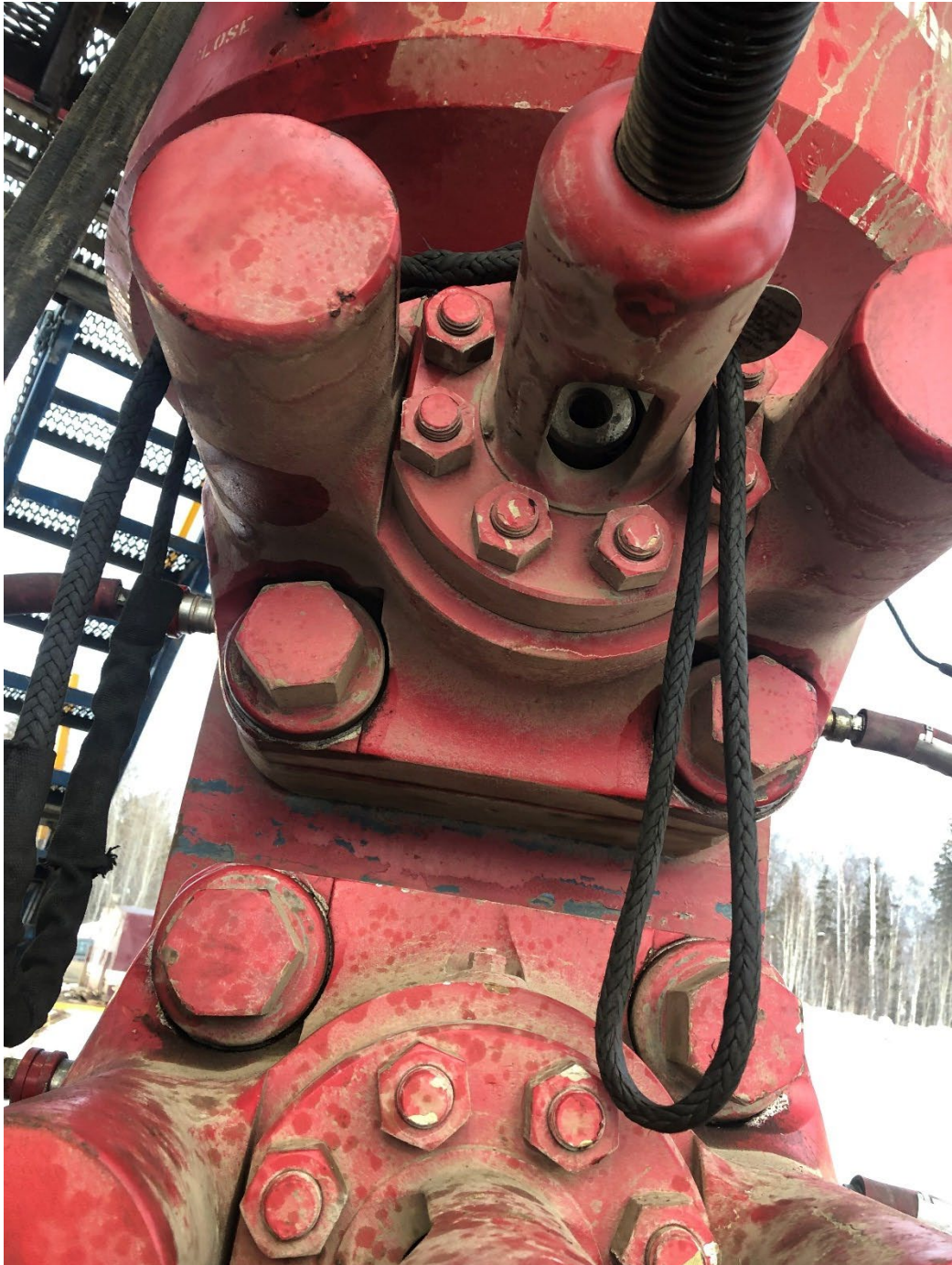
Photo #3: Verification blind ram closed during January 25, 2022 function test.
