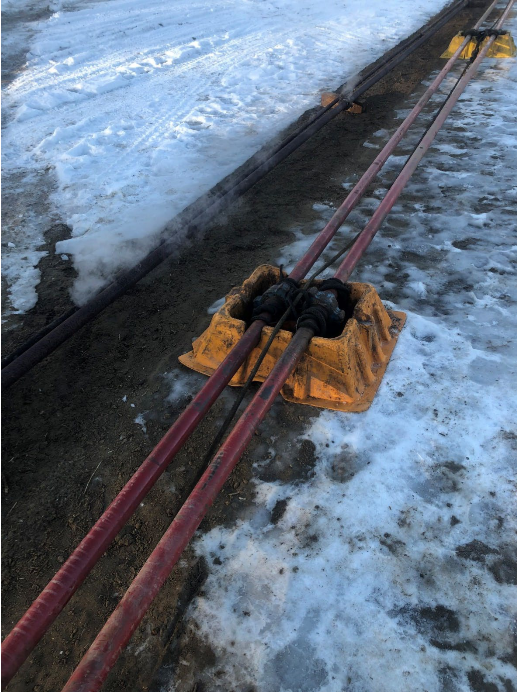
Photo #5: Flow lines to the rig tank raised from the ground and Anchored at each connection with one continuous high tensile strength line.
