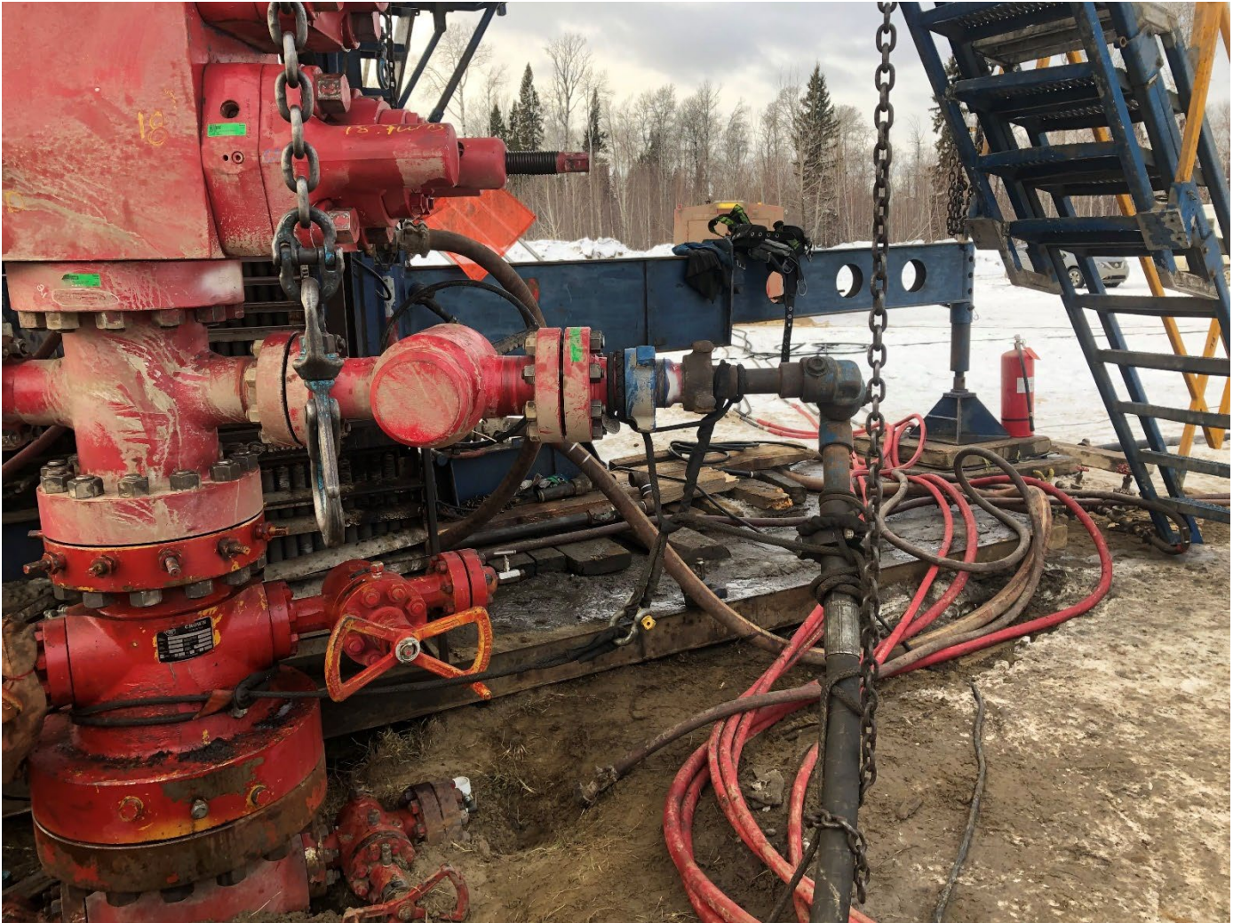
Photo #6: BOP Stack with fire retardant kelly hoses which were confirmed to extend > 7m from the well centre.
