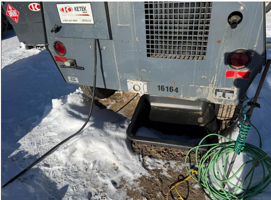
Photo 28: Drip tray under generator
