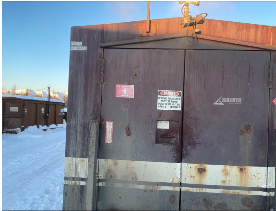
Photo 11: Boiler PWS 710 (in service)
