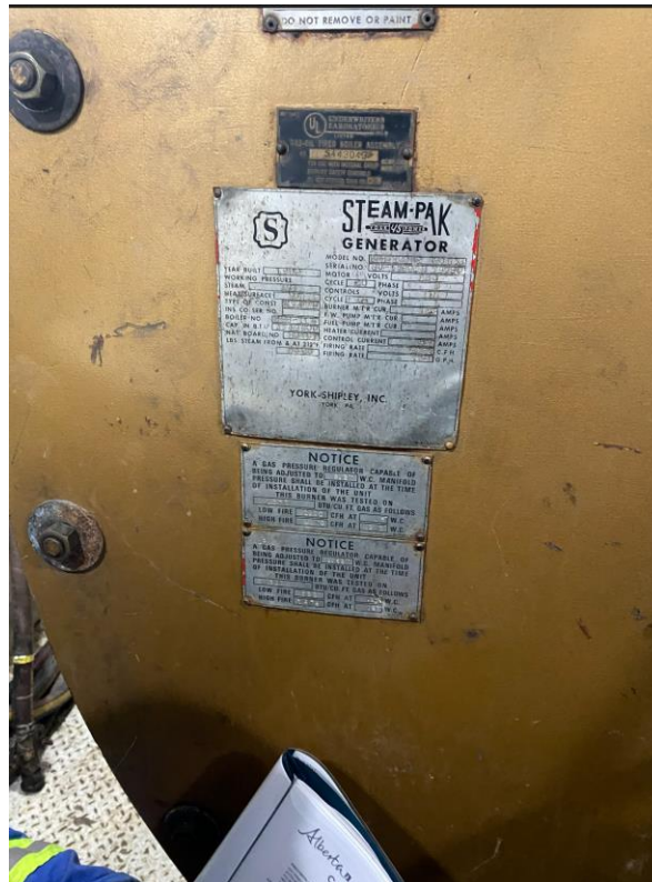
Photo 10: Boiler PWS 757 boiler information placard
