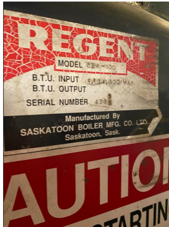
Photo 13: Boiler PWS 710 boiler information placard
