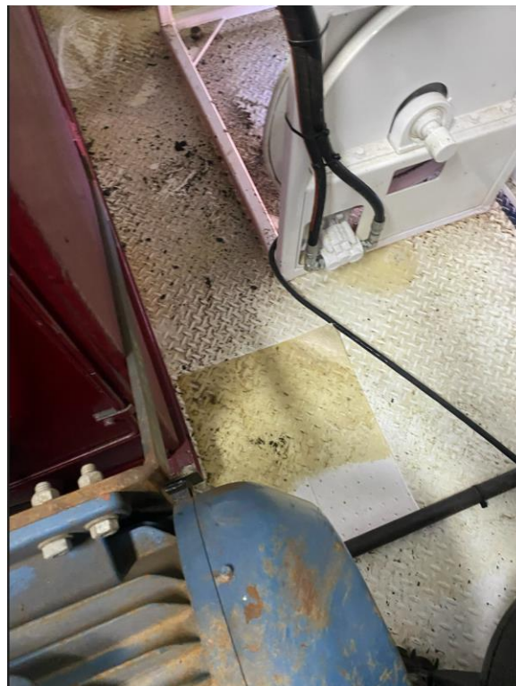
Photo 16: Leak below swivel joints in accumulator container
