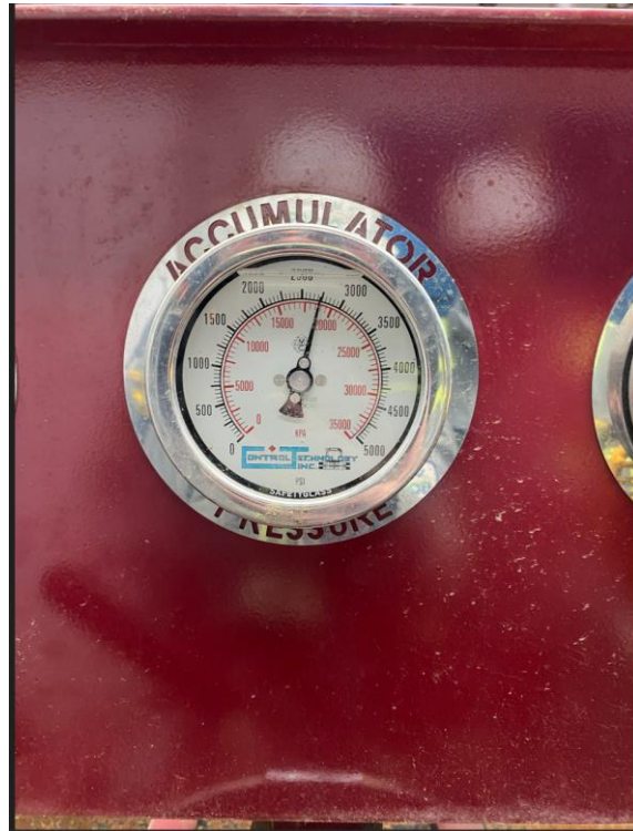
Photo 1: Accumulator at 19,000 kPa prior to 3 function test
