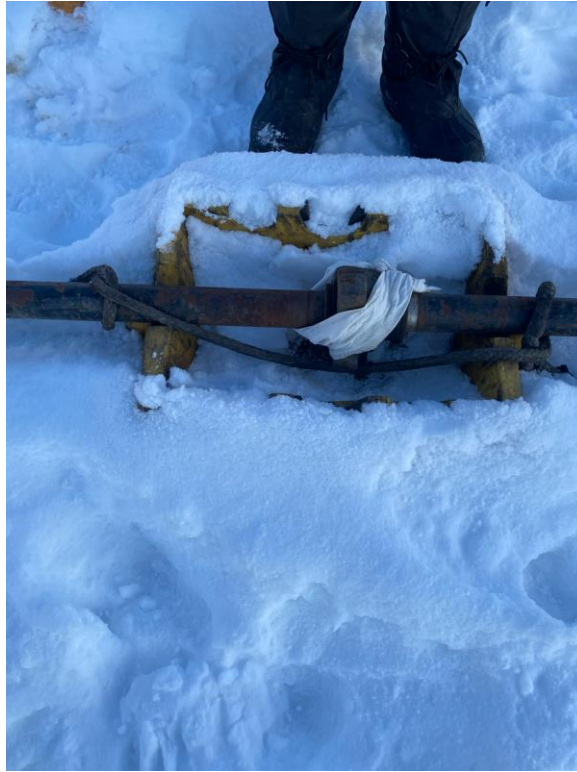
Photo 19: Flow lines from the well centre to the manifold with anchored joints
