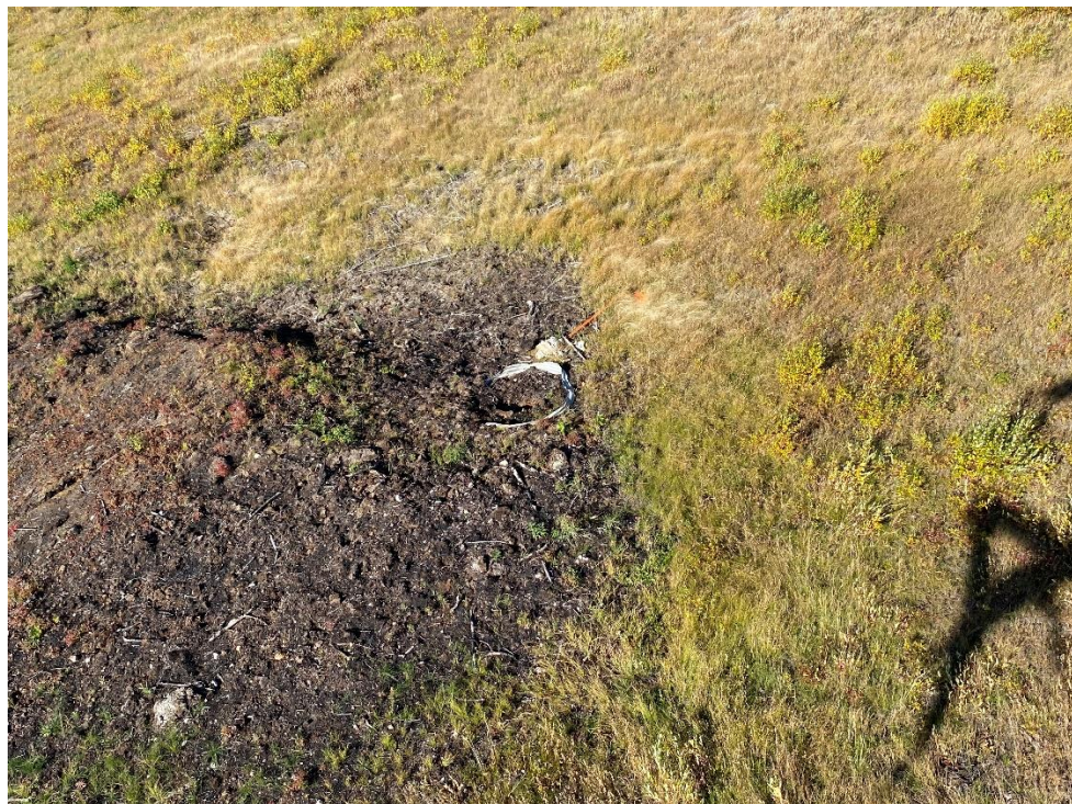
Photo 2: Cameron A-68 (WID1746) – Open excavation at well center, cellar still in place and improperly installed well abandonment sign.
