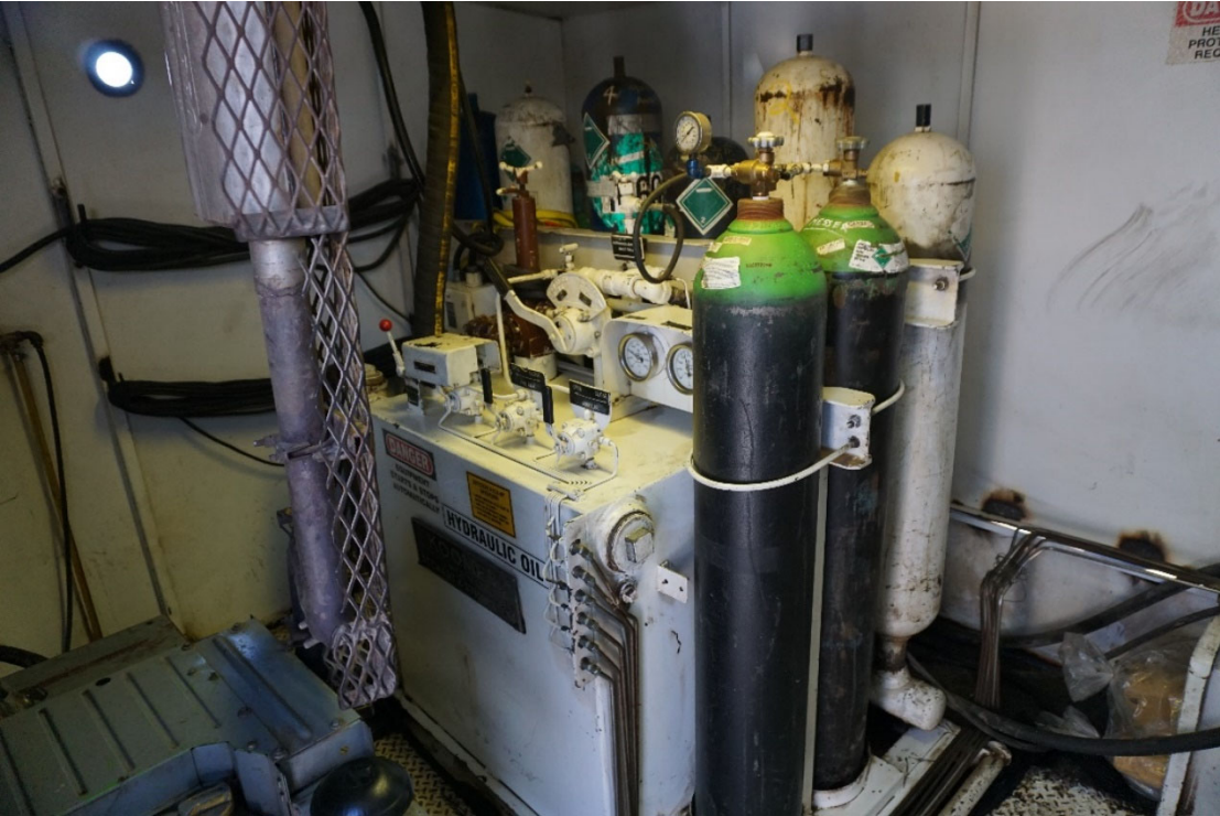
PHOTO #1: Accumulator shack and nitrogen bottles located adjacent to the Doghouse.
