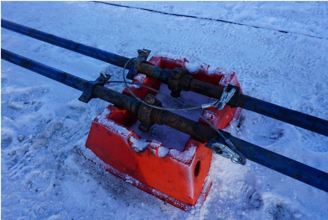
PHOTO #7: Pump lines were secured with heavy gauge cable and no concerns were noted.
