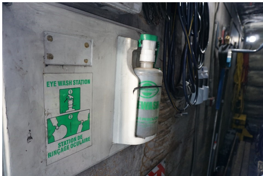
PHOTO #10: The white aerosol style eye wash equipment in the background was expired and must be replaced prior to the next scheduled inspection.
