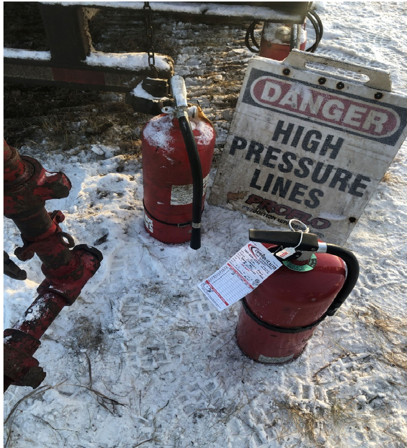
PHOTO #9: Verified fire extinguishers were brought to site for replacement at the Pressure tank.
