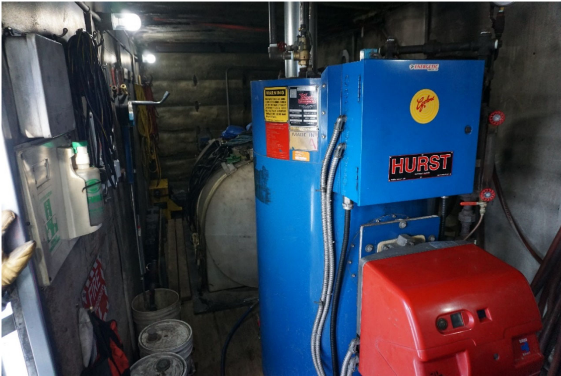
PHOTO #4: Inside view of the boiler and water tank.
