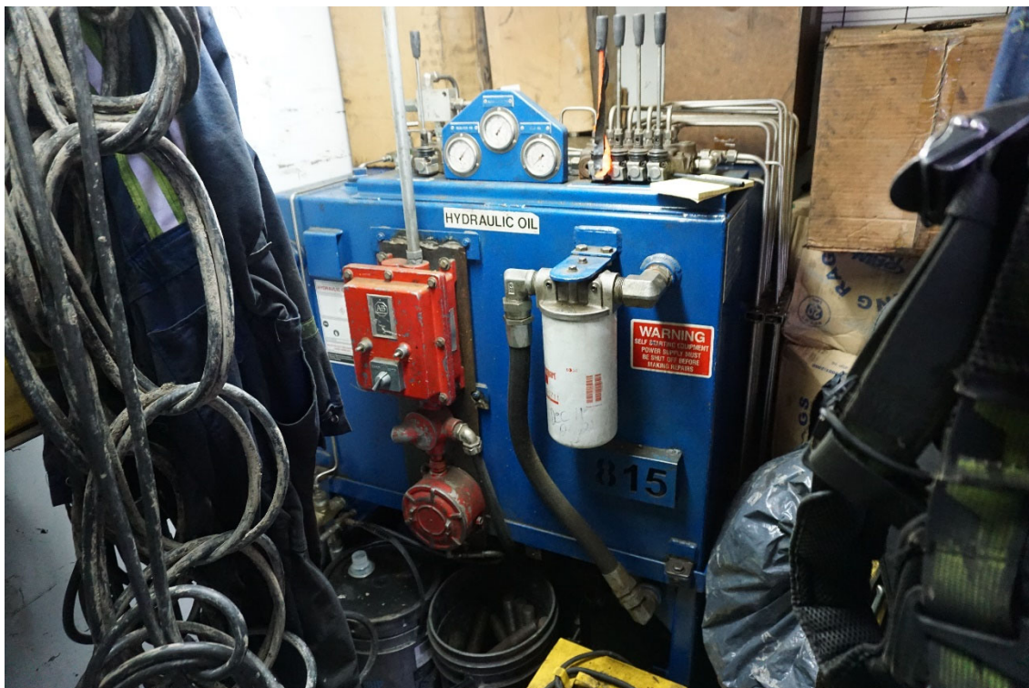
Photo #1: Accumulator repressurized after function test.
