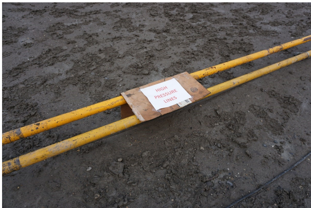
Photo #9: Temporary hazard signage was placed on pump lines after wildlife in the area misplaced them. No concerns were noted since signage was still made visible to all workers on site.
