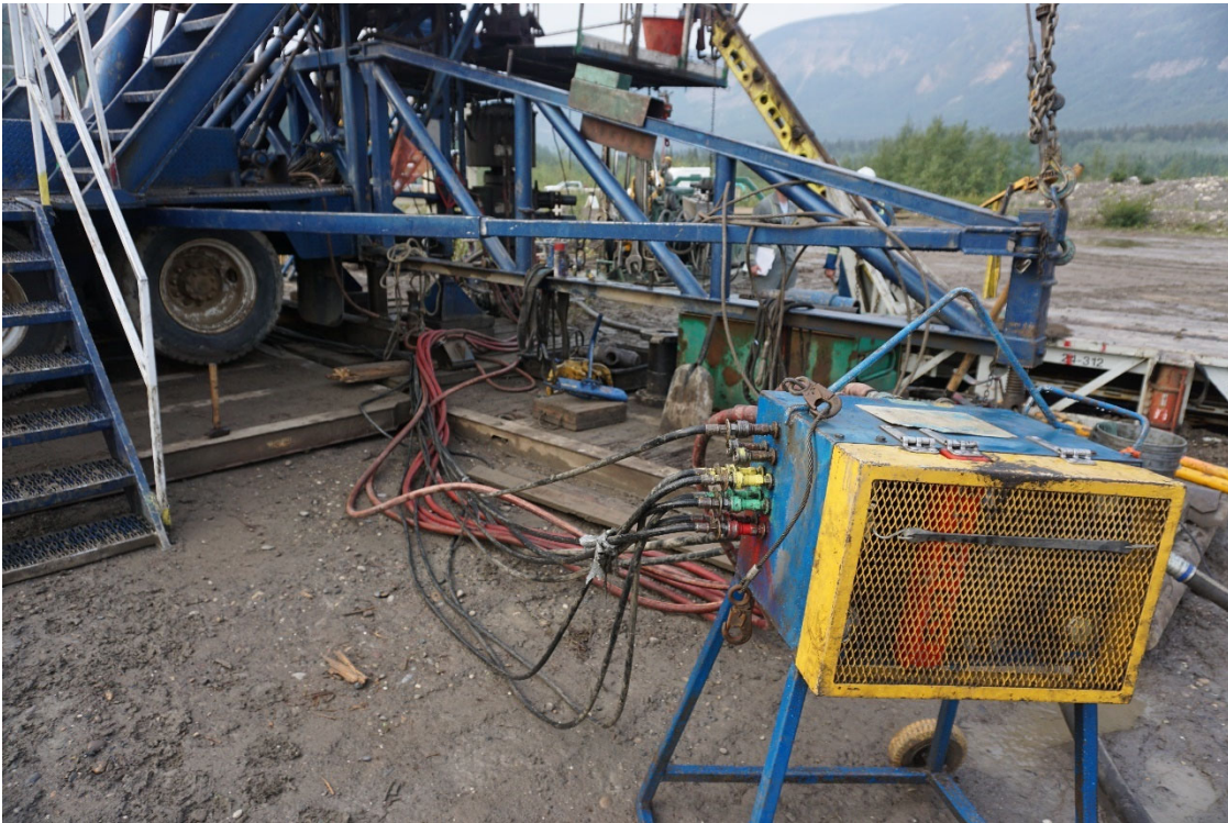
Photo #4: Fire rated Kelly hoses were greater than 7 meters from the BOP stack.
