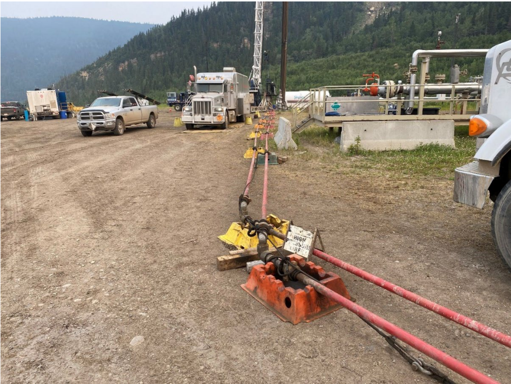
Photo #9: High Pressure Lines sign posted
