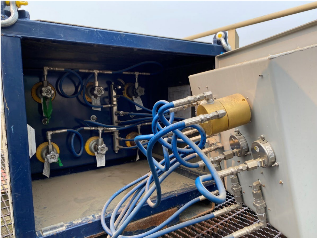
Photo #8: Supplied Air 6 tank system
