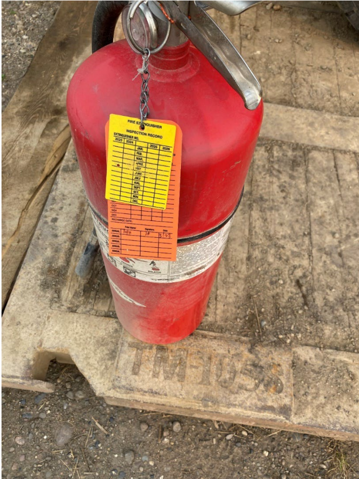
Photo #5: Fire extinguisher last inspected May 2023
