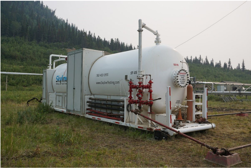
Photo #7: Flow turns were present and installed correctly.
