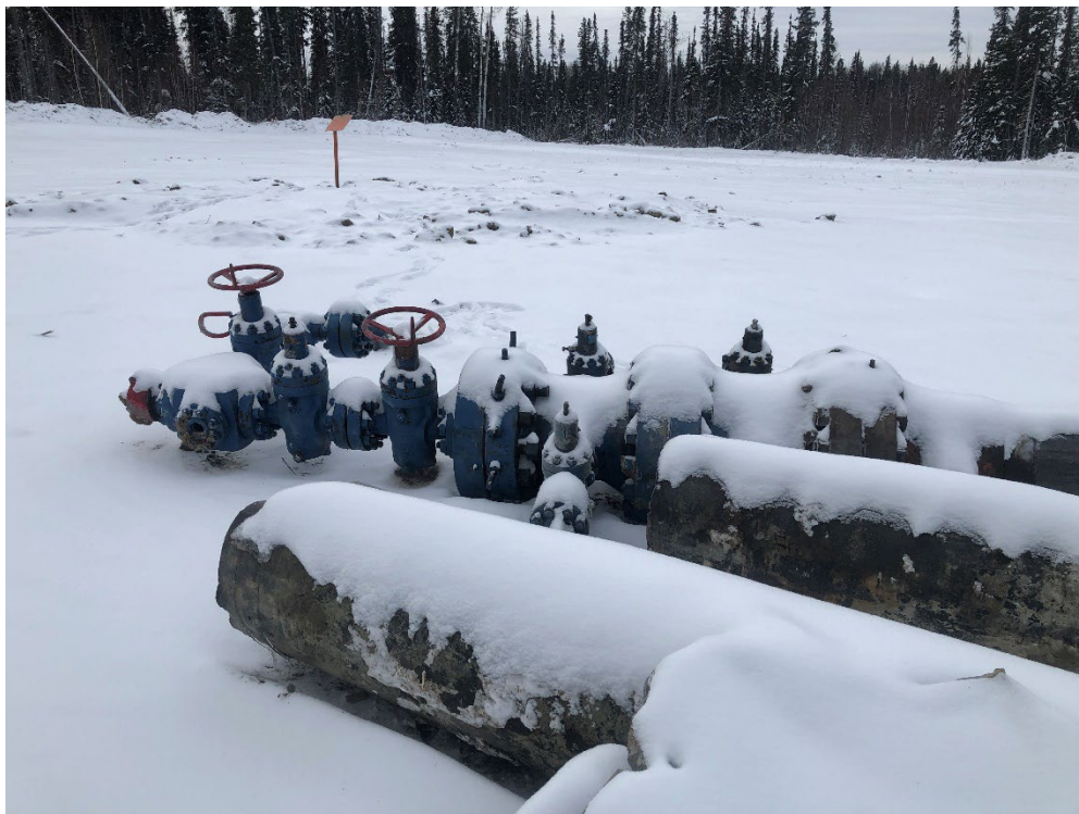
PHOTO #2: Wellhead and scrap casing requiring removal.
