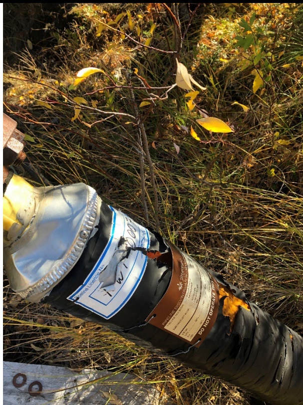
Photo #6: F-73/2F-73 inlet to gathering system. Tagged 'Do Not Operate'
