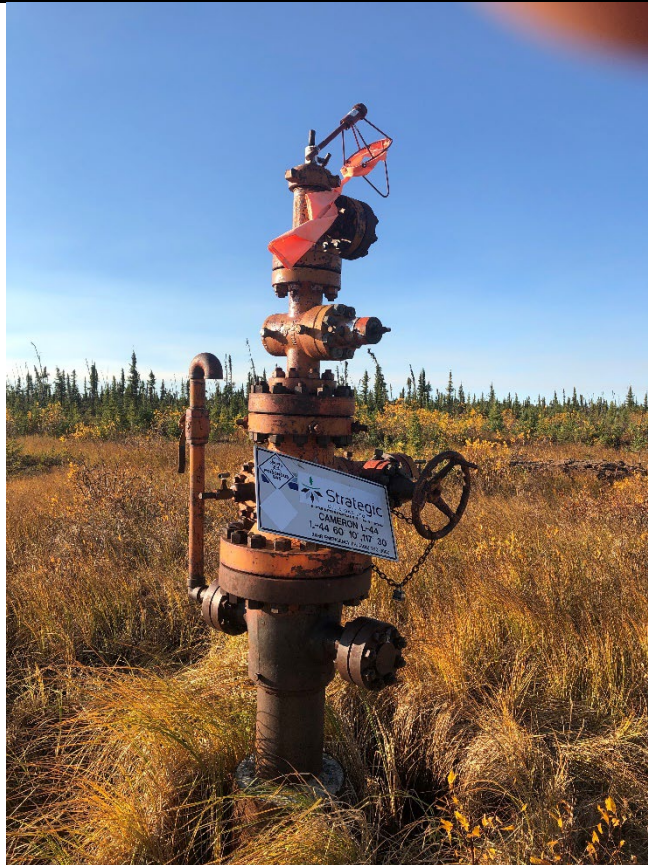
Photo #2: Cameron L-44 wellhead
