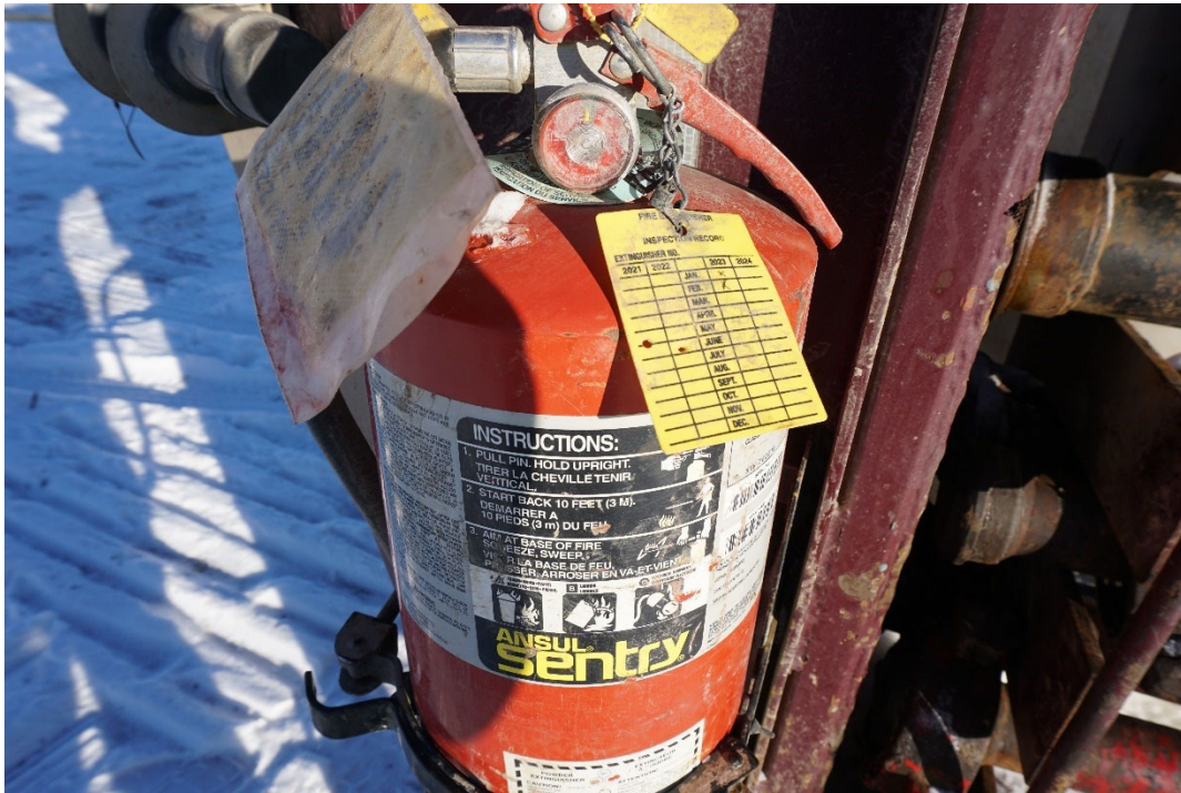
PHOTO #5: Fire extinguishers have been recertified within the last 12 months.
