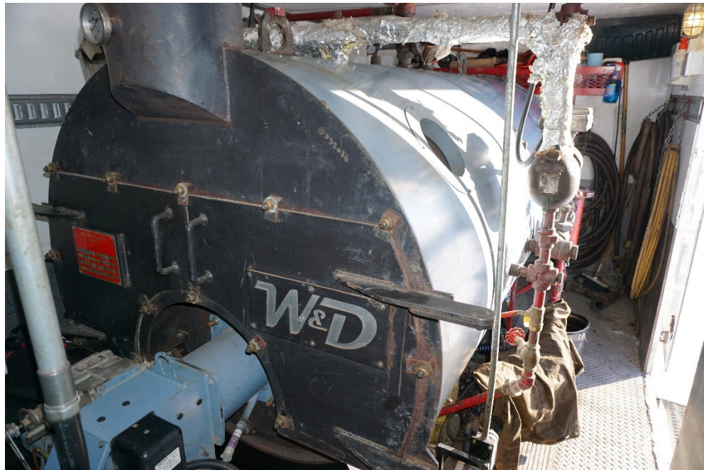
PHOTO #2: Another view of the boiler inside.
