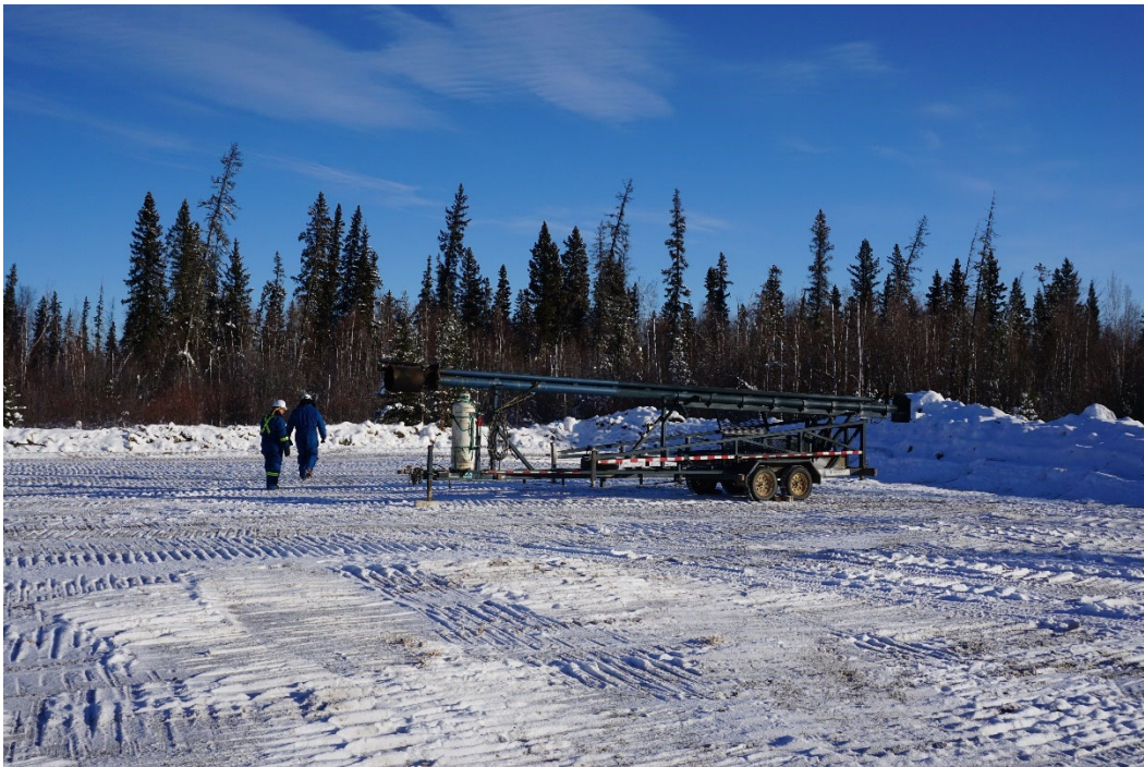
PHOTO #6: Flare stack was being re-positioned to an area that was at least 50 meters from the well center.
