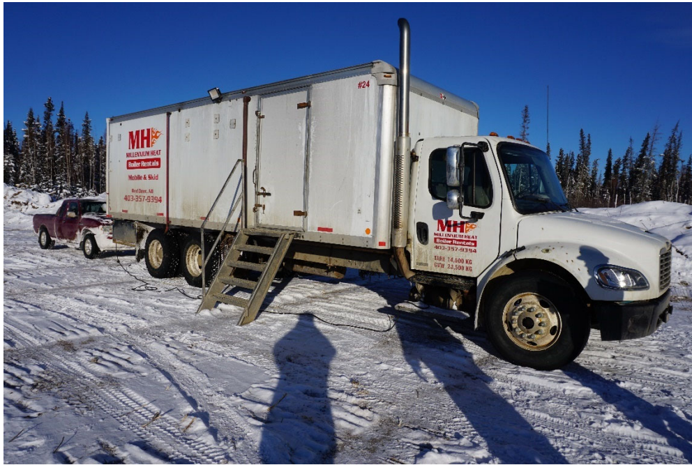
PHOTO #1: View of the Boiler.
