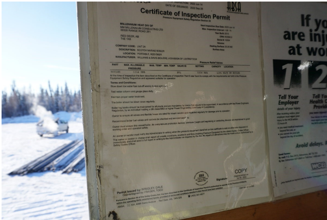
PHOTO #4: View of the Boiler Certifications hung up on the wall inside.
