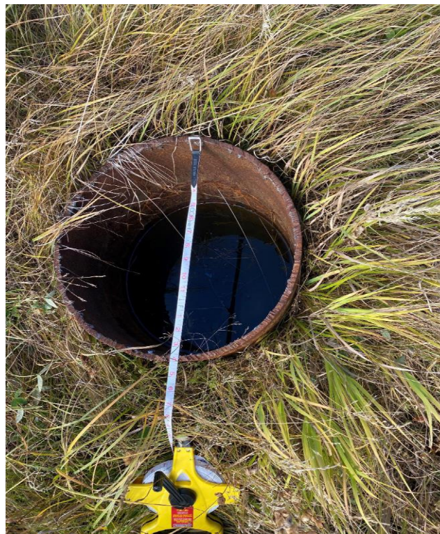
Photo 2: Cameron 2H-03 (WID2073) – 18" Unsecured piling
