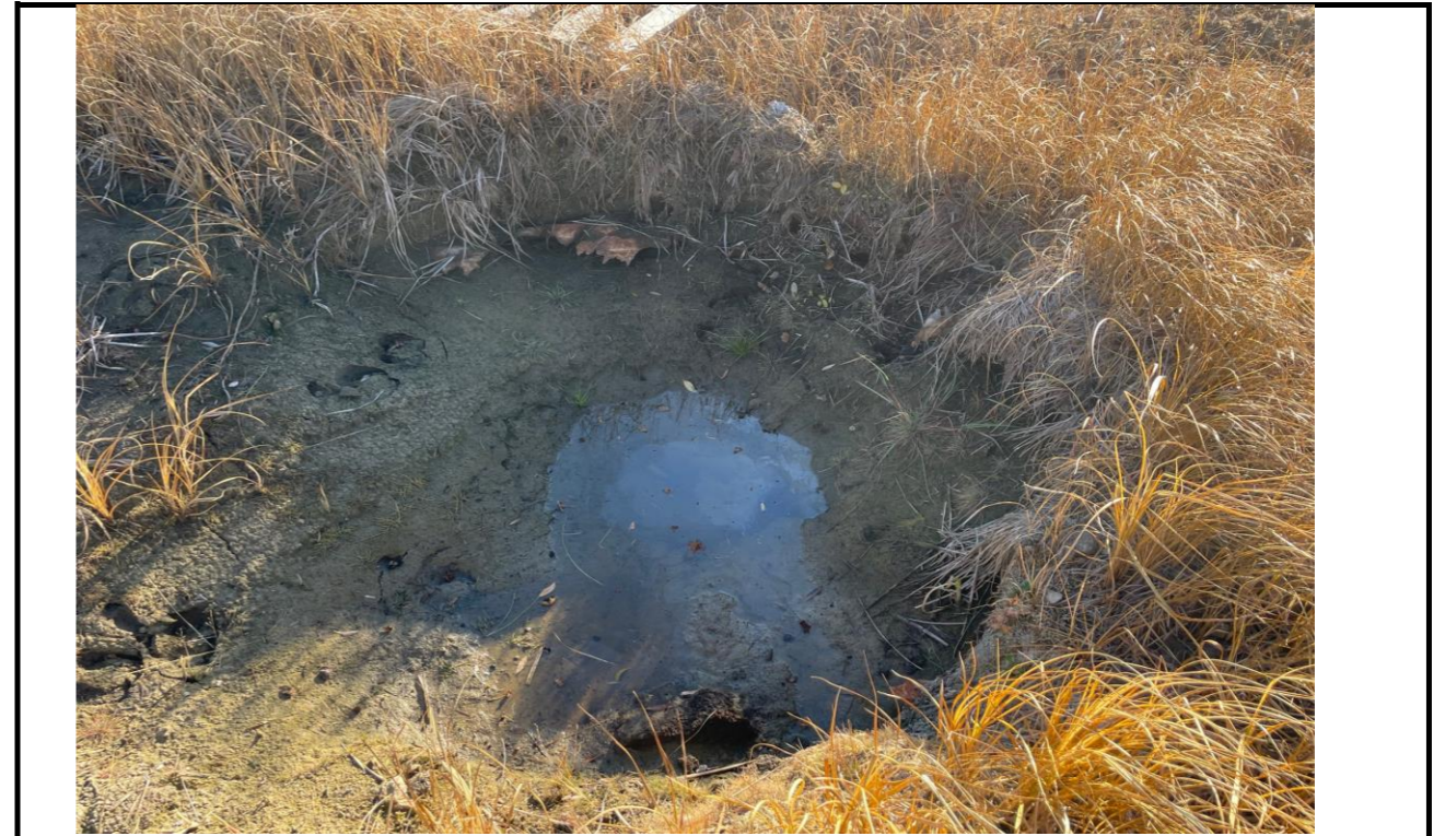
Subsidence at well centre
