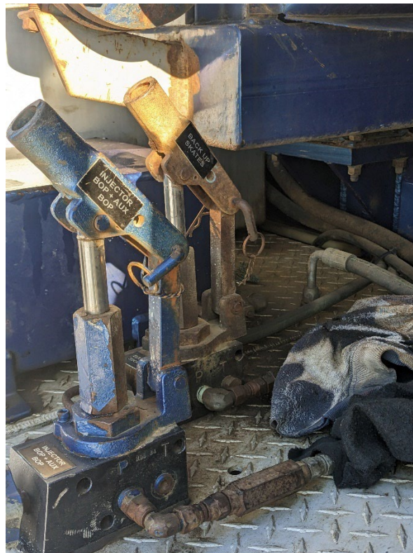
PHOTO #12: Manual pumps to pressurize Coiled Tubing Unit BOP.
