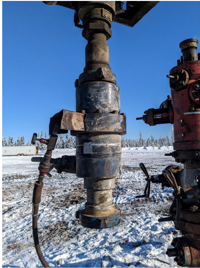
PHOTO #3: Coiled tubing annular disconnected after down hole abandonment operations were complete.
