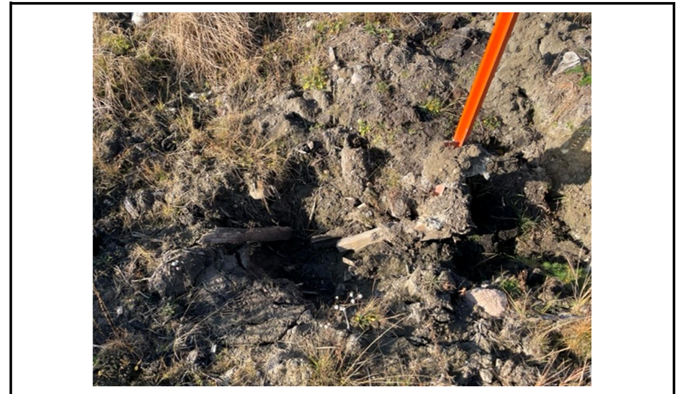
Subsidence at well centre from cut and cap
