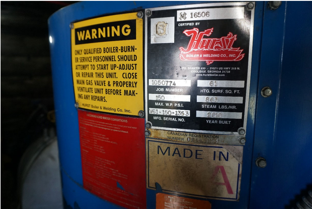
PHOTO #6: Boiler S/N# V61-15-1353.
