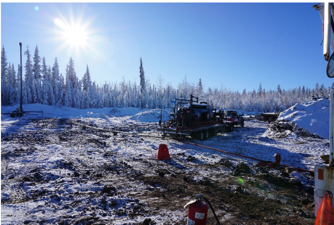
PHOTO #13: P tank and flare stack both hooked up prior to the end of the inspection.
