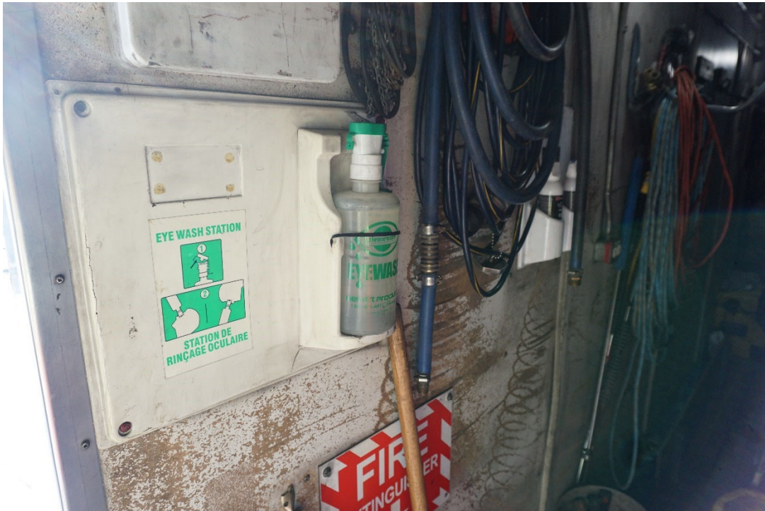
PHOTO #10: Eye wash station in the boiler has been replaced since the previous inspection.
