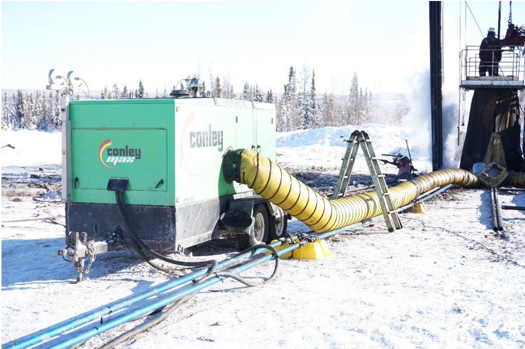
PHOTO #7: Lines were elevated to prevent thawing of the underlying ground and no concerns were noted.
